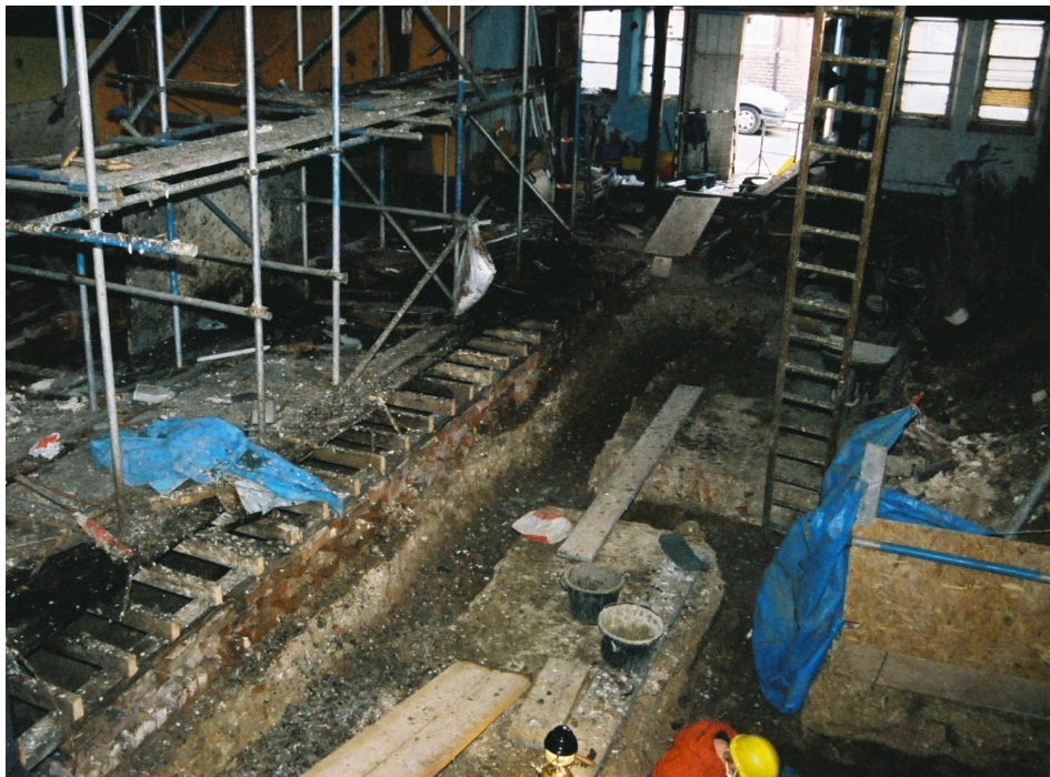
Fig 4 – the hand excavated trenches within the church in progress showing the difficult working conditions within the nave of the former church
