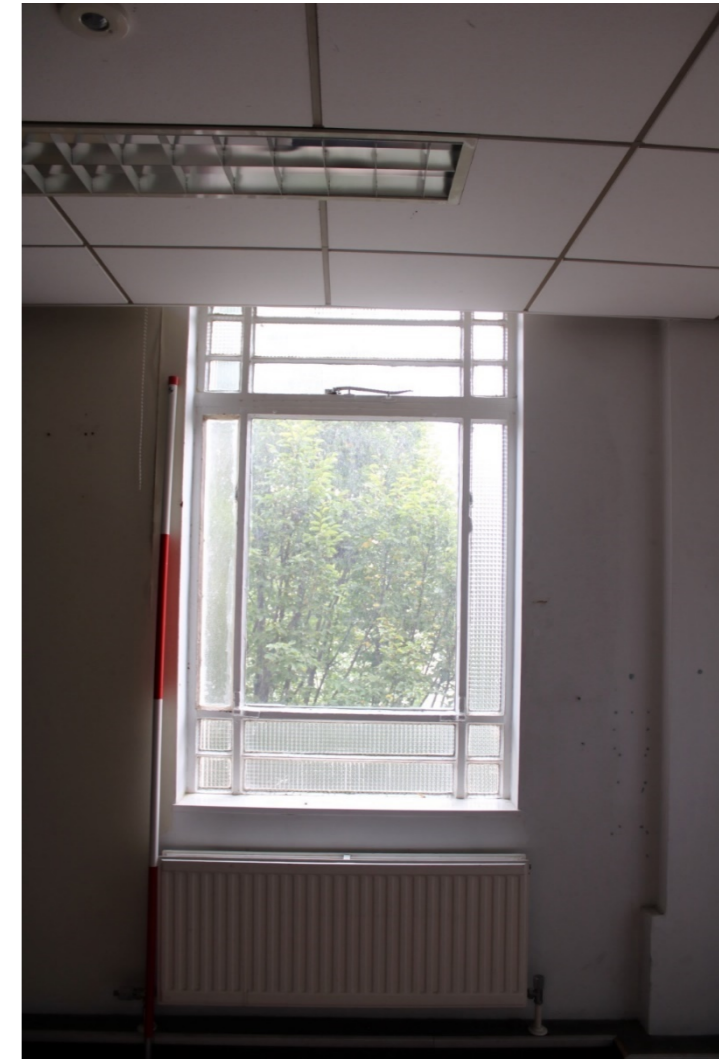
Photo 45: View east of second floor window 9 of central bay overlooking Lister Gate
