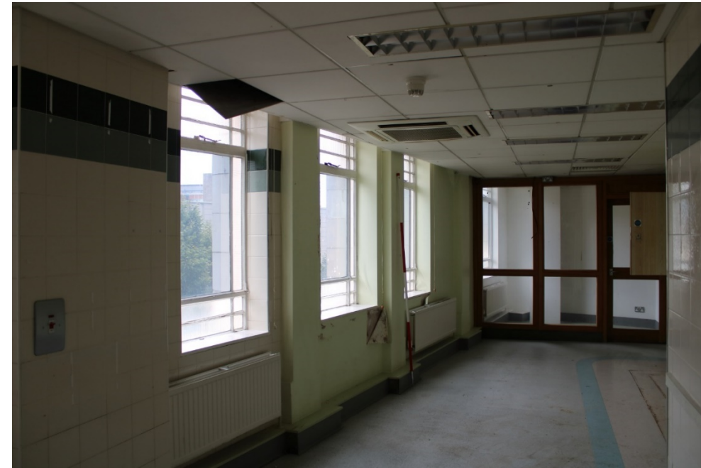
Photo 51: View southeast along staff room towards small end office showing windows 4, 3 and 2 (l to r) of southern side bay in staff room and window 1 of end bay within office to rear
