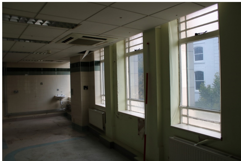
Photo 50: View northeast across second floor windows 5 of central bay and 4, 3 and 2 (l to r) of southern side bay overlooking Lister Gate within end staff room
