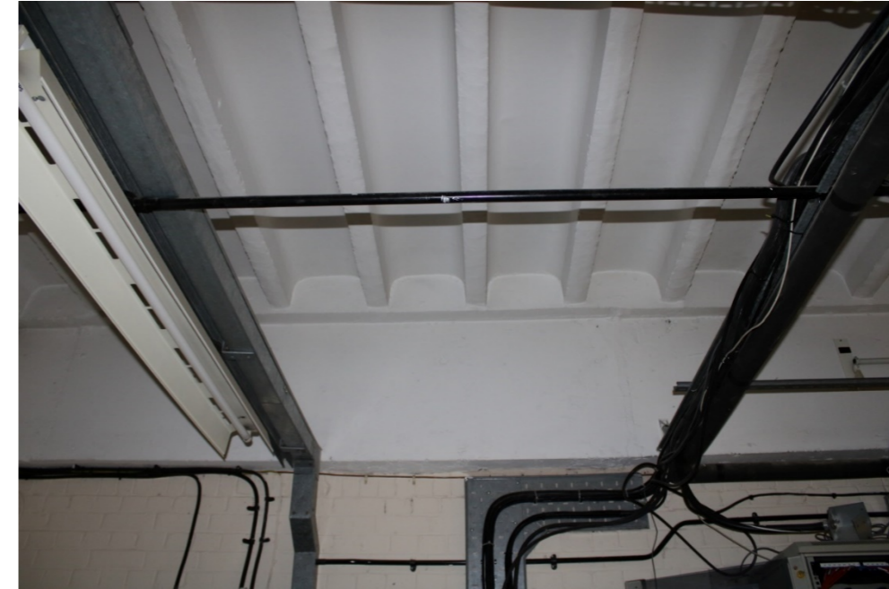
Photo 37: Further view of roof structure in rear storage area showing roof structure on concrete beam
