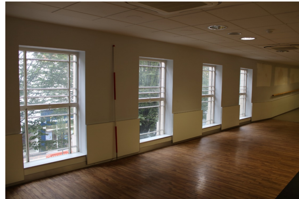
Photo 27: View southeast across first floor windows 6, 7, 8 and 9 of the central bay looking out over Lister Gate
