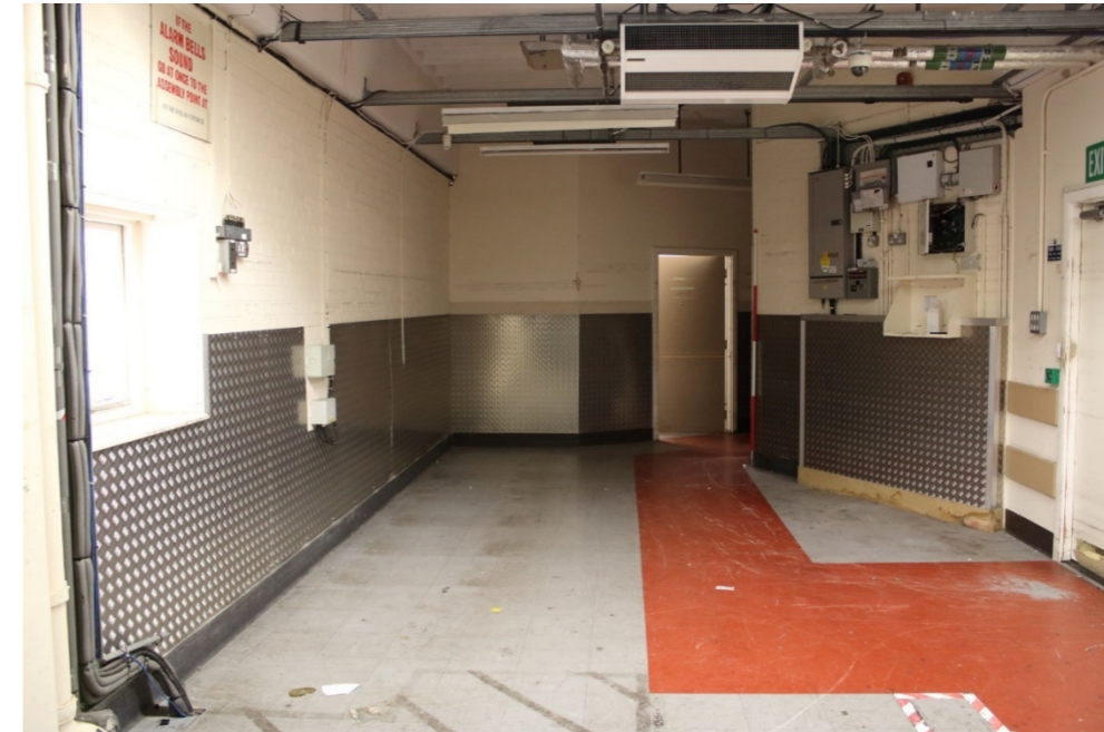
Photo 34: View north along rear storage area to west of first floor retail area with door to right, with corridor and door to office and further plant room to rear and window to yard area to left
