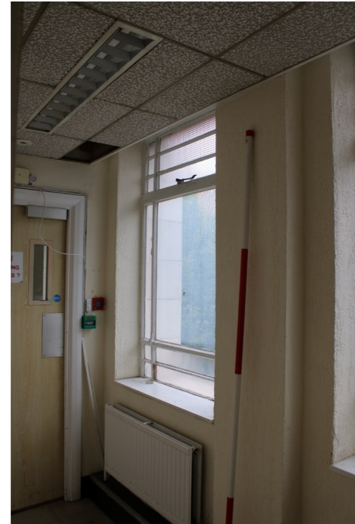
Photo 42: View northeast of second floor window 11 of northern side bay in bathroom south of landing
