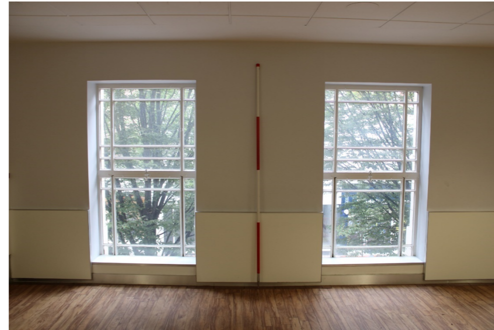
Photo 26: View east of first floor windows 8 and 9 of central bay showing metal window frames and original styling
