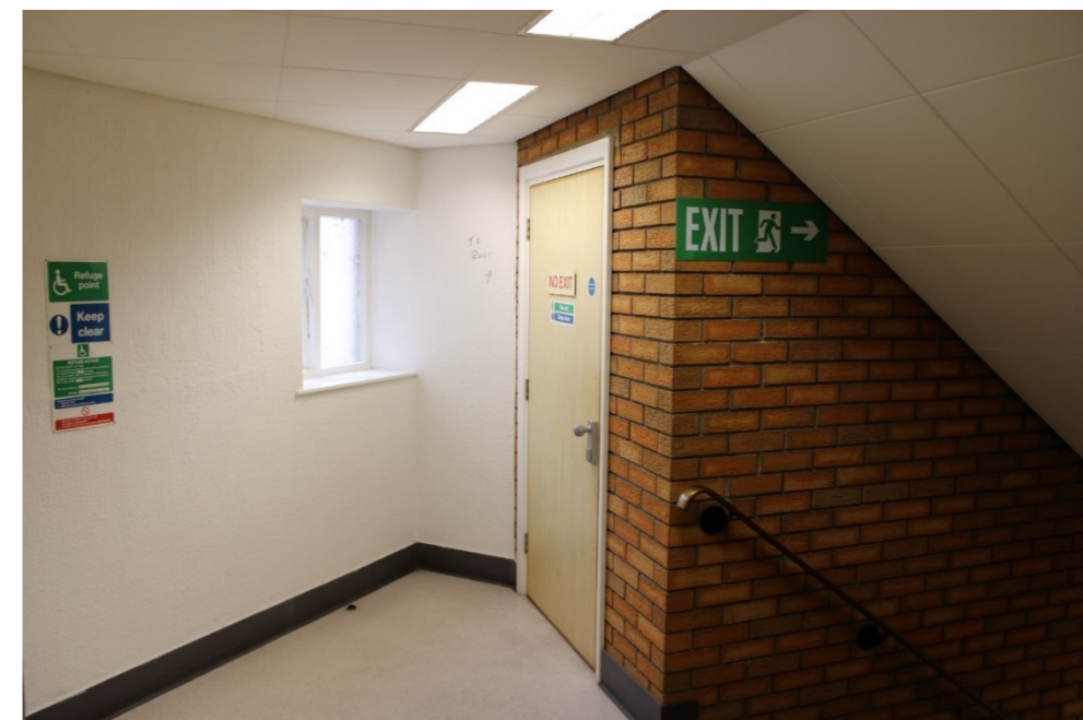
Photo 31: Top of southern stairwell showing window overlooking rear yard area and doorway that leads to the staircase to roof area (not accessed)
