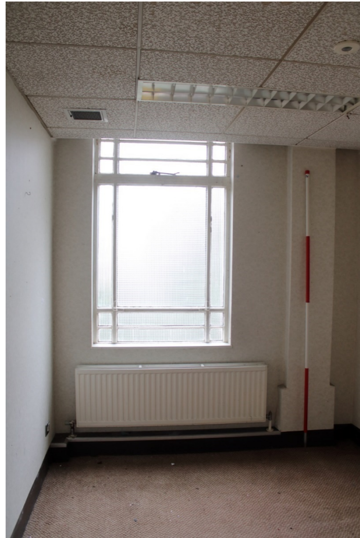
Photo 46: View east of second floor window 8 of central bay overlooking Lister Gate
