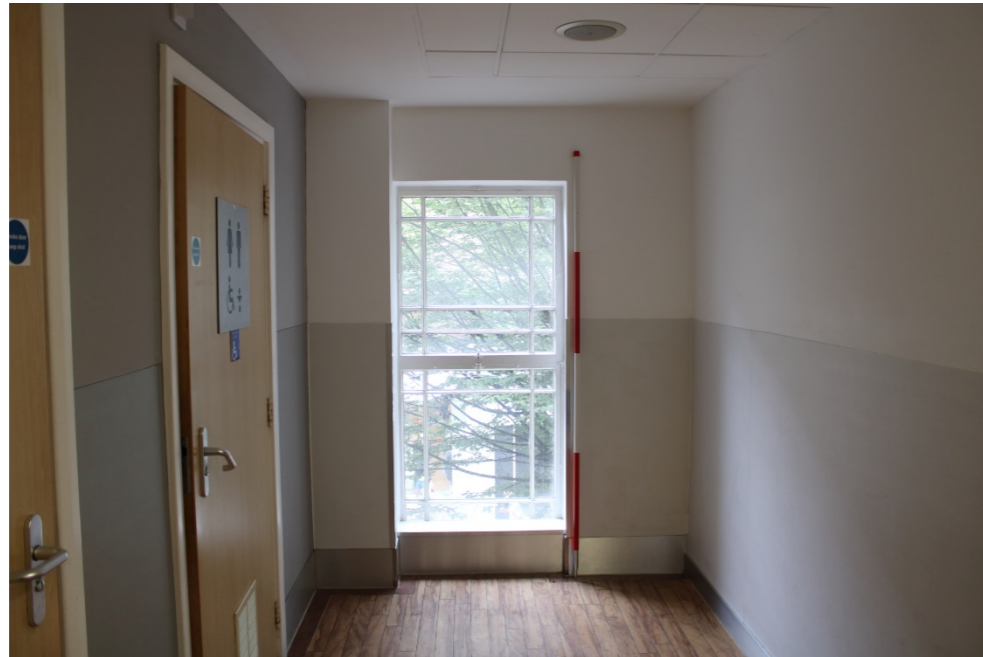
Photo 28: View east of first floor window 10 of northern side bay present within the vestibule area in front of the toilets
