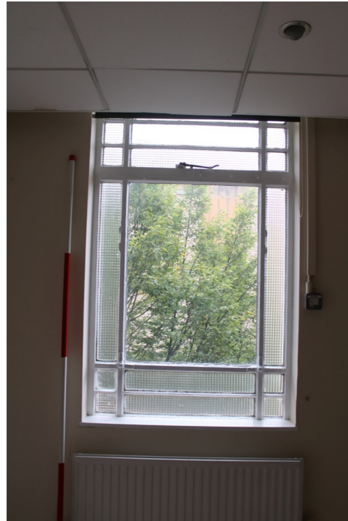
Photo 41: View east of second floor window 13 of northern end bay on Lister Gate frontage located in small office to north of landing
