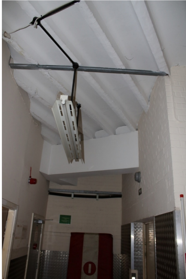
Photo 36: Exposed modern roof structure above storage room to rear of first floor retail area, with large concrete support beam visible
