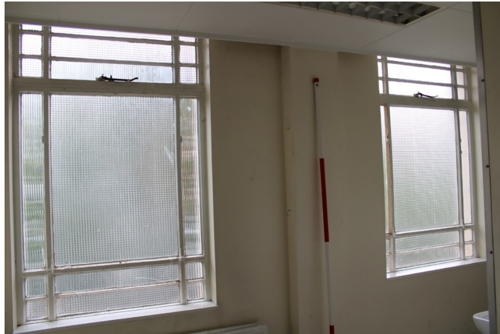
Photo 49: View east-southeast of second floor windows 6 and 7 of central bay overlooking Lister Gate, within toilets accessed off corridor
