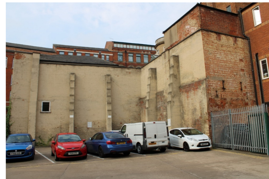
Photo 17: View west of area to north of ramp from Stanford Street showing brick walls with added buttresses. The brick walls survive from previous structures that stood in the rear yard area and which were largely demolished before 1993 but leaving the existing walls standing.
