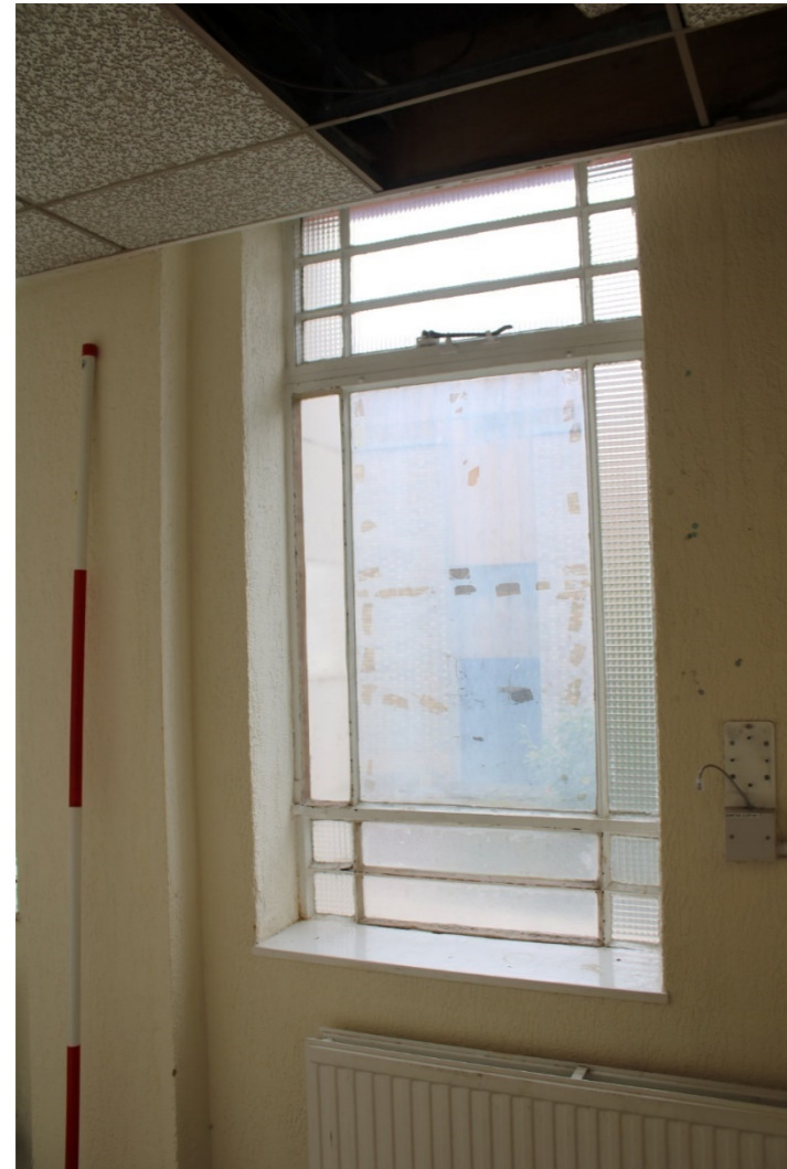
Photo 43: View east-northeast of second floor window 10 of northern side bay in bathroom south of landing
