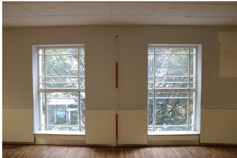
Photo 25: View east of first floor windows 6 and 7 of central bay showing metal window frames and original styling
