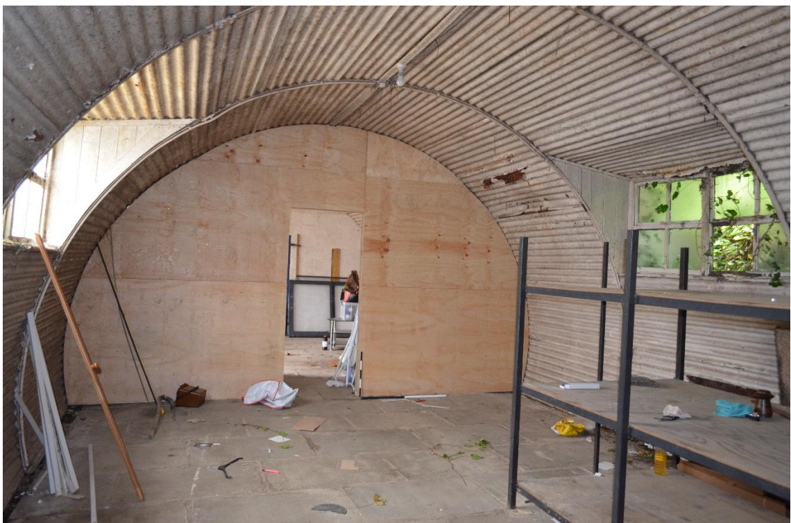
7: The larger northern room looking towards the inserted timber partition. Opposed windows. E
