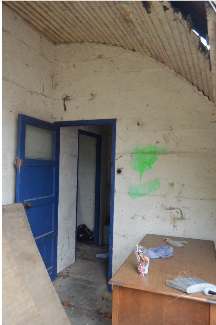
12: One of three smaller rooms at the eastern end of the building, viewed through a collapsed section of wall. Note mid-20 th century four panel door.
