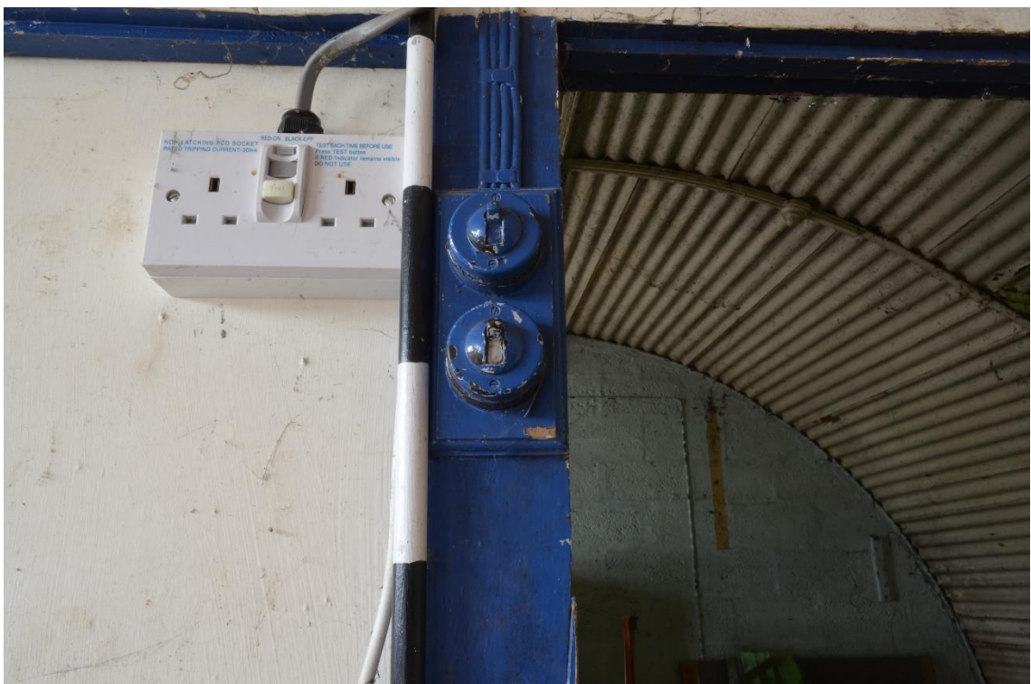
14: Historic light switches with later added modern socket in the central part of the building.
