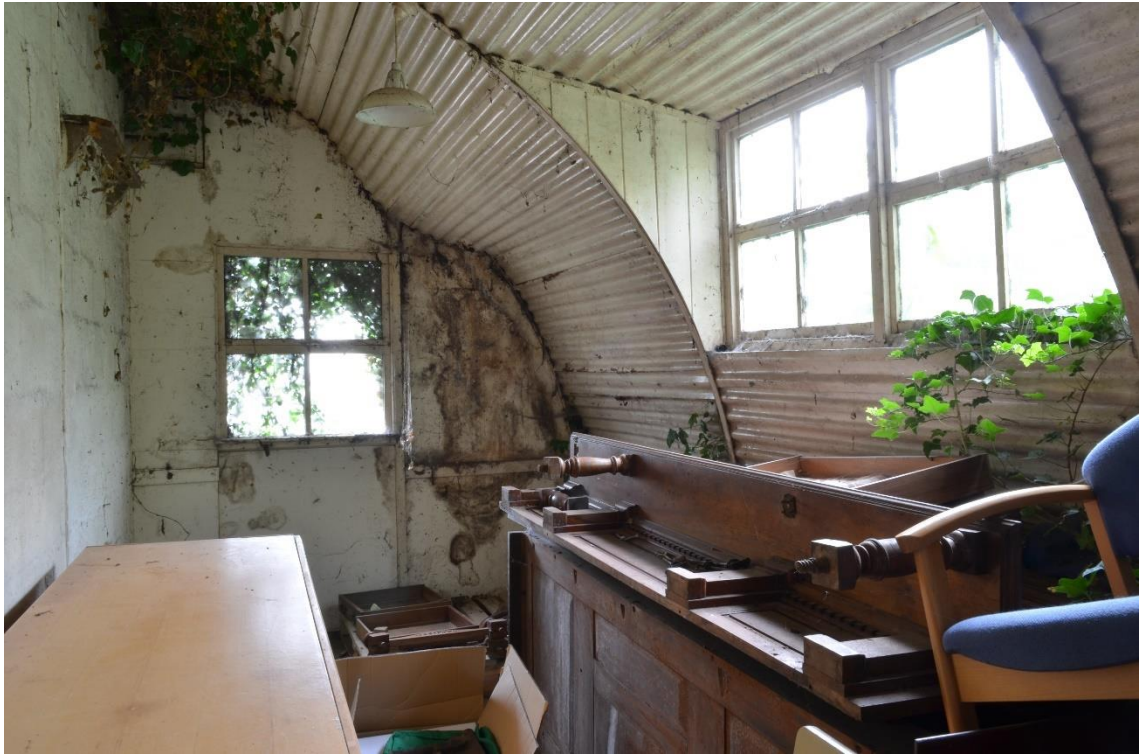
13: South eastern of three small rooms at eastern end of the building. Note plank construction of the window sides and smaller four pane window in the end elevation. SE
