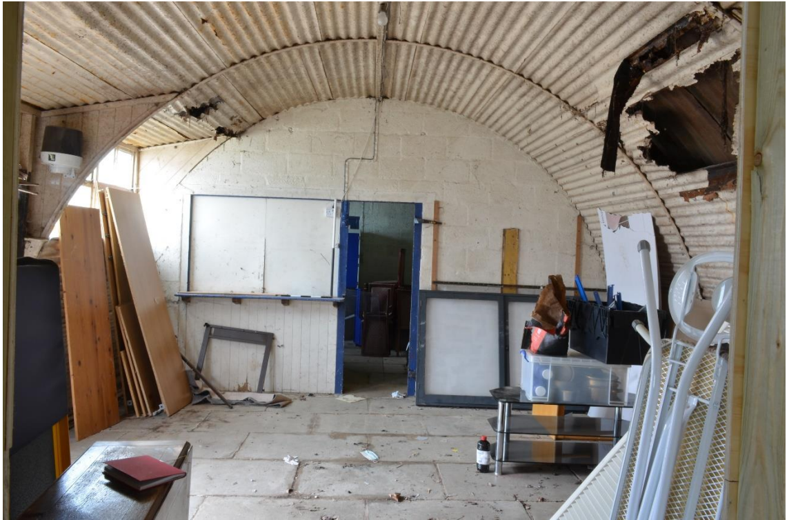
8: Central room looking towards older concrete block wall with central door and serving hatch. E
