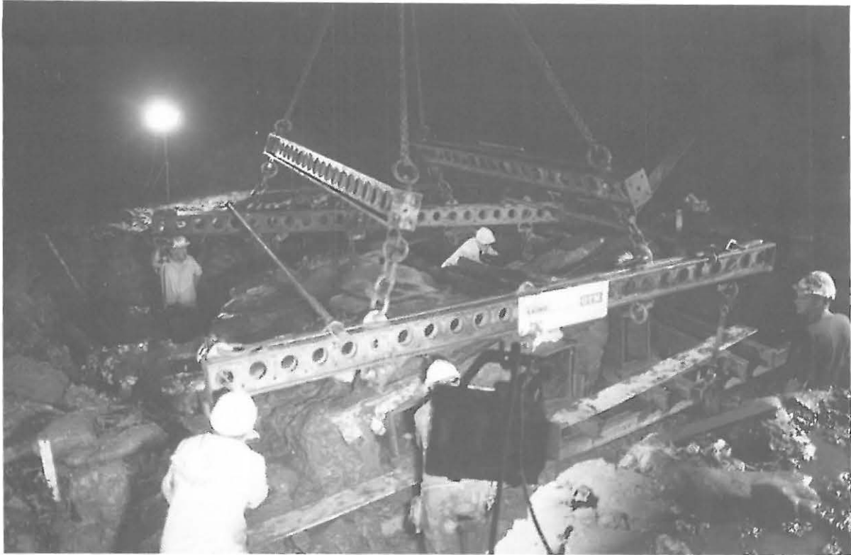
Figure 38. Magor Pill Wreck: The lifting frame taking the weight prior to removal of remaining underlying clay.
