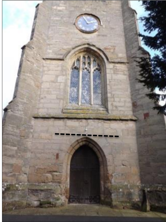
Fig 8: The tower, west face; note the lift scar above the door arch (dashed). The window tracery was extensively conserved in 1997 (see below). The first clock was affixed in 1816 (also below)
