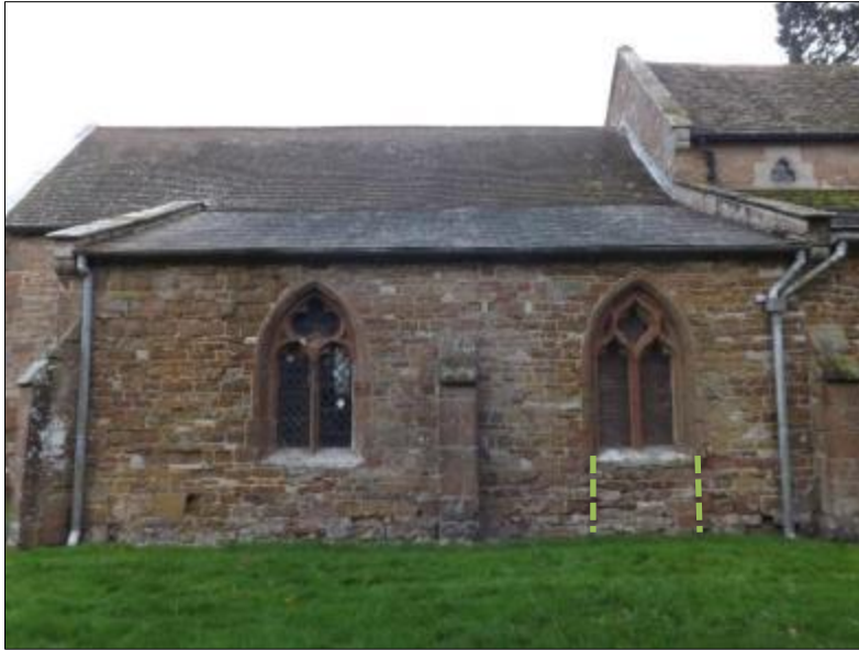
Fig 6: North chancel aisle (chapel/vestry); the window on the right was a doorway until after c1820
