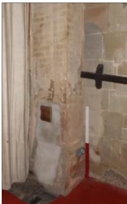
Fig 35: Heating flue in tower, scale 1m. Note the blocked doorway behind and to the right
