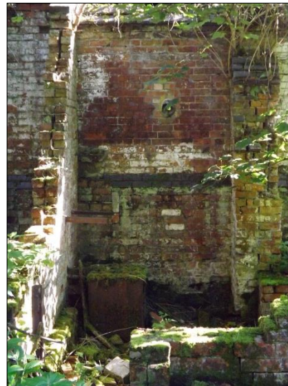
Ruined boiler house on south-west wall
