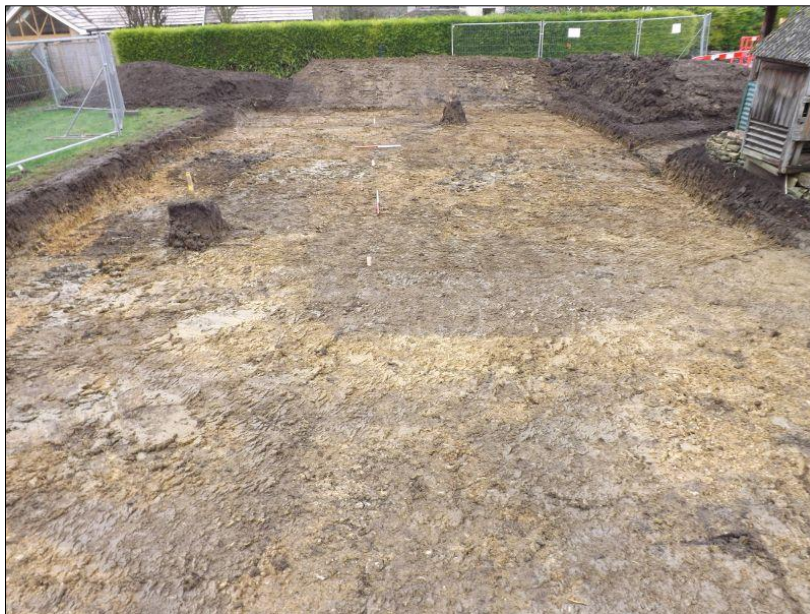
Fig 6: The site, machine-stripped before any hand-excitation, looking north; pegs down centre-line at 5m intervals with scales each 1m
