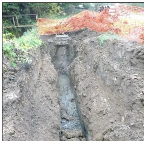
Fig 14: Cutting the new sewer trench south of Area B; stream and bridge behind to left
