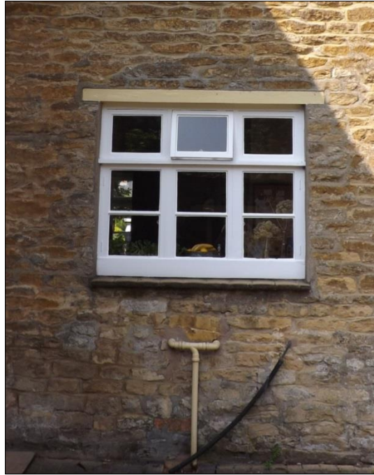
Fig 20: Inserted kitchen window (matching the pantry), with tell-tale mortaring repairs around; the coursing below is awkwardly re-set, suggesting a former doorway direct to the outside well-head
