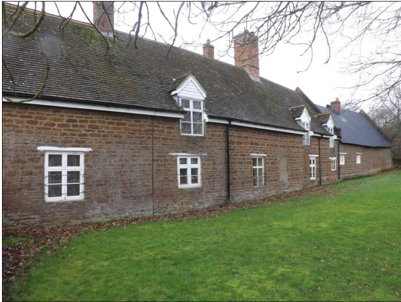
Fig 13: The outside (east face) of the house and the barn beyond. The first floor window locations are no older than later 19 th century. The original eaves were probably lower, with a first floor much more constrained and not specifically for bedrooms, but rather combined with general storage.
