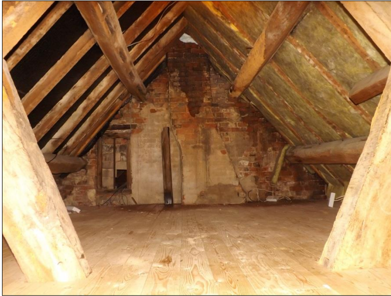
Fig 27: 18 th century range, roof, looking east. Note the re-used timber of the purlin, top left
