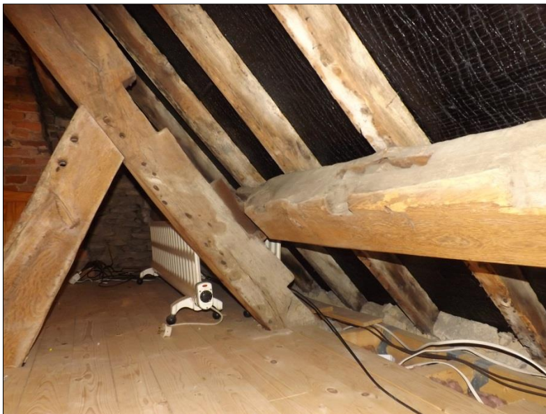
Fig 28: 18 th century range, roof, looking west. Note the original roof arrangement indicated by the two empty purlin trenches in the truss. The replacement purlin is also re-used from elsewhere, being a former wall-plate or purlin turned around, with cut rafter shoes.
