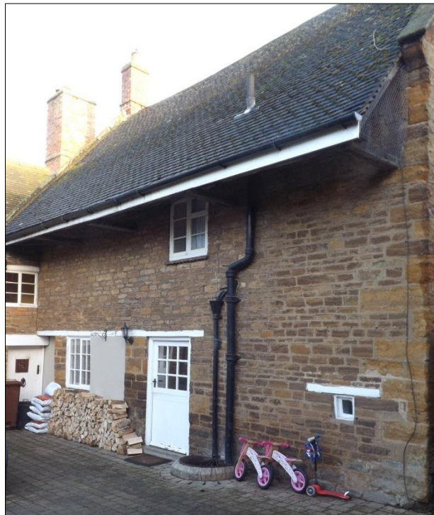
Fig 14: The rear of the 18 th -century addition; much of the long wall beneath the extravagantly-overhanging eaves-drip appears to have been re-built
