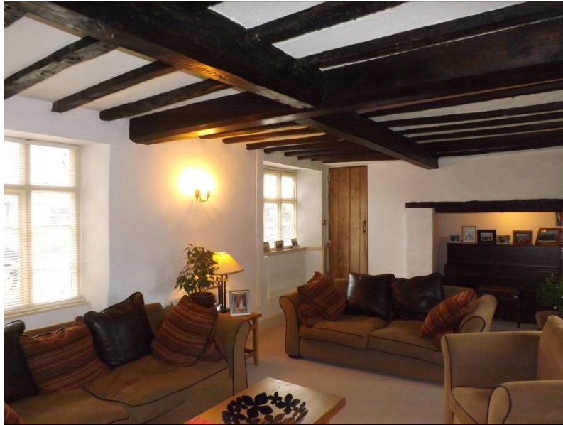
Fig 18: Looking from G5a across G5. An original partition wall is missing from left to right.
