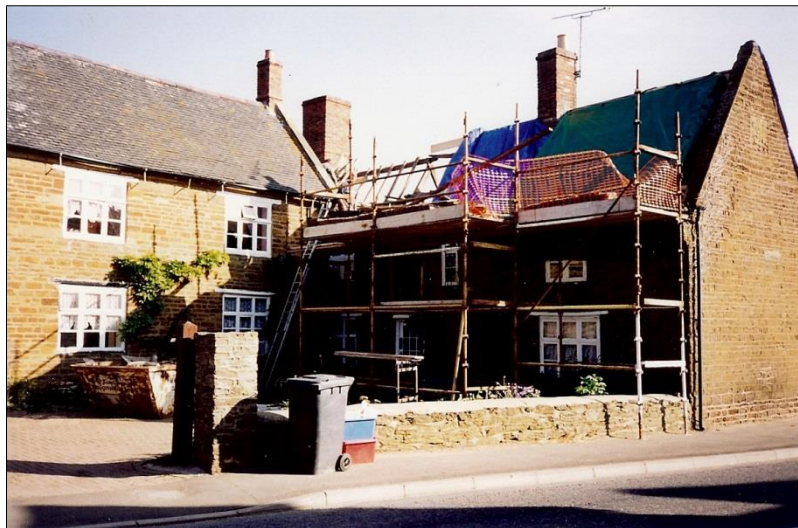
Fig 8: The house during the replacement of its roof-covering in c2000; a part-glazed front door, subsequently replaced.
