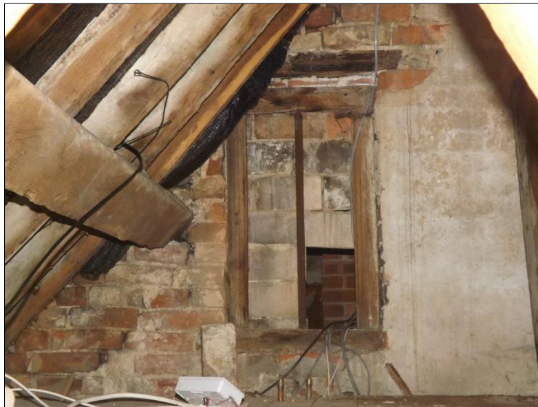
Fig 26: 18 th century range, roof, looking east. Blocked window in brick-lined gable. When thatched, this window looked out over the adjacent roof-slope and the main chimney stack. Slate or tile could not so easily run water away in a curve and the angle (and view) were lost beneath a covering roof junction.
