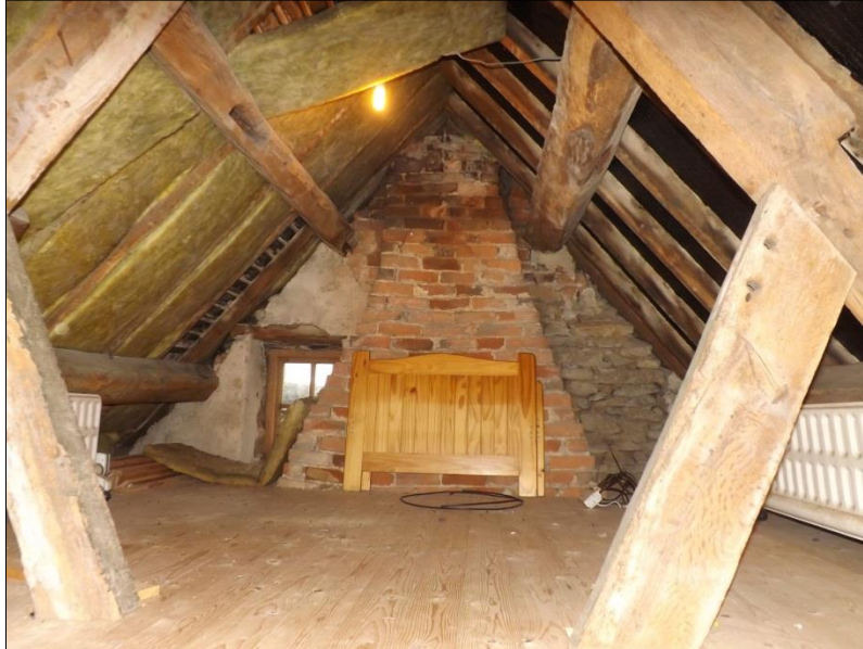
Fig 25: 18 th century range, roof, looking west. Note the window to the left of the chimney-hood
