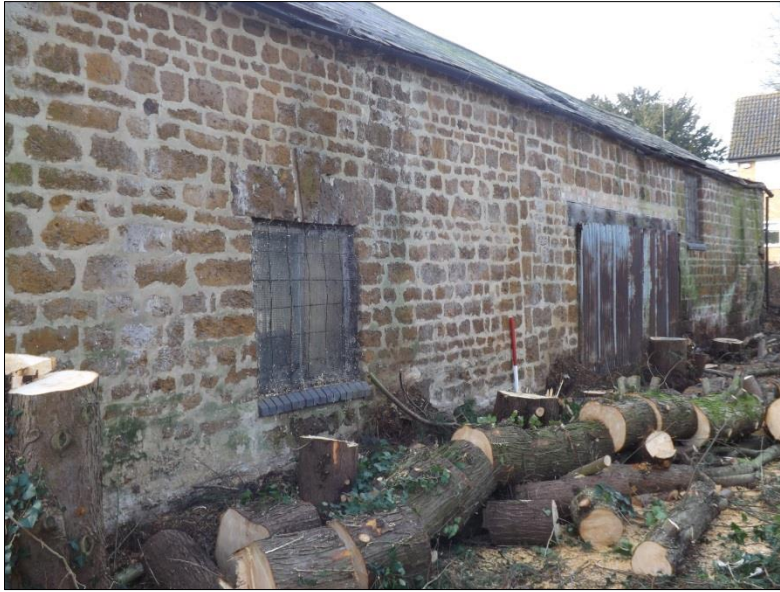
Fig 4: The barn's rear (north) side. Note the prominent butt joint of the two phases; scale 1m
