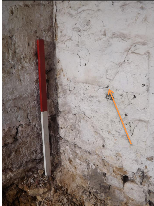
Fig 9: The scar (arrowed) of an animal trough in the eastern half of the barn; scale 1m
