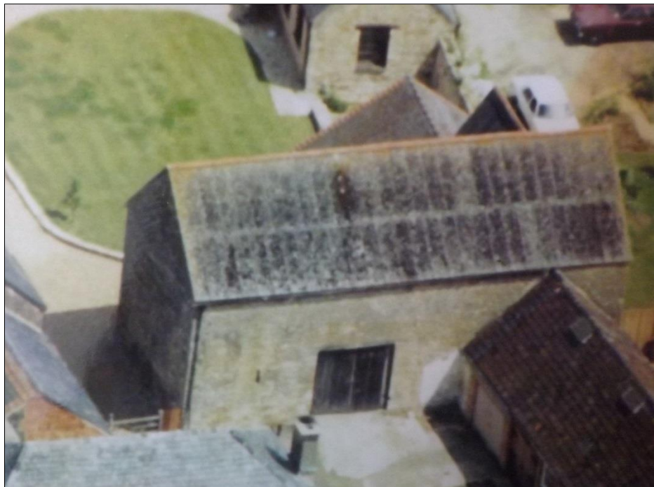
Fig 4: An aerial photo of c1979 from the owner's own collection. Note the barn doors blocked in the recent conversion and the virtual absence of features in the west gable.
