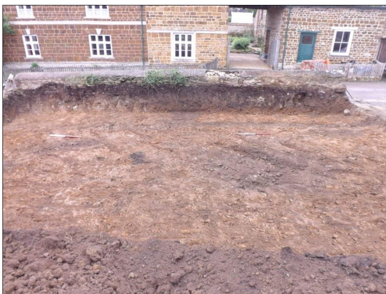
Fig 2: The southern half of the site along Middle Street, newly stripped, looking south; scales 1m
