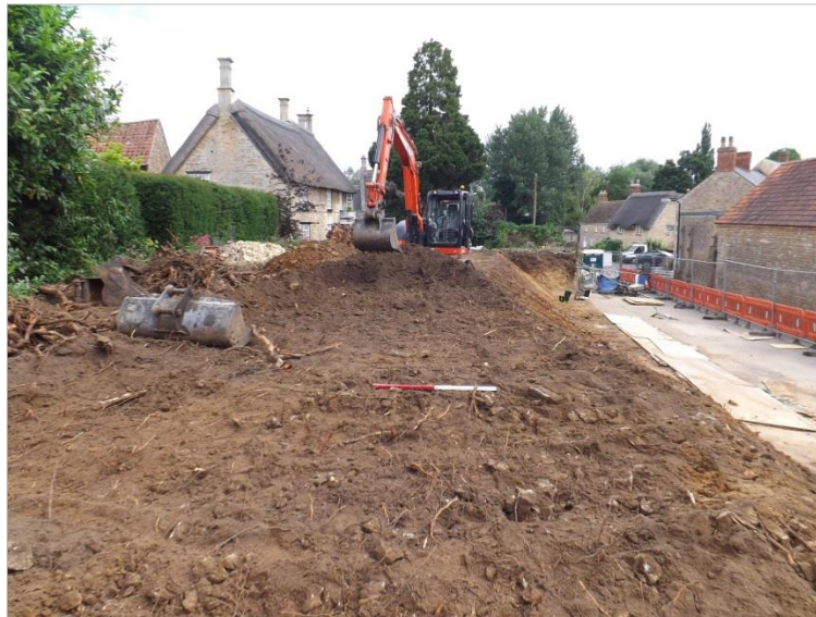
Fig 12: Topsoil strip of the garden to the rear of the wall, looking north-east. Note the far end of the works battered back from the road, recorded in Fig 10; scale 1m
