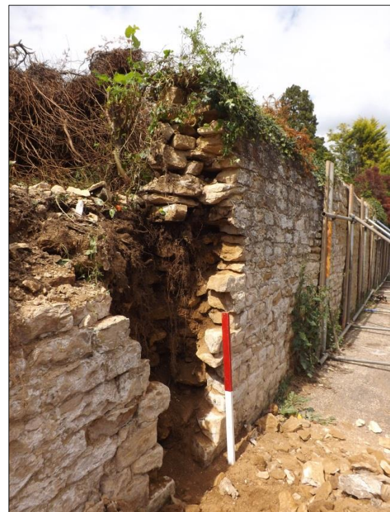
Fig 9: The wall at around 20m from the corner, preparatory to drawing; scale 1m.
