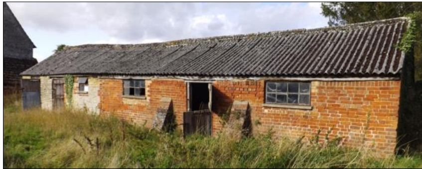
Fig 21: The so-called Barn C, looking north. The gable of Spring Hill farmhouse is to the left
