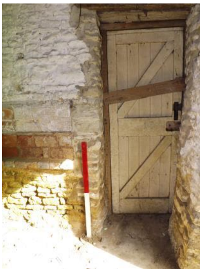
Fig 22: Barn C, west room, interior; note the brick-blocked band at 1m high
