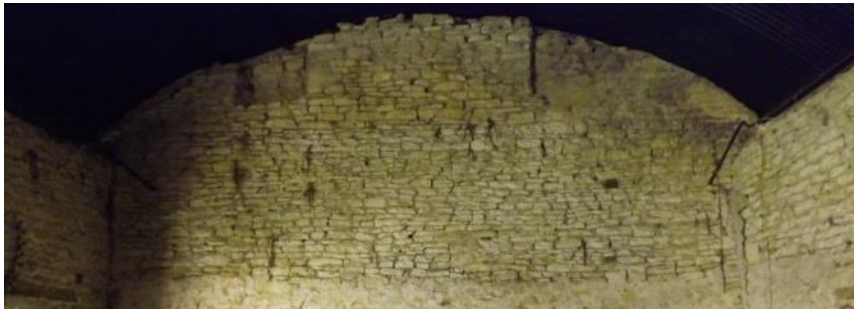
Fig 9: The southern gable's upper portion, with blocked, roof-truncated vents
