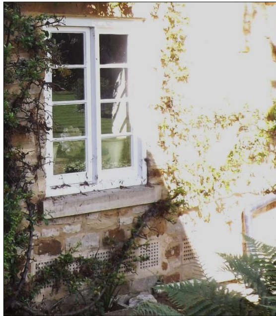
Fig 19: The utility room window, with its majority re-ordered stonework, due partly to six ventilators below
