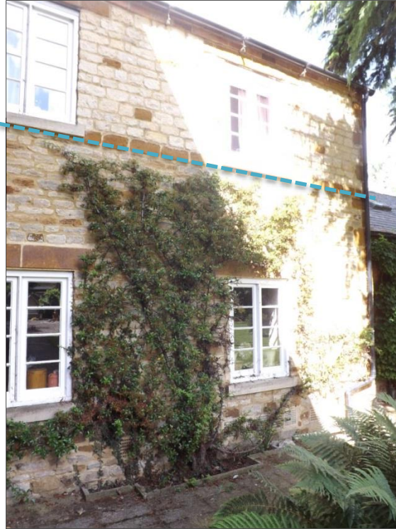
Fig 15: Added rear store wing, from the east. The first floor is entirely modern, the break visible.
