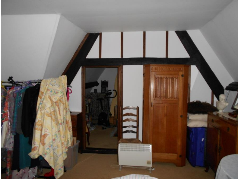
Fig 16: The partition between the north attic bedroom and the dividing wall on the line of the principal truss, looking south into the other bedroom
