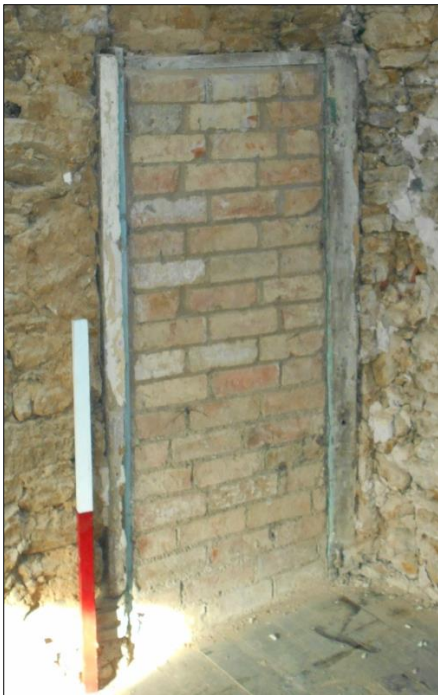
Fig 12: Blocked diminutive access doorway in NW corner of western bedroom (to no 6, next-door); scale 1m
