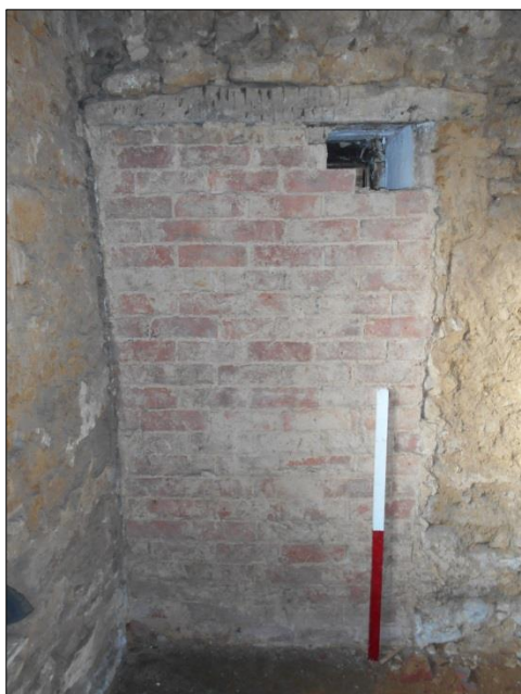
Fig 5: Blocked doorway from kitchen to hall; scale 1m
