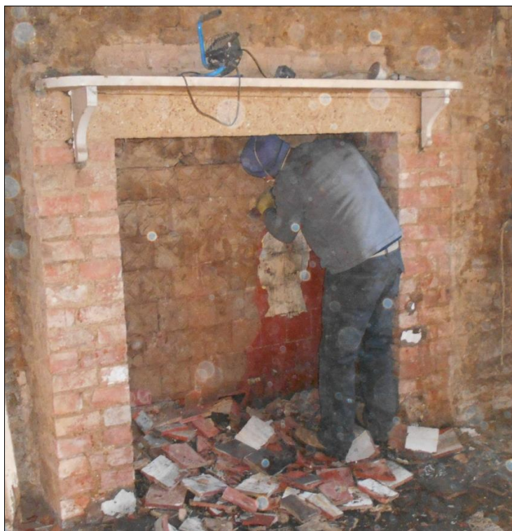
Fig 4: Paring back to the stone and brick on the east wall of the eastern room (kitchen)
