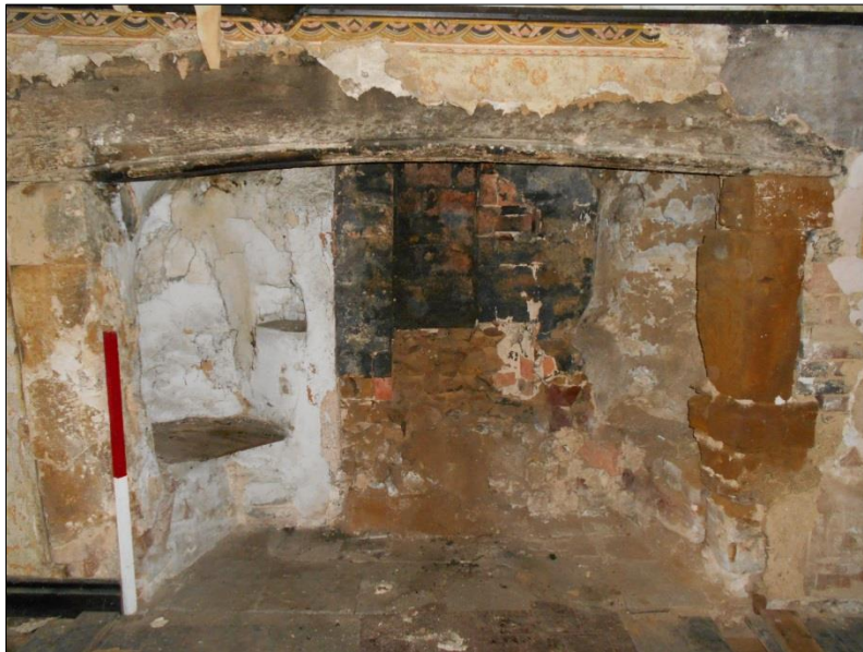
Fig 1: The western room inglenook, fully cleared; scale 1m. Note the seat-niches and tankard-rest
