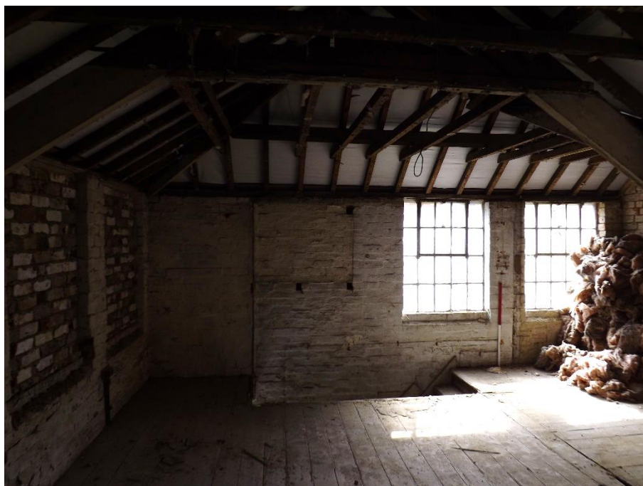
Fig 10: First floor, looking south (scar of timber partition wall to right of 1m scale)
