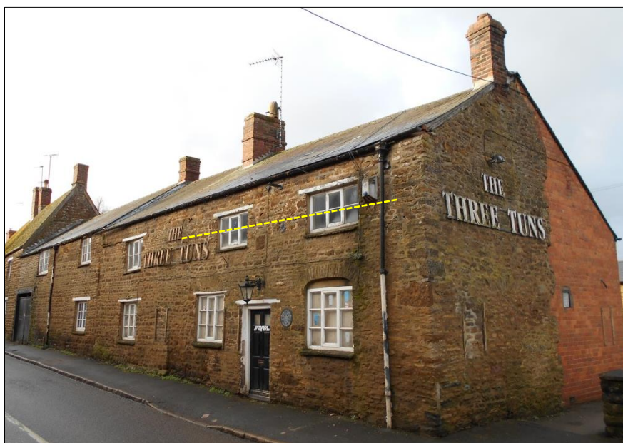
Fig 5: Three Tuns' long building frontage, from across the road. The earlier phase is nearest the camera. Note the through carriageway at far left. The dotted yellow line marks the stonework change where the original eaves were raised and the current windows cut.
