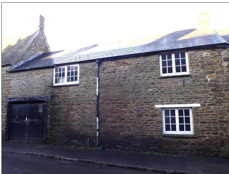
Fig 11 : The plain front of the former added service range with carriage entrance. Note the butt-joint at the right.
