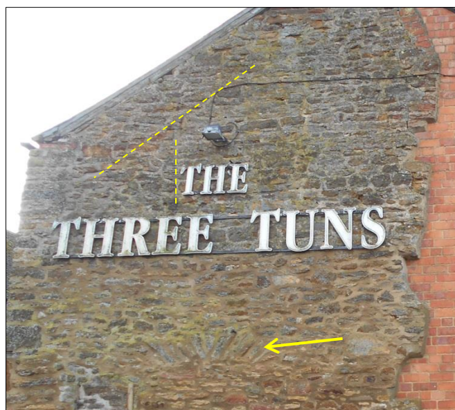
Fig 10: the former roofline in the north gable; a butt-joint may mark a former window, or possibly an attic-level hatch into the lost adjacent building; note also the blocked window or fireplace lintel arch on the ground floor (arrowed)
