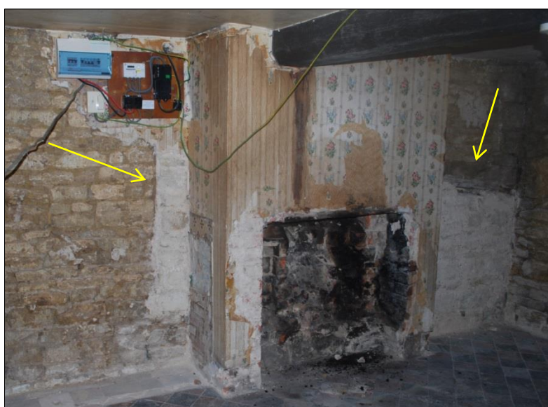
Fig 12: Room G2, looking north-west showing inserted chimney breast, blocked window (left) and blocked fireplace (right, both arrowed)
