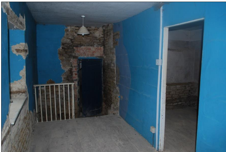
Fig 14: Landing, F1, looking east towards the blocked window and store doorway; note the flimsy stud partition with F2 on the right
