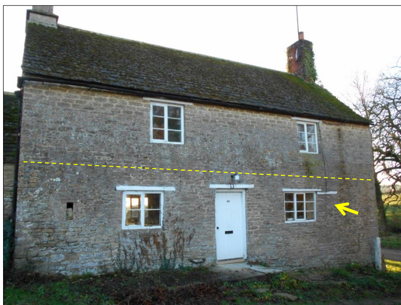
Fig 6: The north face of the cottage, showing the old eaves line and original blocked window (arrowed)
