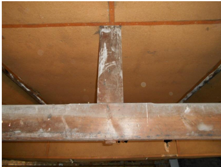
Fig 18: The part-covered roof truss at the junction between S2 and S4, viewed from S4. Unlike all other roof elements, it is chamfered (if only simply) and varnished. Its upper reaches are boarded-in and hidden.
