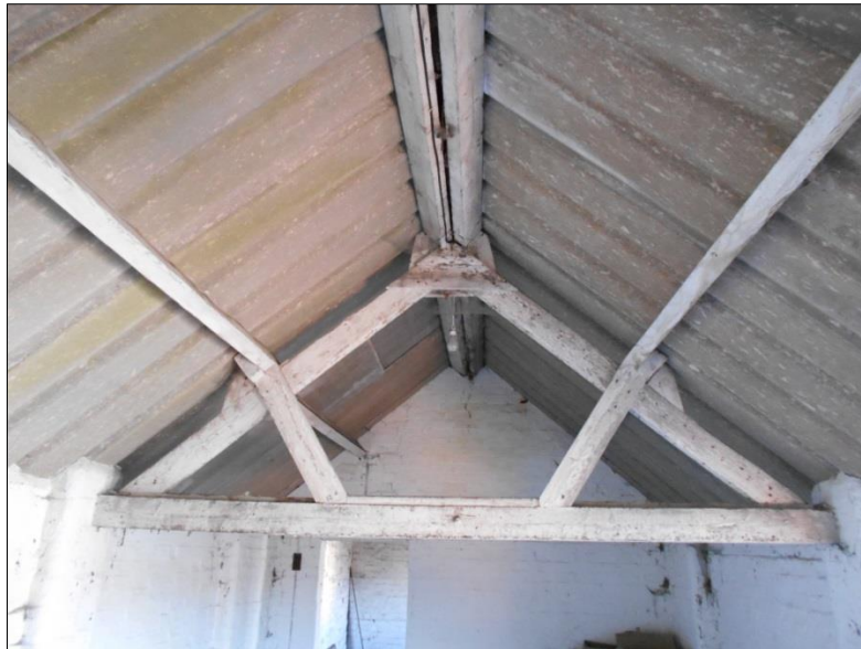
Fig 17: The roof in Room S1, showing the simple and relatively flimsy truss
