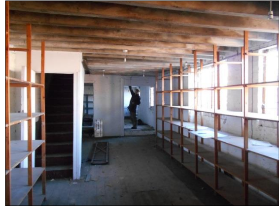
Fig 16: F3 Interior, looking north towards the back of the chimney breast in F1; boxed-in stair to left
