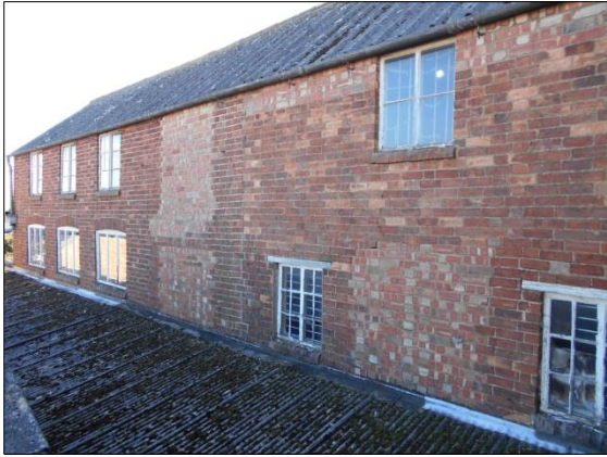
Fig 15: The secondary block with F3 and S3 to left; note possible blocked loading bay doorway at second floor level
