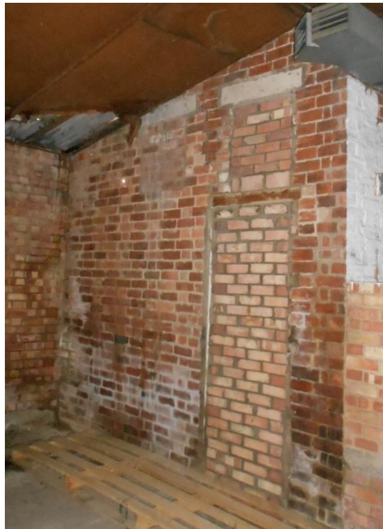
Fig 13: G3, south wall with blockings, viewed from a later room to the south
