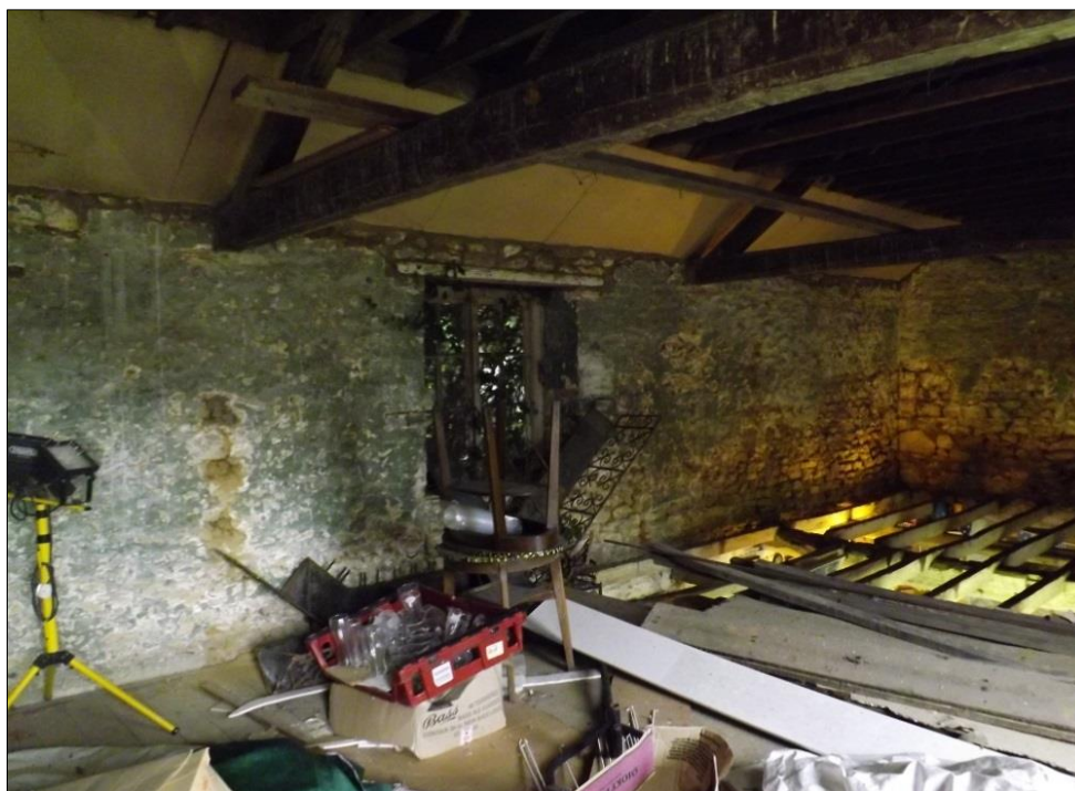
Fig 10: The first floor level looking north-east. Note lack of floorboards at the eastern end and ivy-covered window in the centre of the north wall.
