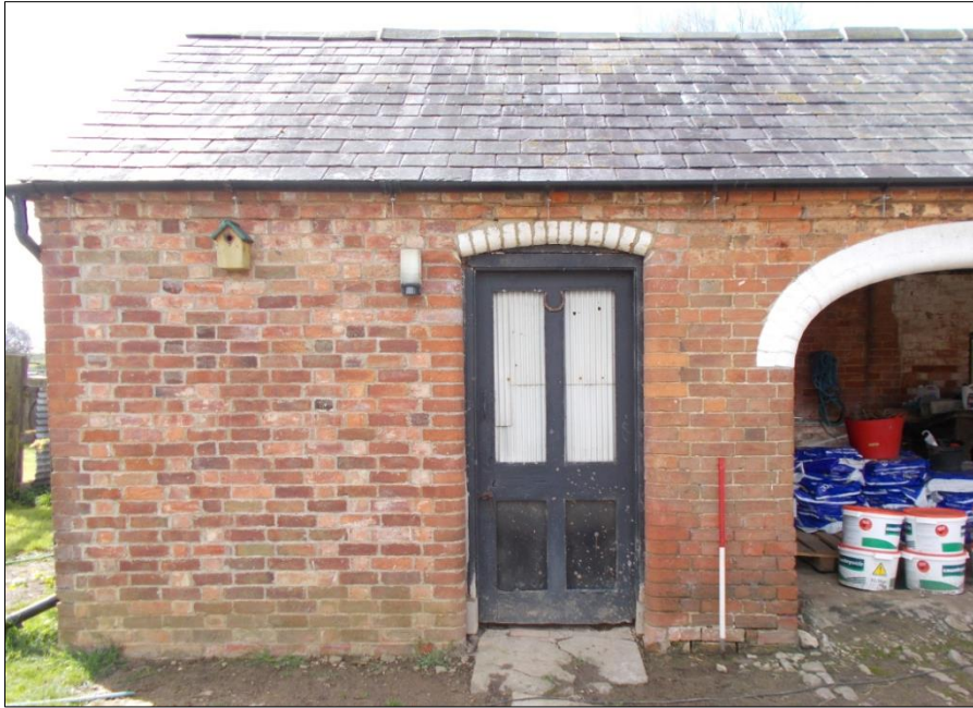
Fig 4: The north elevation of the former meat larder looking south; 1m scale.
