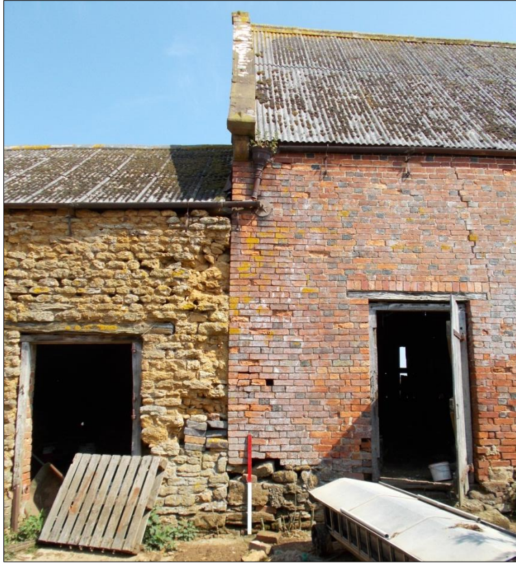
Fig 6: The south elevation of the field barn showing doorway into the barn (and later animal shelter to the left) looking north; 1m scale.
