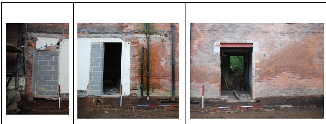
Fig 5: Composite photo-montage showing the exposed rear of the 1886 building after demolition of the modern accretions and ground reduction. Scales 1m and 2m
