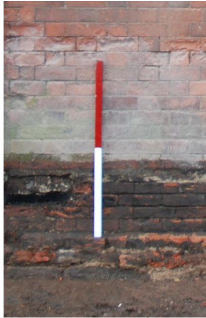
Fig 6: Detail showing the flimsy brick offset and single course of stone foundation; scale 1m
