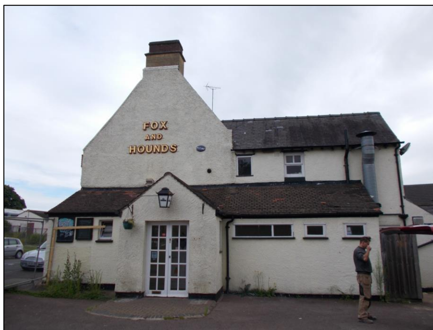
Fig 6: The west elevation, looking east. Later additions at ground level foreground and to both storeys to the right.
