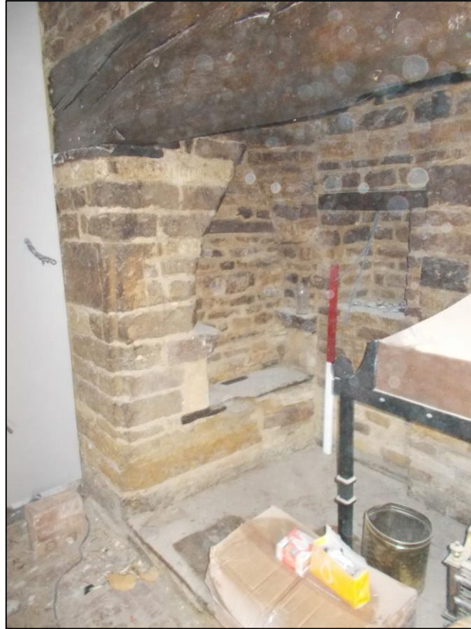
Fig 9: The built-in seat in the south wall of the inglenook looking south-west; 1m scale. Note also the recess in the west wall.
