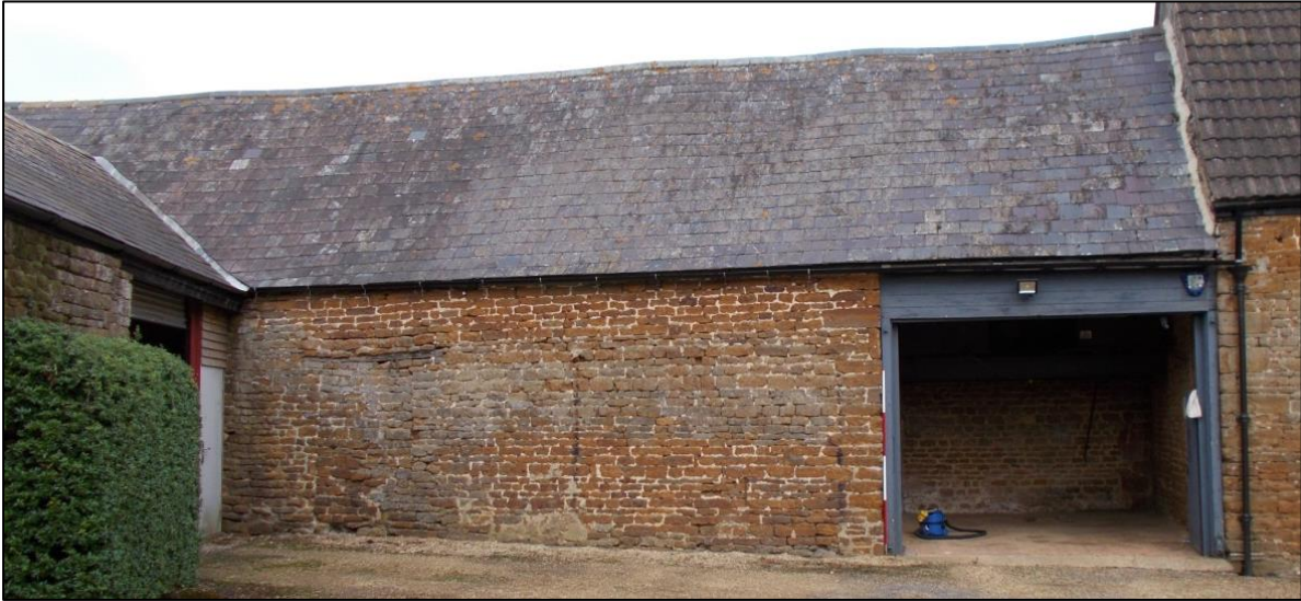
Fig 11: The south elevation of the 2 nd phase barn, looking north; 2m scale.
