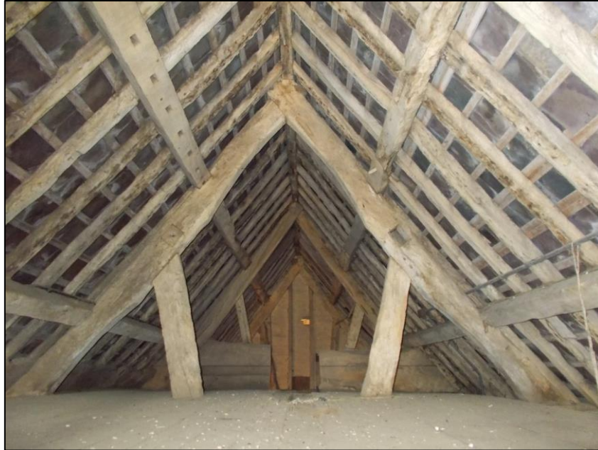
Fig 13: The roof of the 2 nd phase barn, looking east. Note the lath and plaster infill within the far truss above the brick wall which forms the west side of the coach-house.
