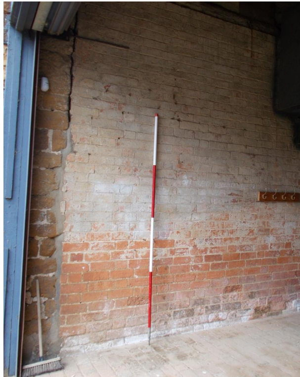
Fig 12: The 2 nd phase barn with inserted brick wall at the east end, looking north-west; 2m scale.
