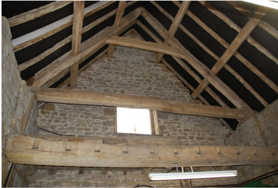
Fig 9: The 17 th century service range roof, looking east towards the later east gable wall.
