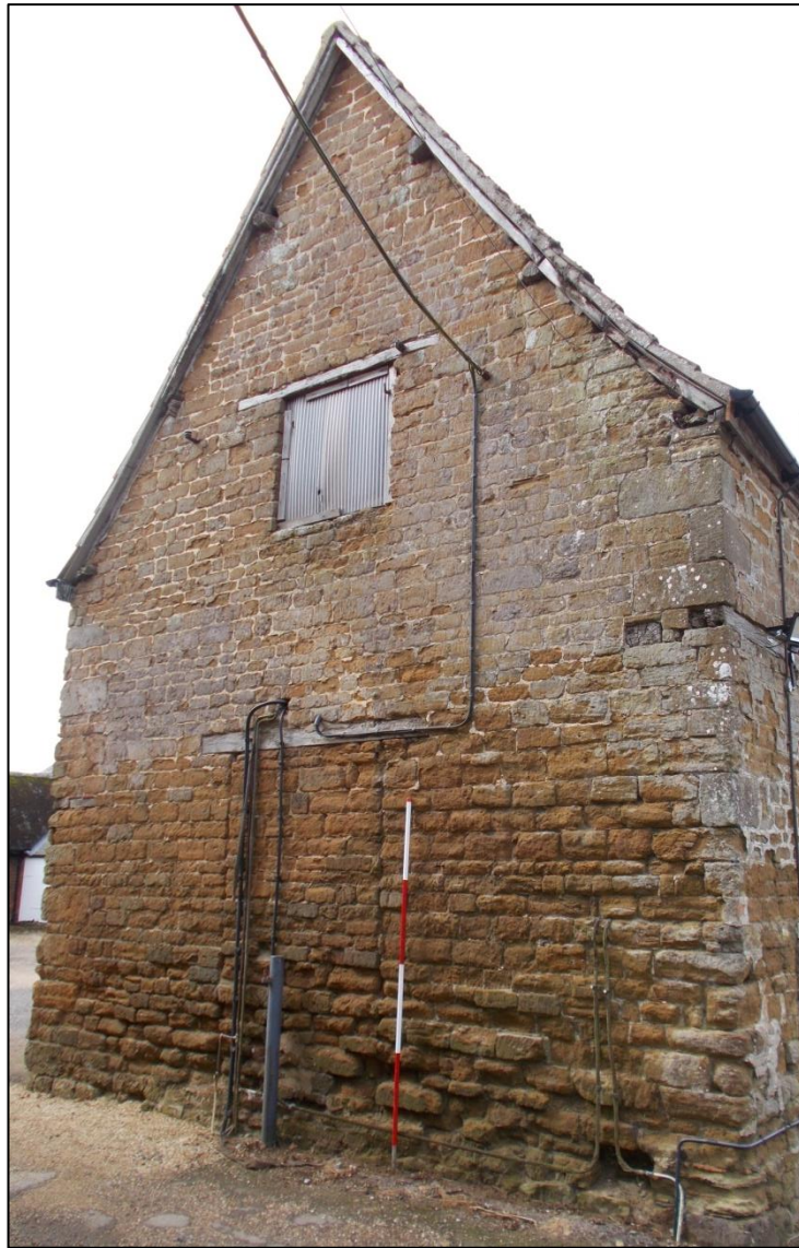
Fig 7: The east gable inserted when the service range was separated from the farmhouse, looking south-west; 2m scale. Secondary infilled door and hayloft door.
