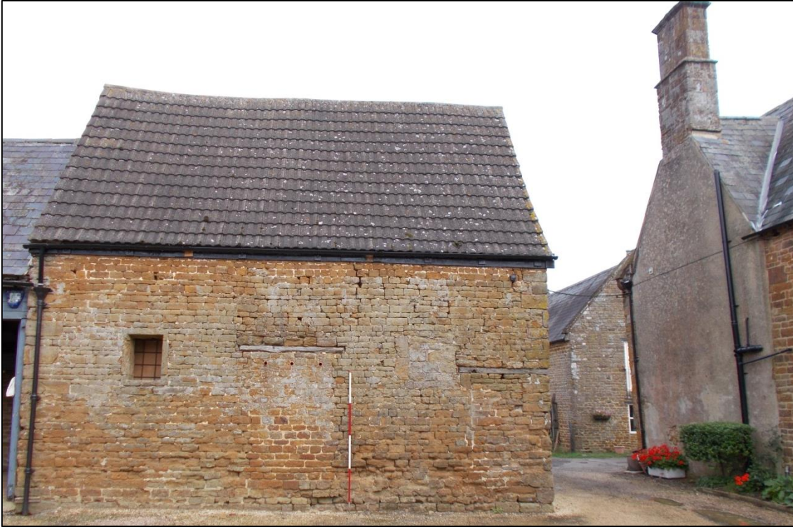
Fig 6: The south elevation of the 17 th century service range, looking north; 2m scale. Note the vertical edge of the rendering on the chimney stack gable of the farmhouse to the right.
