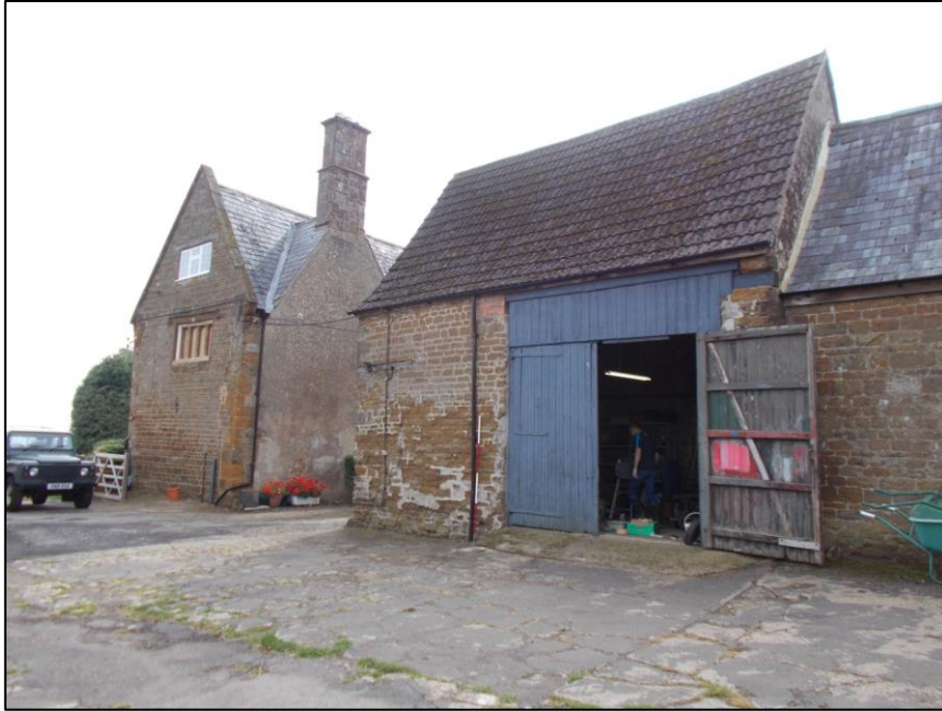
Fig 5: The north elevation of the 17 th century service range, looking south-east; 2m scale. The original farmhouse lies to the left; note the rendered west wall beneath the chimney stack.
