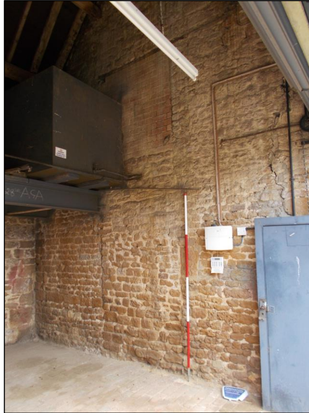
Fig 8: The west gable of the 17 th century service range, looking north-east; 2m scale.
