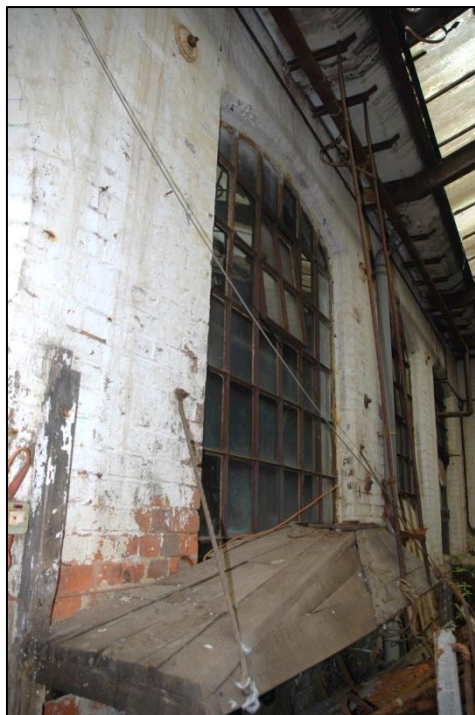
Fig 78: The shaped wooden fume-hood at shoulder-height; an exit pipe to the roof is missing.
