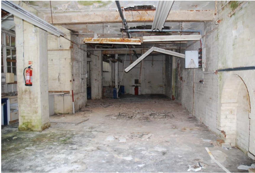
Fig 104: Room EG25 looking west towards a stamp battery in far left behind the WC block, verandah to far left; scale 1m
