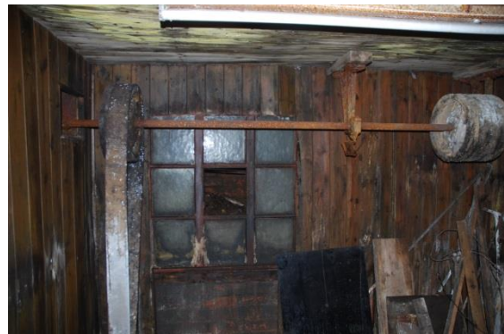
Fig 86: The surviving basement light well in west wall of EB04, with drive shaft and drive-wheel (top left), with belt still attached
