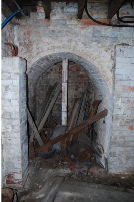
Fig 33: Arched alcove in north-west corner of EB11, containing a collection of cast-iron wheels from a drive-shaft. The arch supported the stairs above, while to both left and right stand two World-War II Fletton-brick buttresses. Most of the basements are highly cluttered like this.
