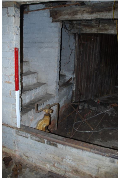
Fig 82: A pair of truncated brick steps (EB05), the lowest two treads and risers removed. 1m scale stands on a bund wall, built to keep an oil spillage in from an adjacent tank.
