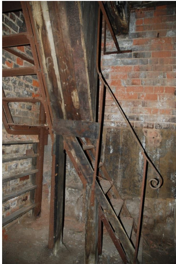
Fig 65: The steep cast iron stair in EG54. Probably the prime staircase in the 1897 rear shopping
