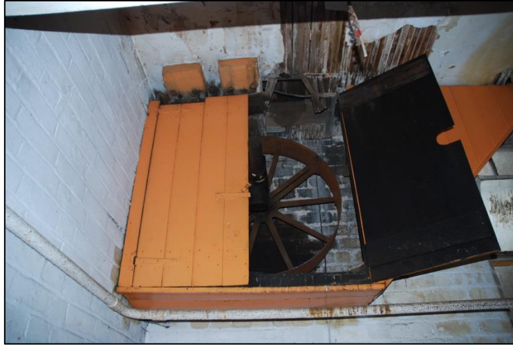
Fig 42: High in the west wall of room EF64, the Beverley Hall Ltd Warehouse, but built as a 'New Silver Room' in 1897. The boxed-in wheel and drive shaft, cut off on the far side of the wall in EF59
