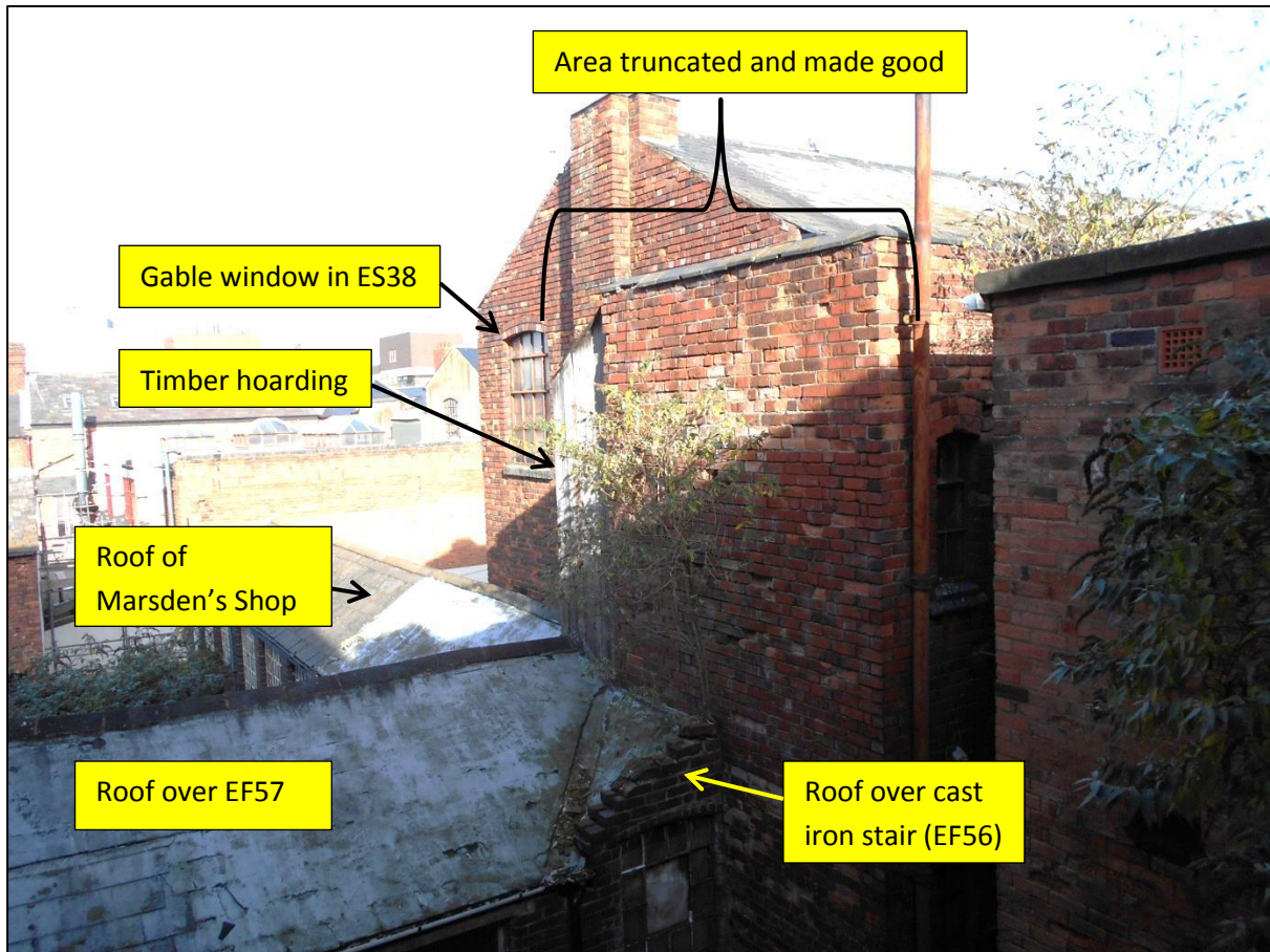
Fig 67: The truncated building end between the second floor rear shopping (ES39) and the earlier buildings to the rear, looking north out of ES29. A scar up the end wall of the plot shows that these were once taller, while the brickwork above the cast iron stair has clearly been truncated and made good, if rather haphazardly. The blank end wall and blue brick coping over the end of the toilet block may indicate a massive brick sticking-plaster.
