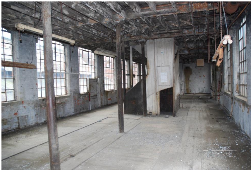
Fig 56: Room EF47 (Spinning Shop) looking west. Note a bearing grease mark on the end wall.
