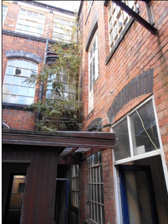
Fig 81: The tiny visible portion of the frontage visible from the rear yard. Note how the southern range of shopping (right) cuts across the edge of a rear-facing window.
