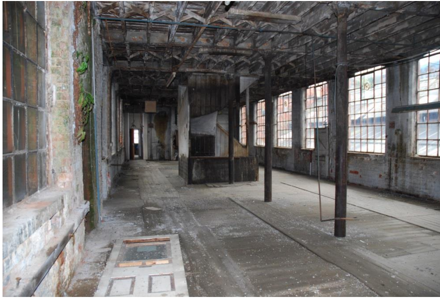
Fig 57: Room EF47 (Spinning Shop) looking east. Note the slightly raised walkways with thickened reinforced timber.
