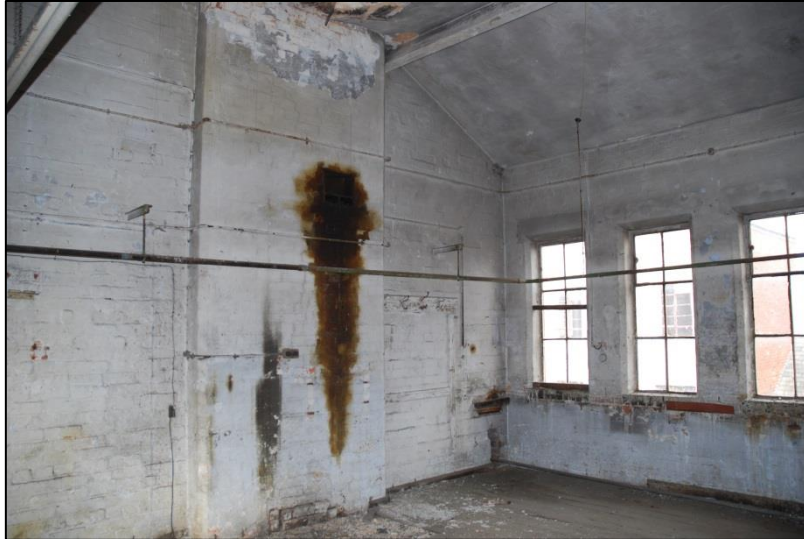
Fig 44: Room ES41. The grease mark from a wall-mounted drive shaft bearing (one of a set of four) the only room at second floor level to contain them. It is unclear where the drive came from, although a discrete electric motor mounted on the second floor seems likely. Note the blocked fireplace and hearth with kerb in the gable.
