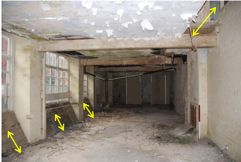
Fig 107: Room EF32 looking east. Note the window-protection and additional natural light afforded by the ceiling gaps and angled boards (arrowed). The steel frame is very clear. Note the bottom corner of the second-floor window (top right), which added light into the first floor from under the benches above
