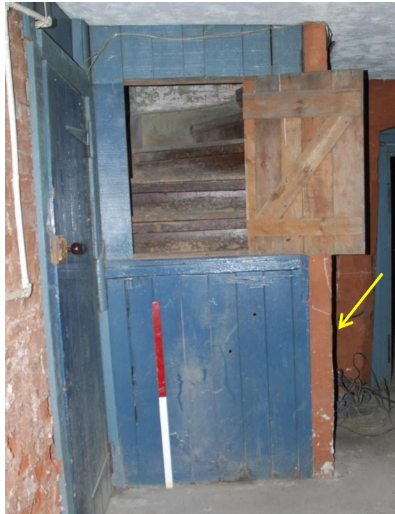
Fig 35: Blanked off and boxed-in stairs in EG 39, looking north towards the winding flight up, once to EF42. The arrow shows the location of the winder downwards in the side-face, once to EB14; Scale 1m
