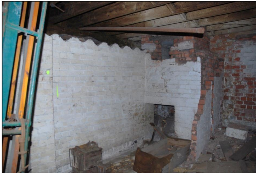
Fig 28: Dividing wall in basement room EB10 (looking East) entirely of Flettons in English Bond with corrugations denoting former inserted roof line under the ground floor joists of EG31
