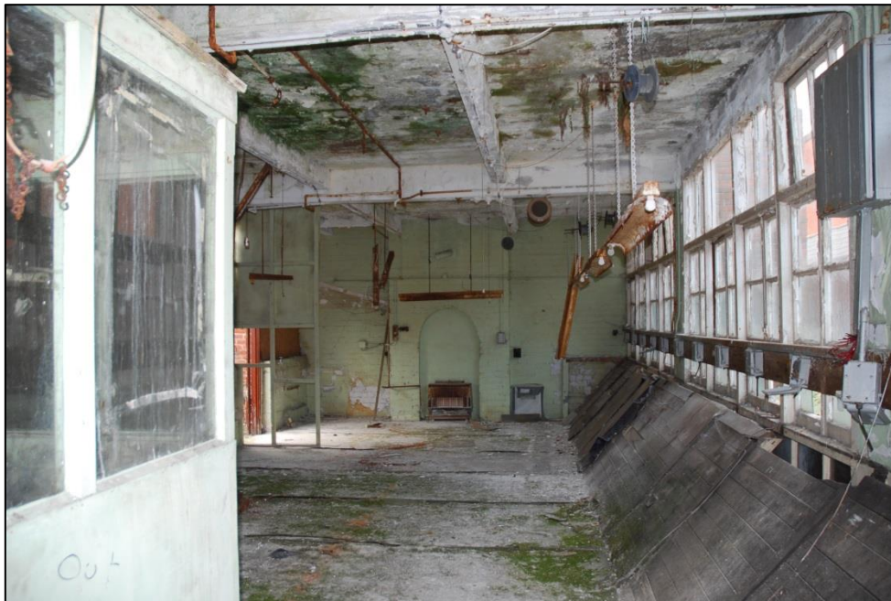
Fig 110: Room ES14 looking west, with annealing hearth at the end. The angled boards protect the lower third of the blinded windows from feet and from dropped materials and tools from the benches, now gone. They also made sure the floor below benefited from their light. On the applied mid-rail are mounted numerous electrical points. Note the circular tannoy-type speaker on the ceiling.
