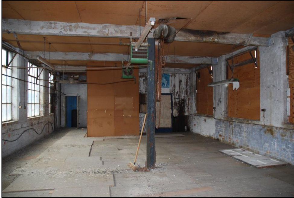
Fig 66: Room ES39 looking west, the end partitioned in modern times to provide an office space. A chain-hoist is fixed next to the supporting post.
