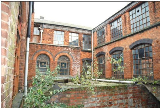
Fig 24: View from EF59 doorway to EF52 east across across roof of the Polishing shop and toilets (flat roofs) showing rear of frontage range and north face of EF47 and ES29
