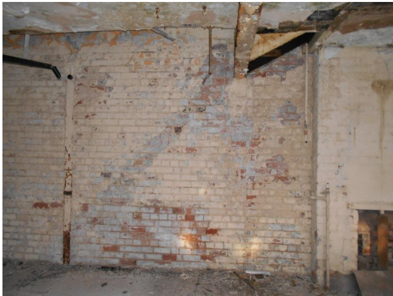
Fig 108: The scar of the former staircase, lost from the north wall of room EF32 up to the second floor
