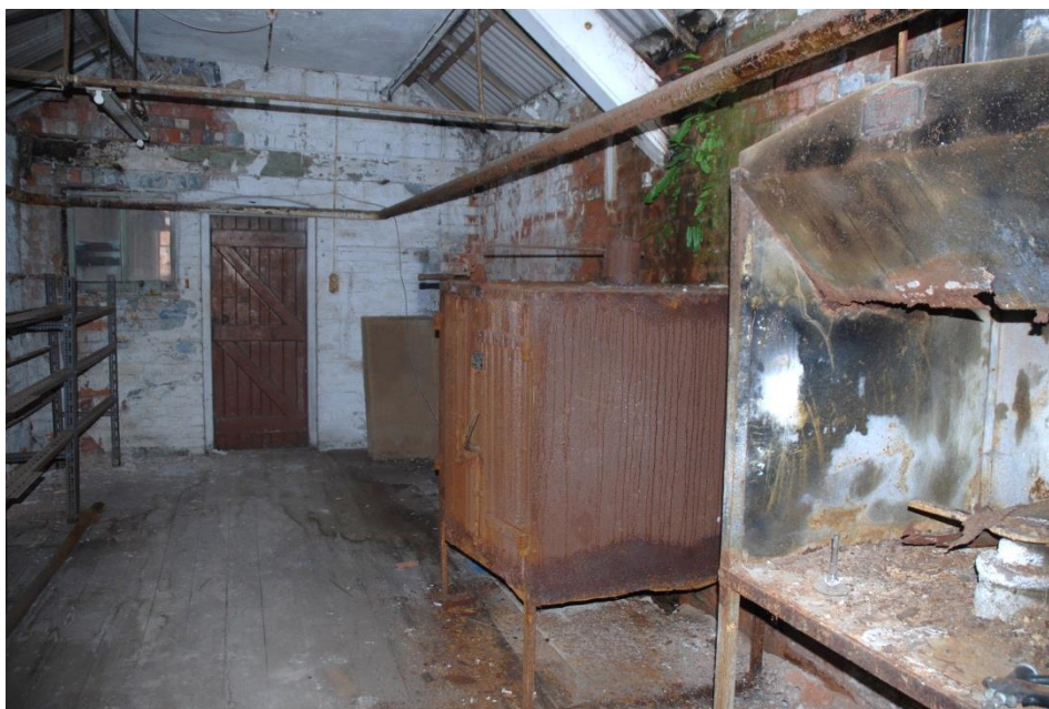
Fig 70: Kiln room EF36, possibly for enamelling (centre) and lacquering (right). The doorway at the end connects directly into EF37 and is secondary.
