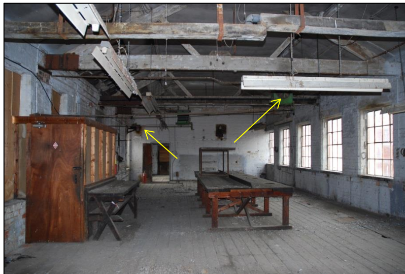
Fig 45: Room ES27, looking north, with boxed-in stair to left. At this level all the windows are square-headed to both front and rear, unlike the arched examples further down the building. The queen-post trusses of the frontage roof are exposed and there is evidence in a number of fitch-plates that the roof trusses have previously had to be extensively-repaired. A variety of side and centre-line benches and work-stations may be inferred from wear patterns on the floor. Any early lighting has been lost to post-war strip lights. Tannoy-type speakers are arrowed.
