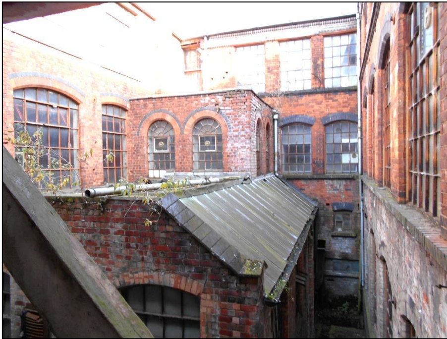
Fig 75: Another view of the polishing shop with its peculiar roofline. Note the truncated parapets surmounting the gable, which possibly indicate a former ridge and fully pitched roof.
