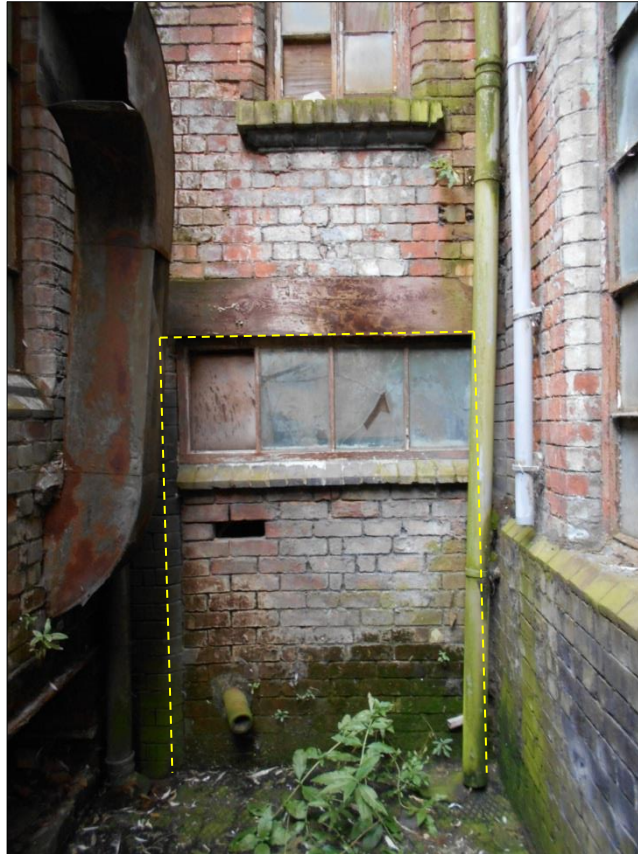
Fig 34: The former main corridor entrance from Vittoria Street to the rear yard and workshops (marked yellow). The small window above once lit a stair quarter-landing
