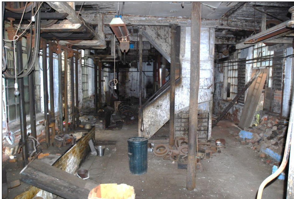
Fig 46: View of EG49, from EG30, looking west. Along both sides lay the brick and concrete benches on which stood the presses, and of which a battery still survives. Heated channels in the floor were intended to provide the working position for the press-setter and operators, while drive was provided through the shafts and belt-driven wheels mounted on substantial timber cradles suspended from the ceiling. The central stair runs up through the whole building.
