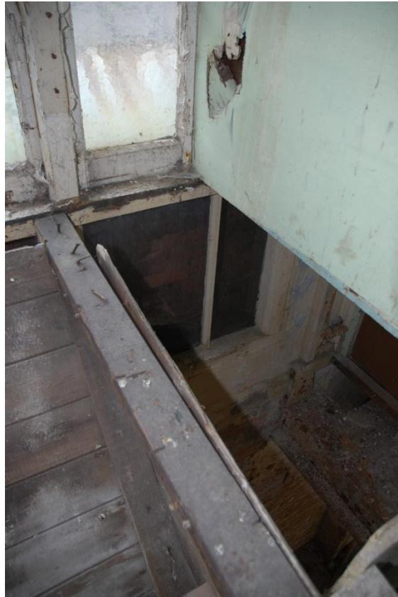
Fig 111: The truncated end of the stair up from the First Floor where it emerges in ES14. Note the lower portion of the huge window, which sits behind the angled protective boards.
