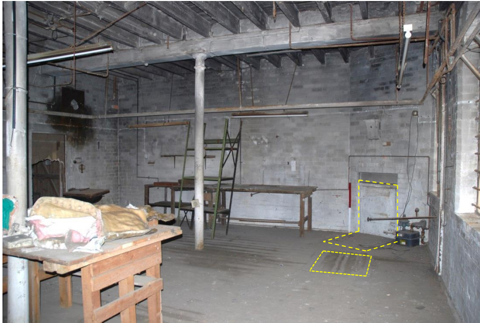
Fig 36: Room EG40, possibly formerly dispatch but built in 1897 as a 'New Stock Shop'. View north from in front of the pavement loading doors, looking north; scale 1m. Note the low-level doorway and hatch to the basement stairs; a second, vertical hatch lies nearby.
