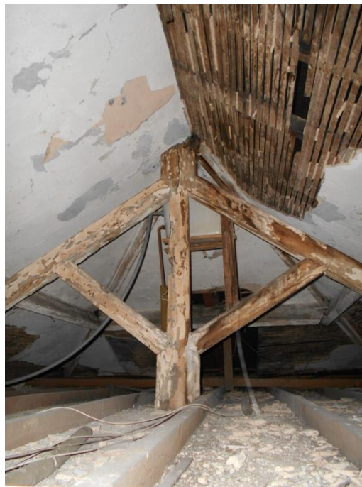
Fig 103: The roof space and truss structure above ES09. A plastered pitch and underside to the rafters show that the present second floor ceiling is an afterthought.
