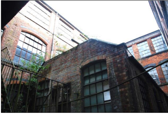
Fig 26: View up over the Polishing shop to the exterior of EF59 and ES39 (top left)
