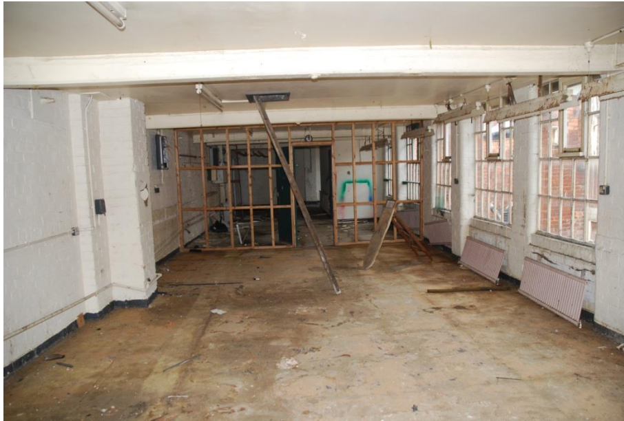
Fig 102: Room ES09 looking west into ES10. The roof is glimpsed through the ceiling hatch (note ladder for location).
