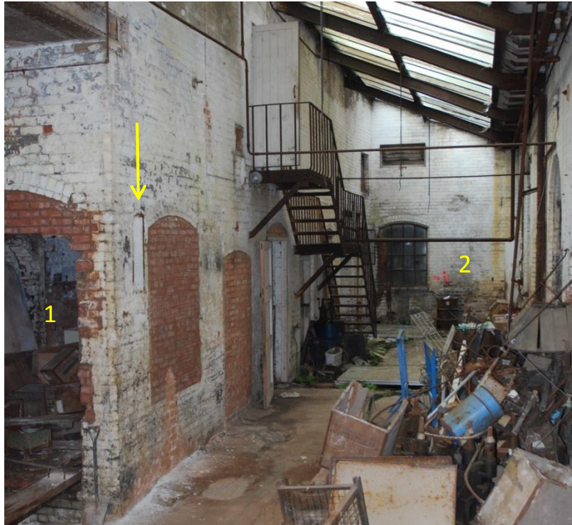
Fig 72: Two boiler houses and engine locations (steam to left (1), gas (2) at the end). Note the large drive-belt slot (arrowed).
