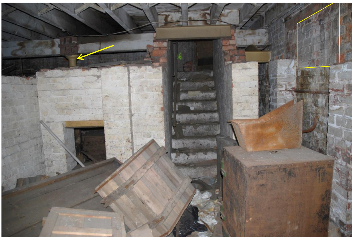
Fig 23: Basement view, looking north in room EB16, with blocked basement light (yellow) on right, with lintel in situ . Note the original ground floor timbers supported on a cast-iron column (arrowed) and almost hidden behind the extensive whitewashed (probably 1940s) Fletton inserts (see below)
