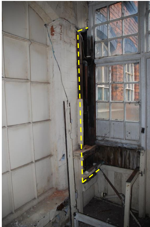
Fig 109: View from EF33. Note the loss of 1¼ rear-facing windows. An earlier range clearly left this as courtyard, as the block-plan of 1896 shows.
