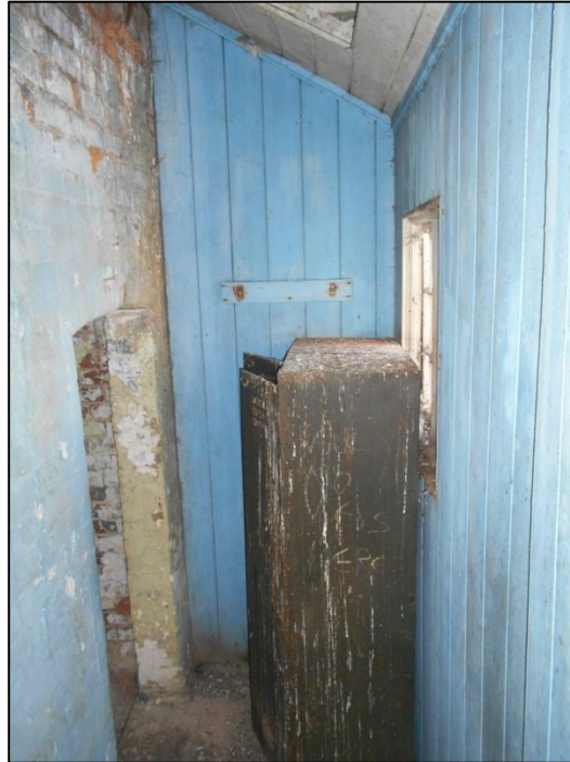
Fig 68: The interior of the dead end passageway in timber (ES36), looking west. It was constructed after the loss of the second floor at the rear, since it remained the only way to access the toilet block (ES35) at this level.
