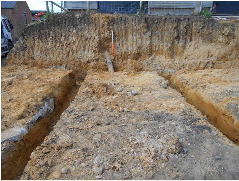
Fig 3: View looking west, showing the extent to which the natural land surface had been previously reduced by over a metre to create the concrete slurry yard; Scale 1m
