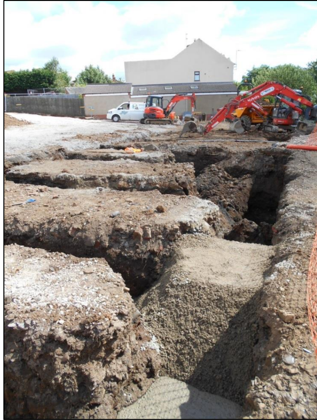
Fig 10: A break in foundation-digging on Units 5-11 (some concreting also), looking east; note the trench collapse in the middle ground on the site of the Victorian well
