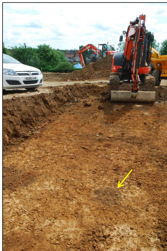
Fig 3: Stripping the northernmost swathe for Units 1-4, looking south. A post-hole is showing up (arrowed).
