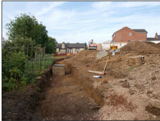
Fig 12: Digging the gabion wall trench, looking west; this view shows the upper factory level, almost as high as a bungalow beyond and the unmodified slope of the garden
