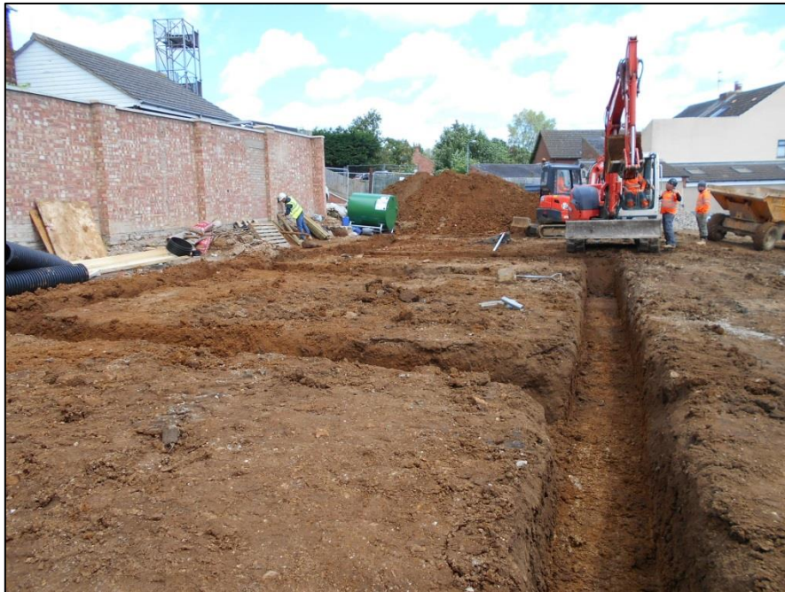
Fig 7: Units 1-4, foundation-digging after stripping, looking east. To the left was the swathe where all the early features were previously exposed and recorded.
