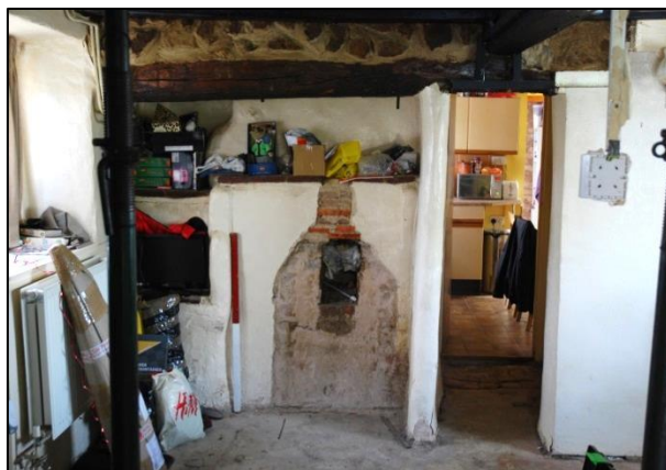
Fig 9: Former inglenook in G1, narrowed for access through on right; Scale 1m
