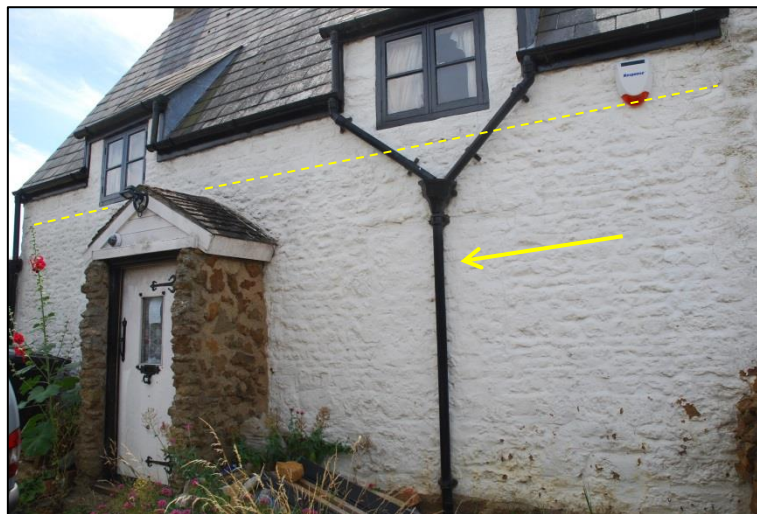
Fig 5: The north-east facing long axis. Note the blocked window beneath a timber lintel. A dashed line shows where the roof has been raised to create the first floor.
