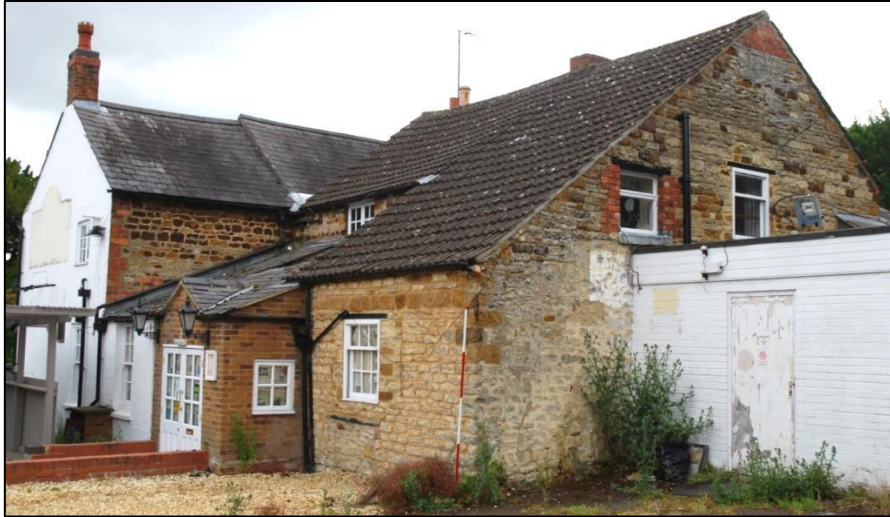
Fig 7: The northern side and rear of the pub; scale 2m. Note the modern brick porch. The blocked cellar light can be seen (but see below for detail).
