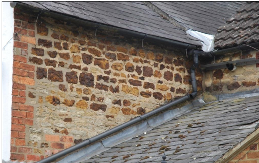
Fig 8: Stonework changes on the rear of the front wing, showing where the roof of the extension was heightened to create a first floor (F2). Stonework of the rear wing too shows differences and a butt joint. Note the independence of the two main roofs.
