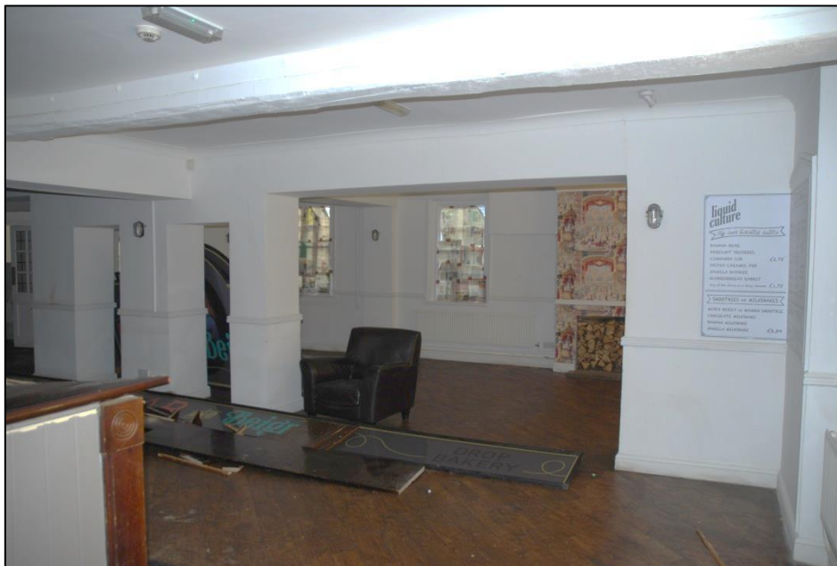
Fig 12: View looking north across G1, fully opened out. Note the former axial beam above. To left, the original rear wall has been all but totally removed, leaving just an RSJ to support the fabric above.
