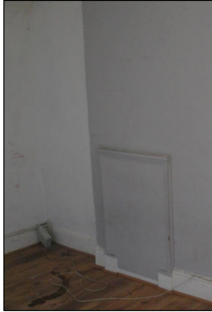
Fig 19: Blocked fireplace in F4. The chimney on the end of the gable has been previously removed.
