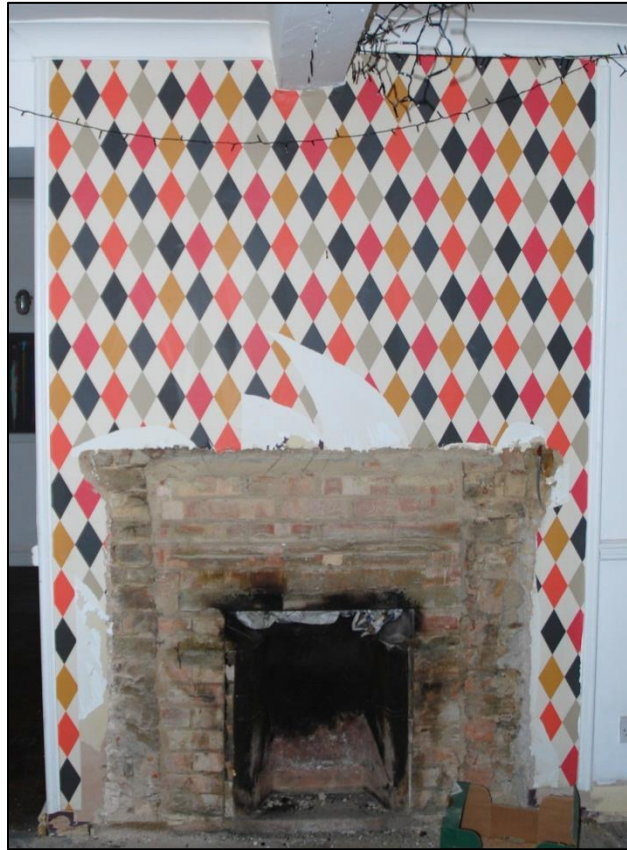
Fig 13: Former fireplace in the west gable of the old rear service wing (G2). The fireplace had been successively reduced during the 20 th century, blocked with Fletton bricks
