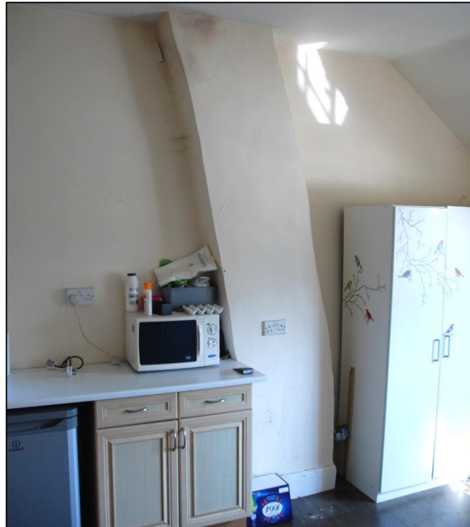
Fig 17: Secondary brick chimney added to the interior of F2. This served an added fireplace at the north end of G1.
