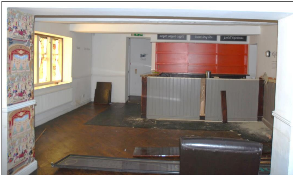
Fig 11: View looking south along G1 to the food counter, the former inglenook, marked by an RSJ above. To extreme left and right in this view are the truncated ends of the original first (north) gable.
