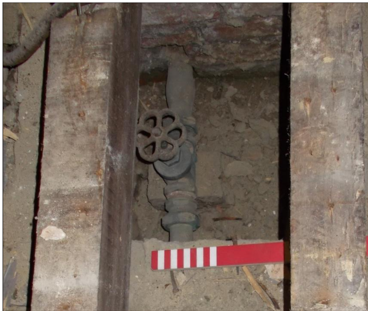
Fig 12: The water pipe and tap beneath the timber floor of Room B7. Scale with 1cm divisions.
