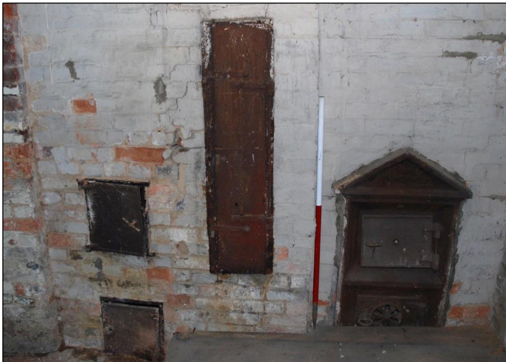
Fig 18: The hot-air firebox and flue boxes in the so-called 'Brush Room' (B17). The iron pediment on the firebox on the right is cast with the name in relief 'G & F Haden, Trowbridge', a 19 th -century supplier of heating to country houses and large institutions. Scale 1m.
