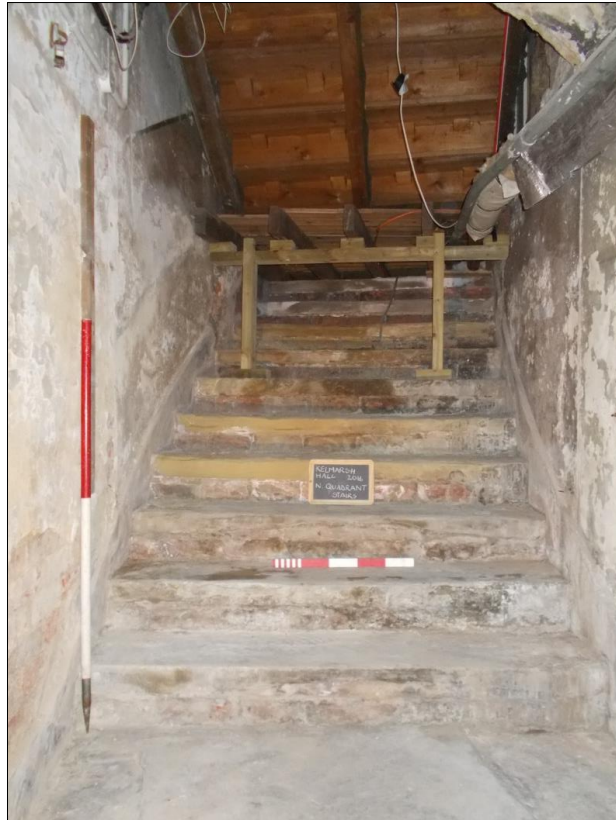
Fig 6: The stone and timber steps in the north quadrant, looking north; 1m and 50cm scales.
