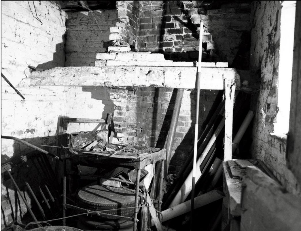
Fig 39: View through the stable door into the clutter of the abandoned forge. To the rear is the part-collapsed brick smoke-canopy and timber bressumer beam; scale 2m.
