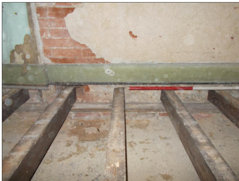
Fig 11: The supporting single brick sleeper-wall capped with a single floorboard supporting the joists, looking south; scale 1m.
