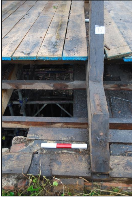
Fig 23: The two wall-plates. Outer one for the roof, inner one to fix the ceiling frame. Between them the brick of the wall top with the scale resting on it. This view shows a mistakenly-cut lap-dovetail adjacent to that actually used to grip the tie-beam of the truss. Scale 30cm
