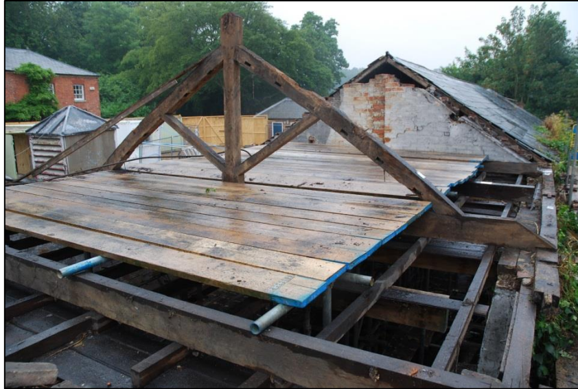
Fig 22: The roof of the ironing room, stripped down to its principal truss. Note at far right the sections of wall-plate falling away from the wall-line. Also the ceiling-frame inside the wall-lines.
