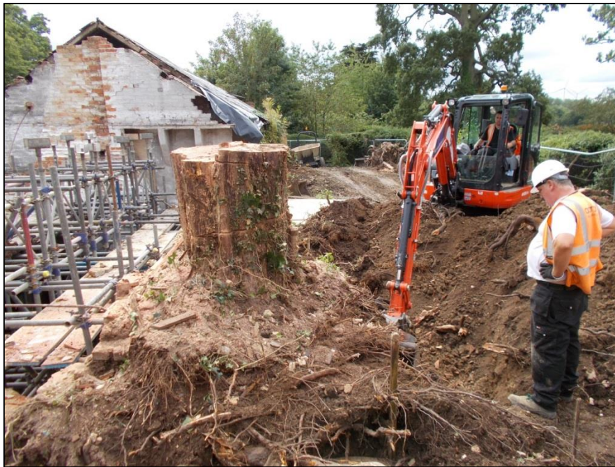
Fig 21: Digging out one of the pine tree stumps from against the still-scaffolded ironing room. Note the steam collector high on the gable behind.
