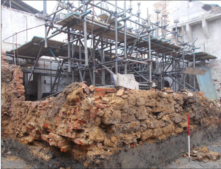
Fig 26: The below-ground stone and brick north and west walls of the ironing room reduced, looking south-east. Note the high-level steam-collector (top right). 1m scale.
