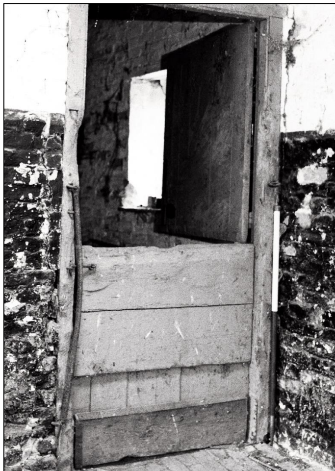
Fig 38: The stable door between stable and forge. Note the hinged iron bar to left, iron strap at lower right, and the excessively chewed exposed edges of the timber; scale 1m
