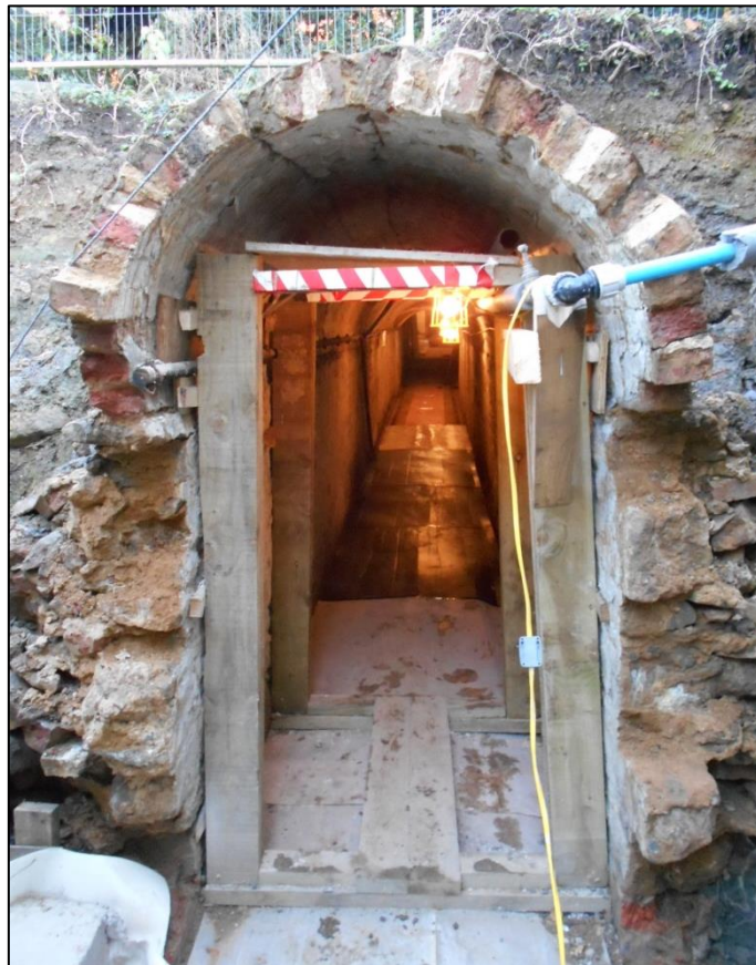
Fig 31: The tunnel, during conservation at its broken end. Note its shallow burial at its apex.
