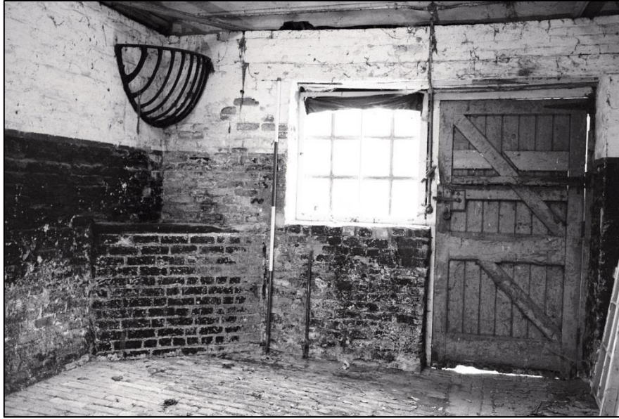
Fig 35: The front of the stable, with two part door, added brick corner trough and iron hay-basket; scale 2m
