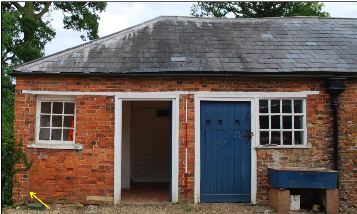
Fig 32: WC to left, stable to right. Note the continuous (flimsy) wall-plate and the butt joint (arrowed) showing how the front of the WC wall is an insert to block a previously open front; scale 2m
