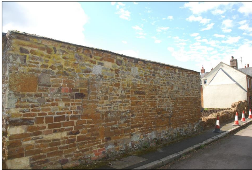
Fig 6: Adjacent garages with former cottage front wall with blocked doorway and window. These are being reused in the new development
