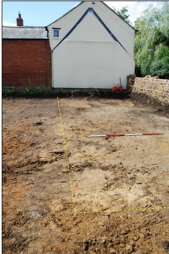
Fig 8: Looking west to the preserved former gable. The former cottage footprint is outlined; scale 2m
