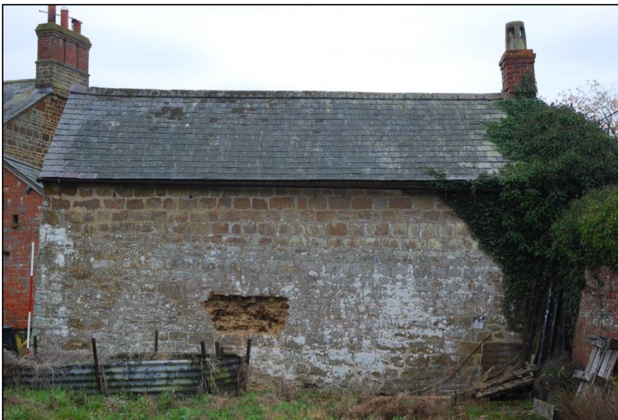
Fig 5: The rear face of the chapel (scale 2m). Note the change in coursing two thirds of the way up.
