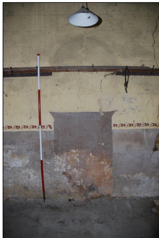
Fig 10: Marks indicating the former presence of a lectern or tabernacle against the south wall (scale 2m). Later the space was infilled with a modification to the coat rail.
