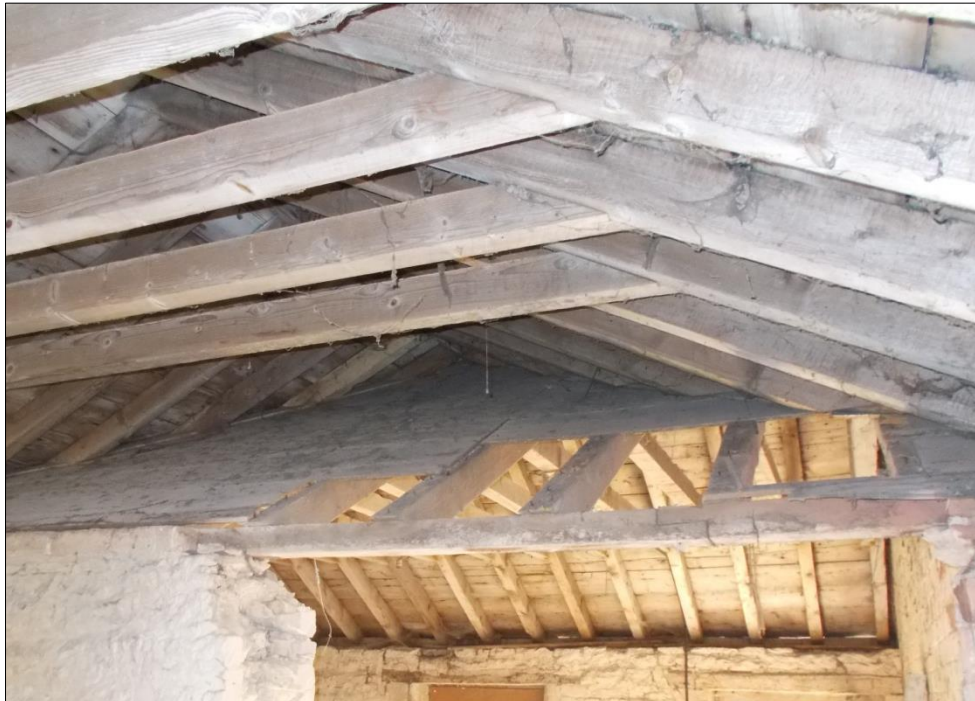
Fig 7: The north roof slope of Barn 2 covered with sarking boards, beneath the roof of Barn 3, looking south.
