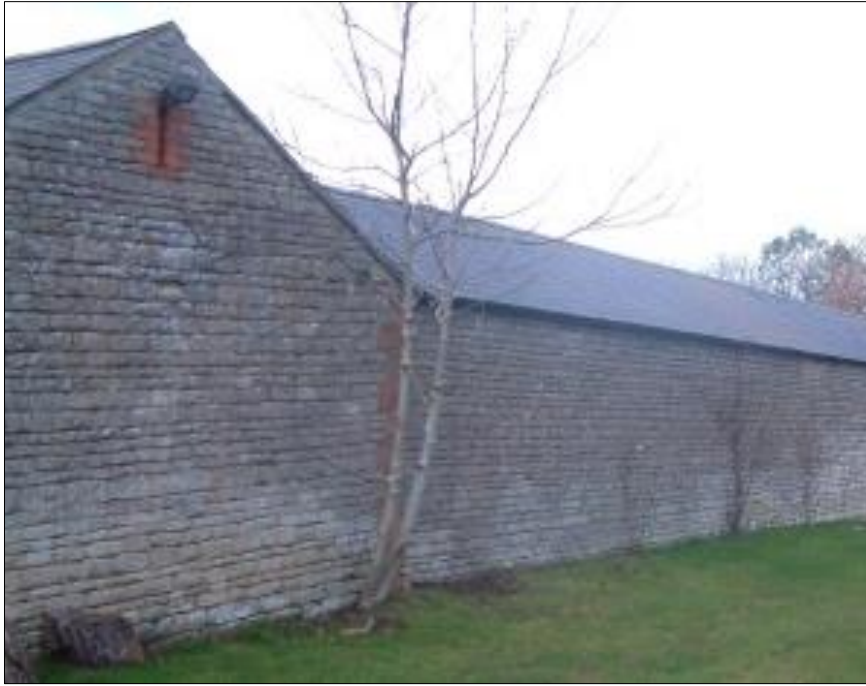
Fig 10: The east gable of Barn 2 (left) and elevation of Barn 3 (right) showing disparate levels of stone courses, looking north-west.
