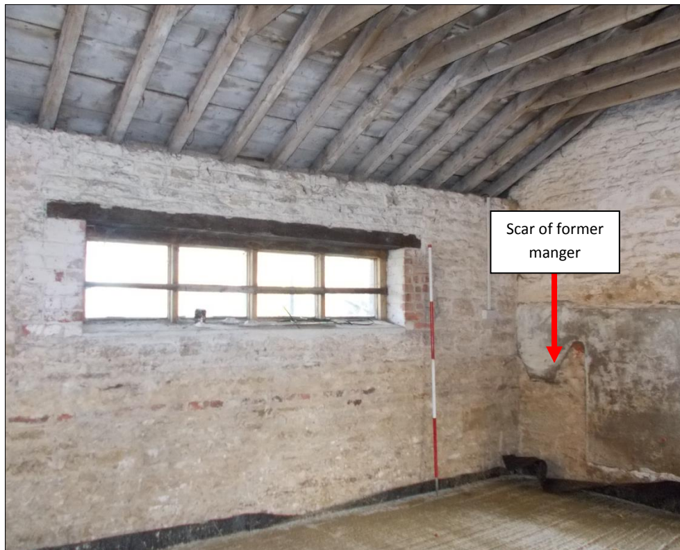
Fig 5: Barn 1, the inserted east window of the north wall, looking north-east. 2m scale.
