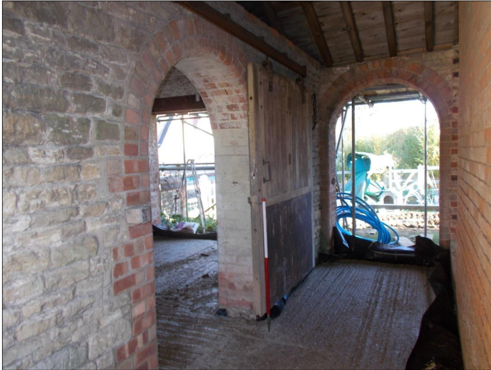
Fig 6: The sliding door closing the arched door from Barn 1 (left) into the corridor (right), looking north-east; 1m scale.
