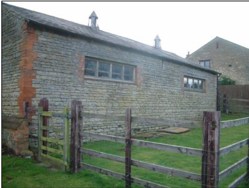
Fig 4: The north elevation of Barn 1 showing brick quoin dressings at corner and inserted window openings, looking south-west.
