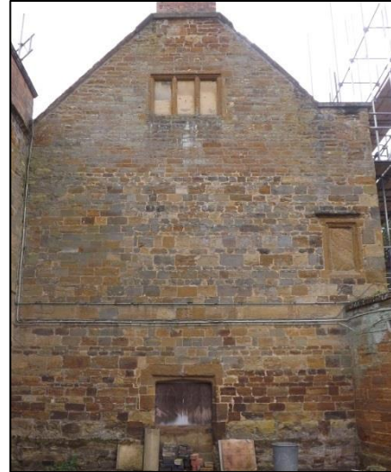
Fig 50: East end of the north range. Note at right the small blocked window which once opened into F10 next to the fireplace
