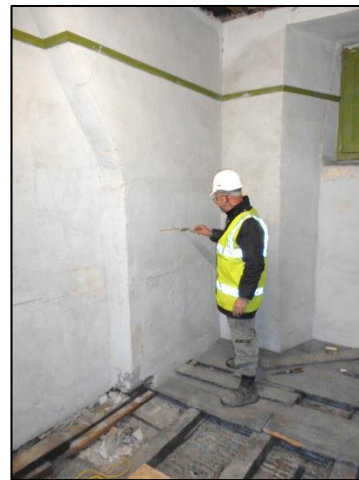
Fig 48: Room F9, discovering a hidden fireplace in the south east corner of the room; note the angled flue to top left
