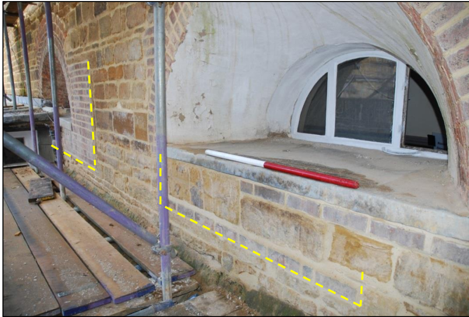
Fig 58: Two courtyard-facing lunettes replaced earlier stone-mullioned windows (dashed), view looking north-east; Scale 1m
