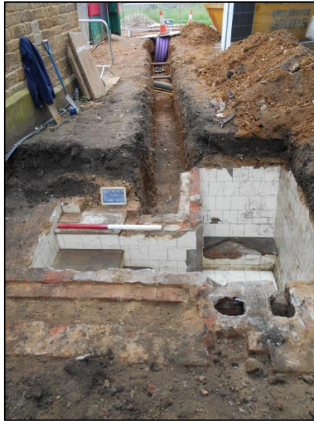
Fig 6: Typical monitoring conditions outside the north range - on this occasion the conduit trench which discovered the Victorian plunge bath
