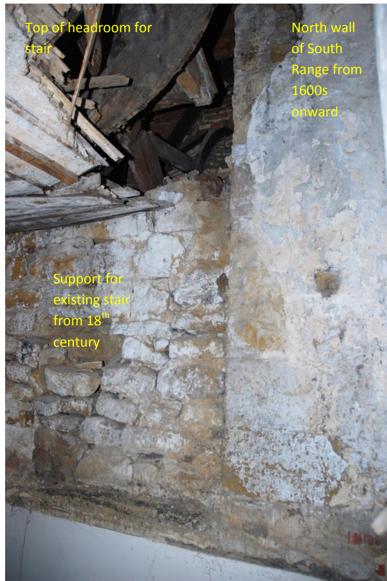
Fig 75: Phases present in G14; note the vertical butt-joint and the curved wooden former creating half an ogee
