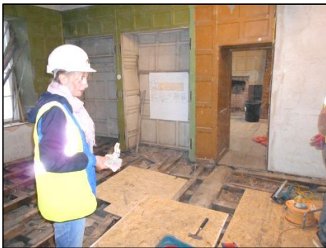
Fig 47: Room F9 looking east into F10. Note the cobbled-together panelling infilling a former fireplace left of centre
