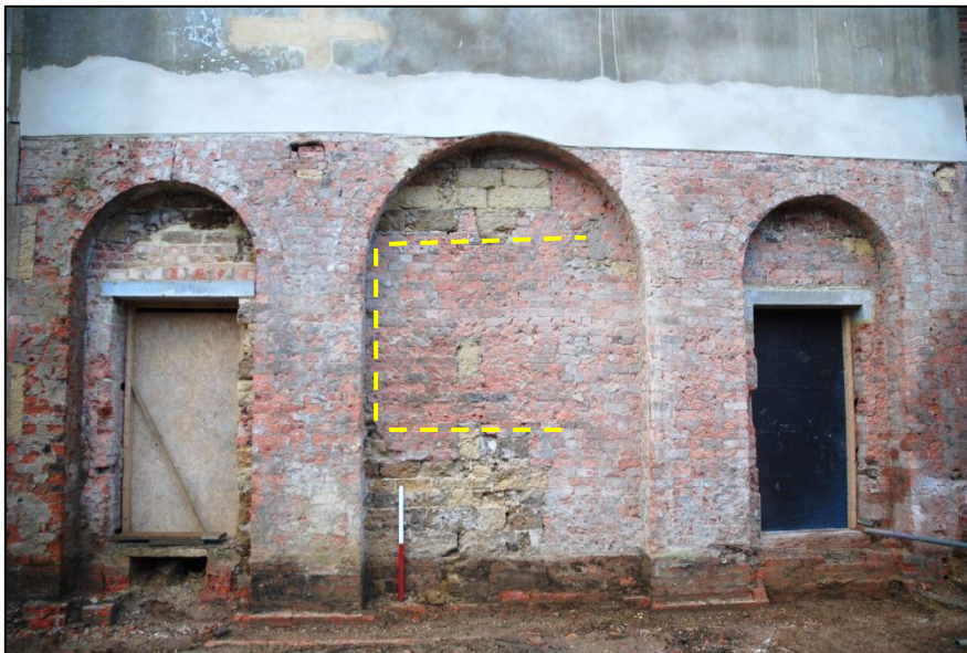
Fig 60: Looking west, applied brick buttressing used to add solidity to the old 17 th -century gable end when it was increased in height in the 18 th century. With 1.6m+ of unstable build-up on this (east) side, and a basement on the far (west) side, stability was paramount. Some remnants of the former stone gable were left where they could be, where build-changes suggest a former window location (dashed); scale 1m.
