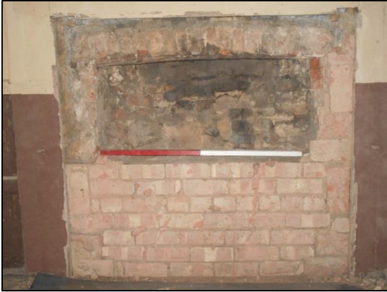
Fig 49: The reduced and blocked 17 th -century fireplace in the east wall of F10; scale 1m
