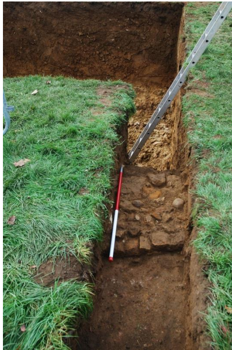
Fig 17: The west wall of the west range, adjacent to the successful 45000L Tank Trench 2 beyond, looking west (Abbey behind camera and slightly to left); scale 1m. The tank trench was c6m x 6m in plan, and 5m deep.
