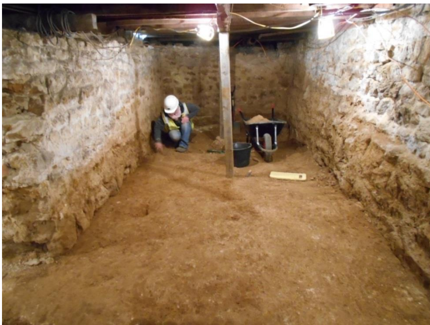
Fig 67: B5 excavated. View looking east within the emptied B5, during cleaning of the natural ground surface; the spine wall, broken through to link B5 and B6, is to the left. This level was then further reduced by a metre to create the new Plant Room. Sand-staining part-way up the walls marks the former height of removed debris.
