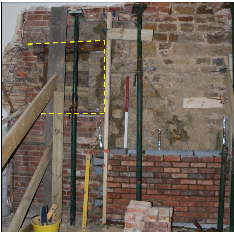
Fig 61: East wall of Room F30, with the old stone fabric and window (yellow) made good in brick with lacing timber courses. Hastily opened up and propped in 2016, the collapsing wall was substantially rebuilt from the inside; scale 1m.
