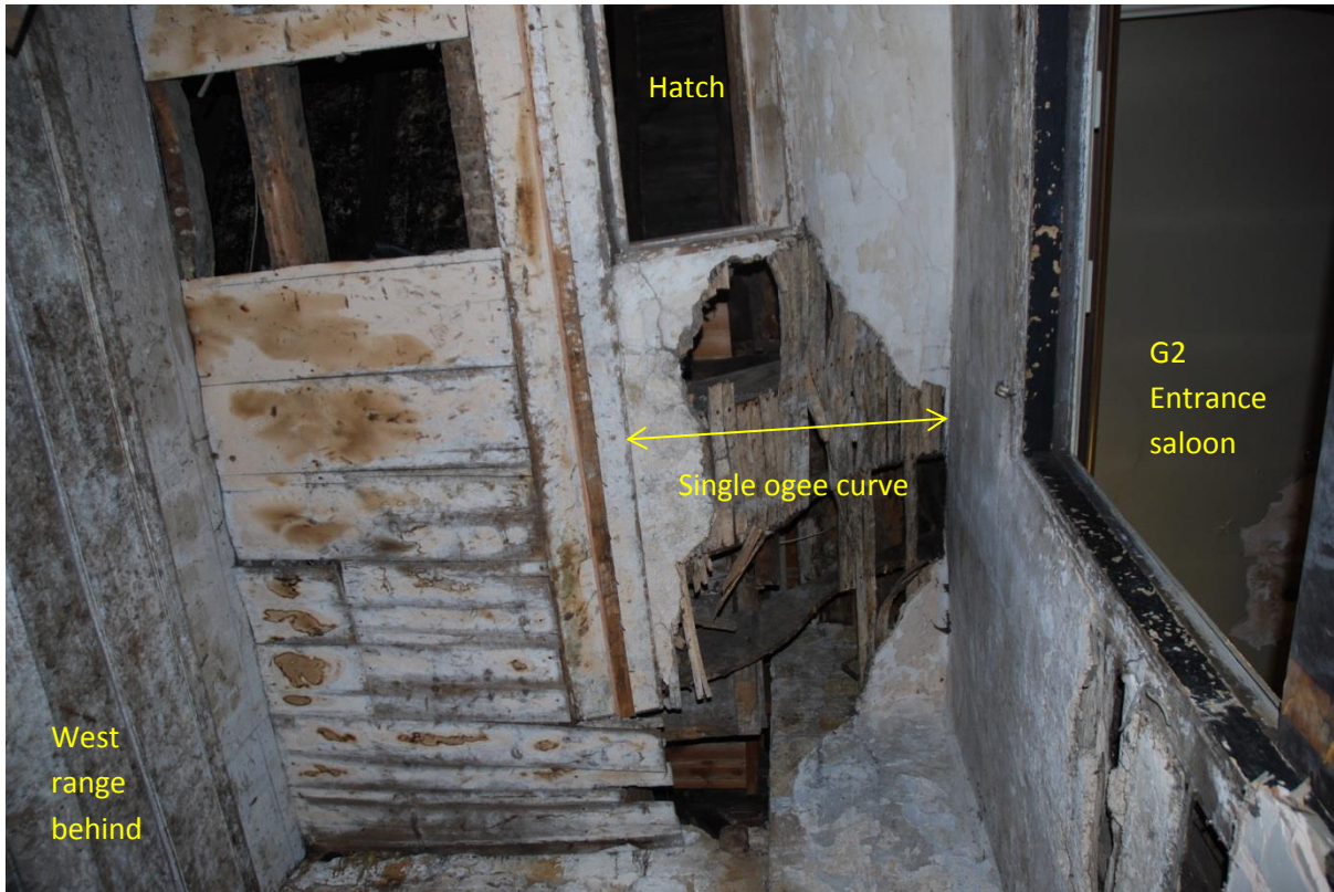
Fig 74: View directly up within G14, showing the underside of the former grand stair into the 1750s South Range when built.
