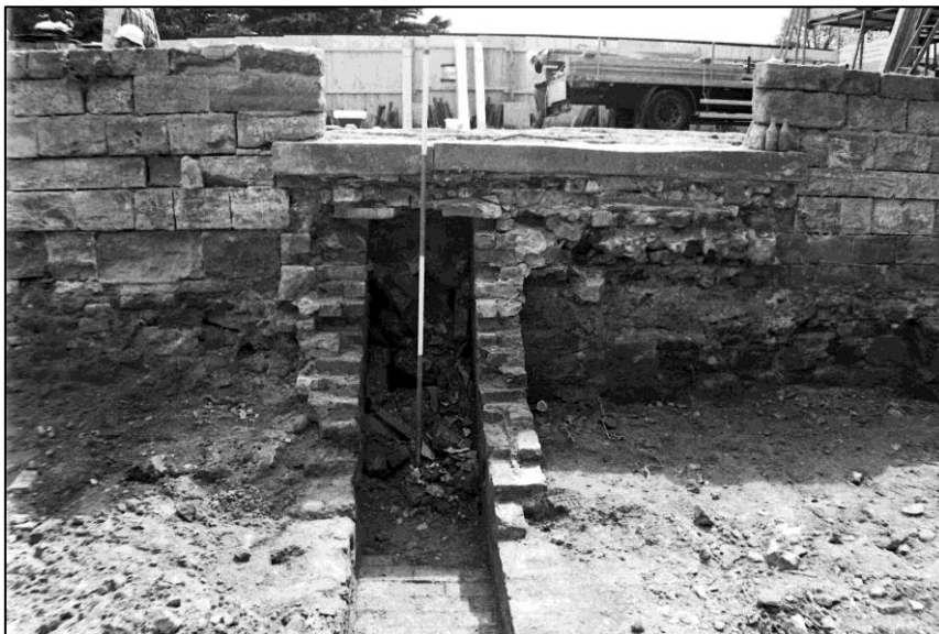
Fig 22: View south from the boiler pit along the heating channel which fed the former Conservatory with hot water. The base of the channel was 1.6m below the conservatory floor. This view is directly south from the inspection chamber adjacent to the boiler pit. Following the loss of the conservatory, the whole was later truncated by a set of steps (and that incremental truncation is visible in the rising brick courses; scale 2m (Scanned from B&W negative in site archive)
