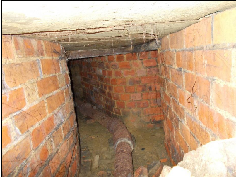
Fig 21: A snatched view along the buried brick culvert from the boiler house to the house, entering under the back door (to G5). This view was only possible by placing head and shoulders in the former maintenance pit.
