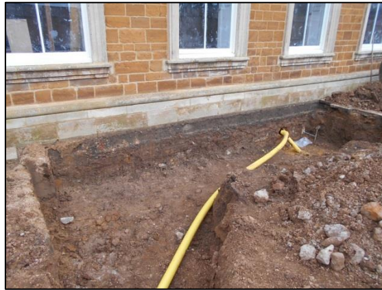
Fig 63: New services entering high in the basement wall of B5. Here Test pit G2 in 2014 noted 18 th century destruction material (17 th century fragments) at 1.2-1.5m below the modern ground surface (Soden 2014). Natural ground is 1.8m below the current ground surface.
