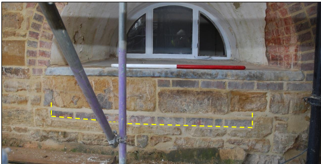
Fig 59: Another, more oblique view of the more southerly of the two lost window locations (dashed), view looking east; scale 1m
