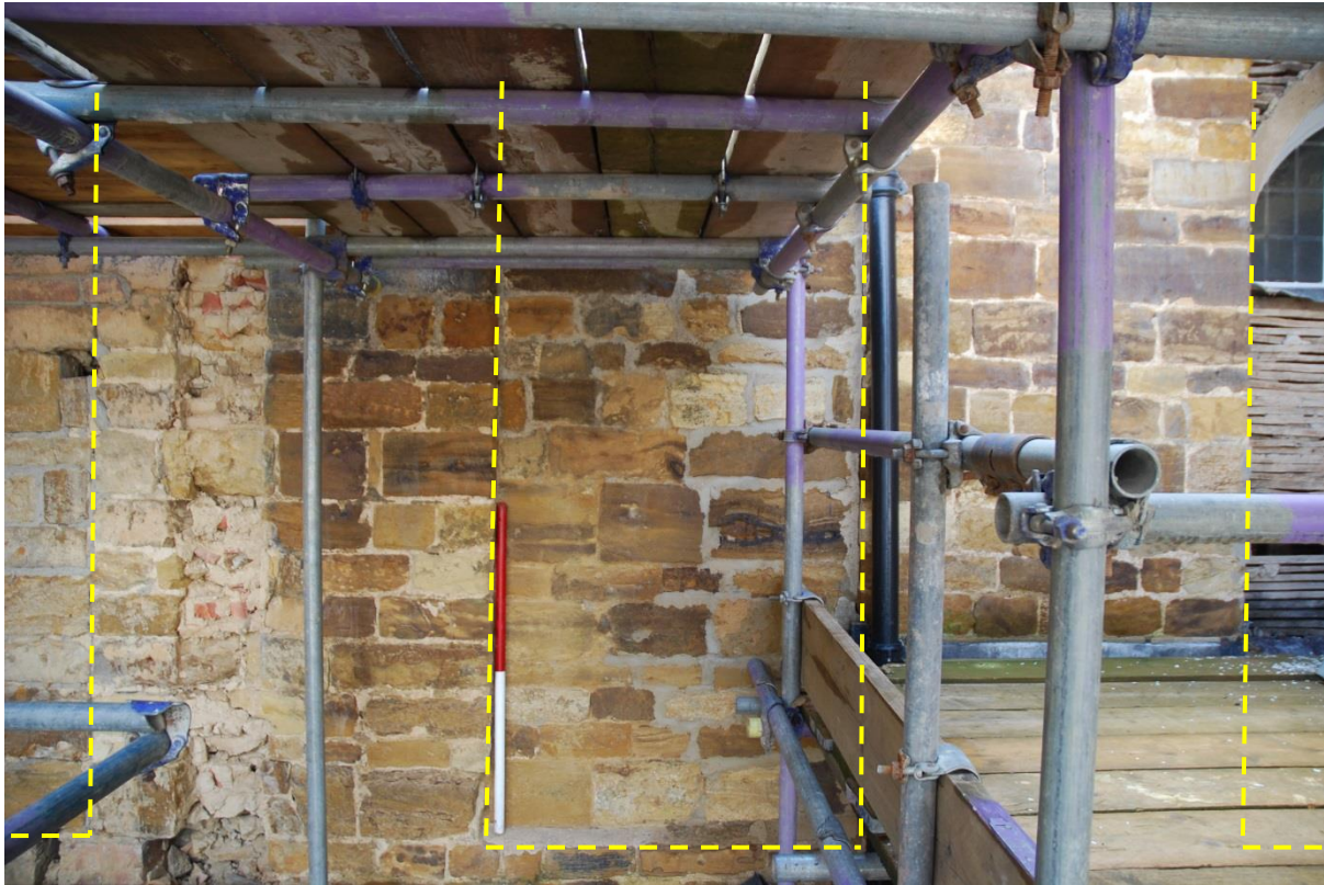
Fig 81: Behind the scaffold cradle lies a row of three former (probably) sash window locations (marked). There is a single replacement lunette (right); scale 1m.
