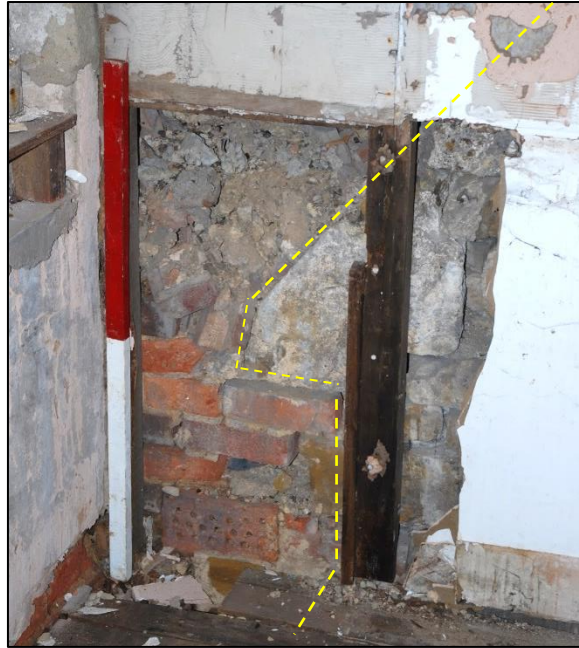
Fig 57: In-situ kneeler low in the east corner of the south wall of room S9; scale 1m. Its presence shows that the original junction of lower (first floor) eaves in the east and south ranges in the early 17 th century onwards must have been configured in a separate gable. The addition of a second floor in brick covered this up.
