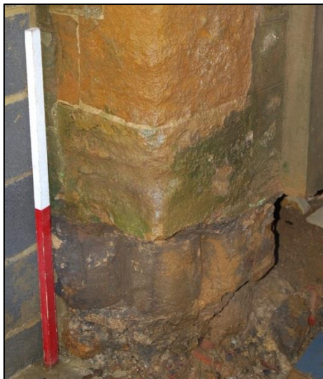
Fig 56: Base of the southern jamb to the eastern doorway, with medieval roll-moulding. This is the best evidence for a late Romanesque/Early English origin. No counterpart survived on the north side; Scale 1m
