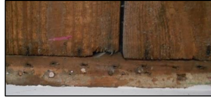
Fig 43: F3 surviving rail/muntin junction
