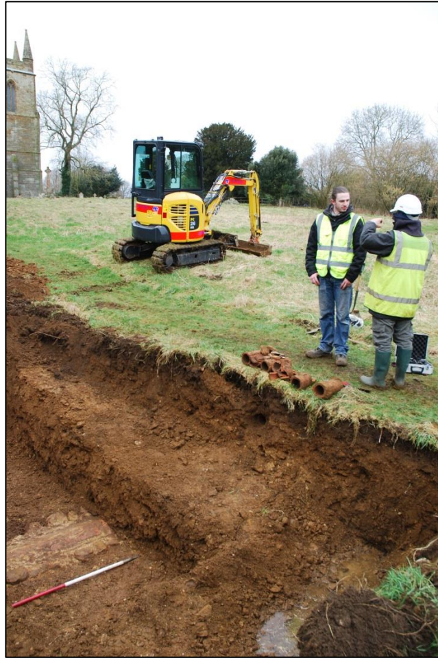
Fig 7: The brick and ironstone culvert, relative to the works, looking north-west; scale 1m
