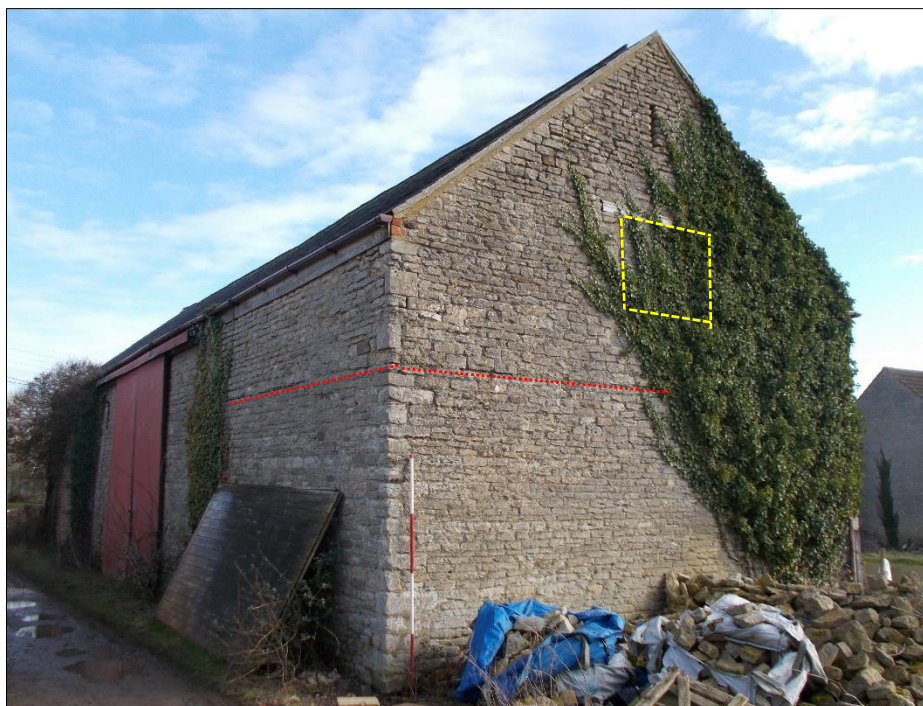
Fig 7: The south gable and west wall, looking north-east. Infilled opening highlighted with yellow dashed lines. Level of iron sheet indicated by red dotted line. 2m scale.
