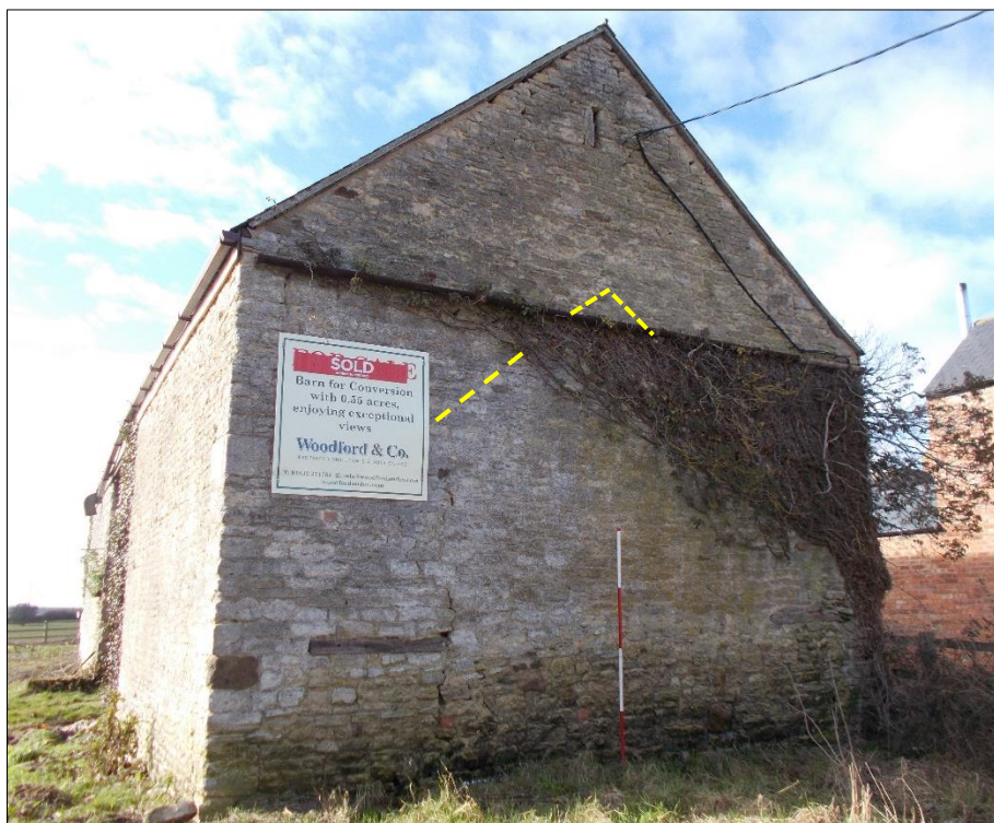
Fig 5: The north gable showing the flaunching scar (dashed yellow line). Looking south. 2m scale.
