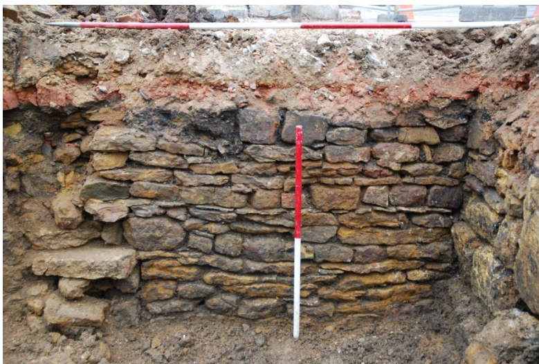
Fig 6: The cellar, looking east along St John's Street. The back (north) wall broken open by insertion and removal of a fuel tank. Scales - 2m horizontal and 1m vertical.
