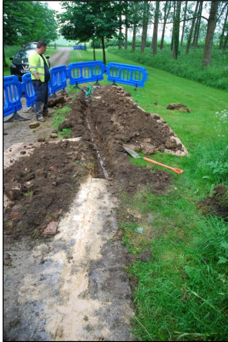
Fig 3: Approaching the bridge from the north, for c10m the new trench shares its line with an existing BT duct. Note the large poplars to the right whose root systems are extensive.
