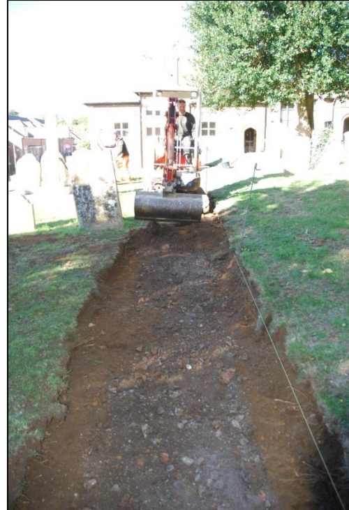
Fig 5: The final machining to a depth of about 250mm. Note the clinker sub-base of the old path down the centre
