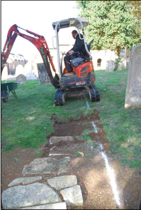
Fig 4: Removing the turf; note the re-used foot-stones being uncovered. At the bottom edge of this view is the top step serving the earlier path
