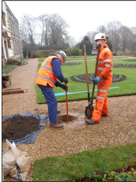
Fig 3: The Window Samples were hand-dug to a depth of 1.2m. Here WS2 is shown.
