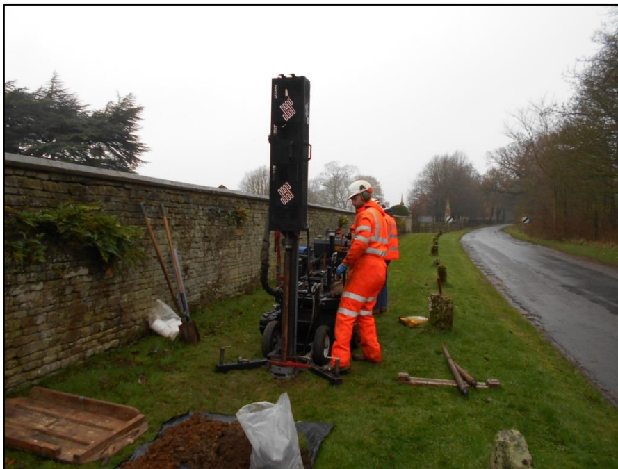
Fig 4: Mechanical coring of the Window samples, the core retained in a removeable plastic sleeve from 1.2m downwards. Here WS1 is shown.
