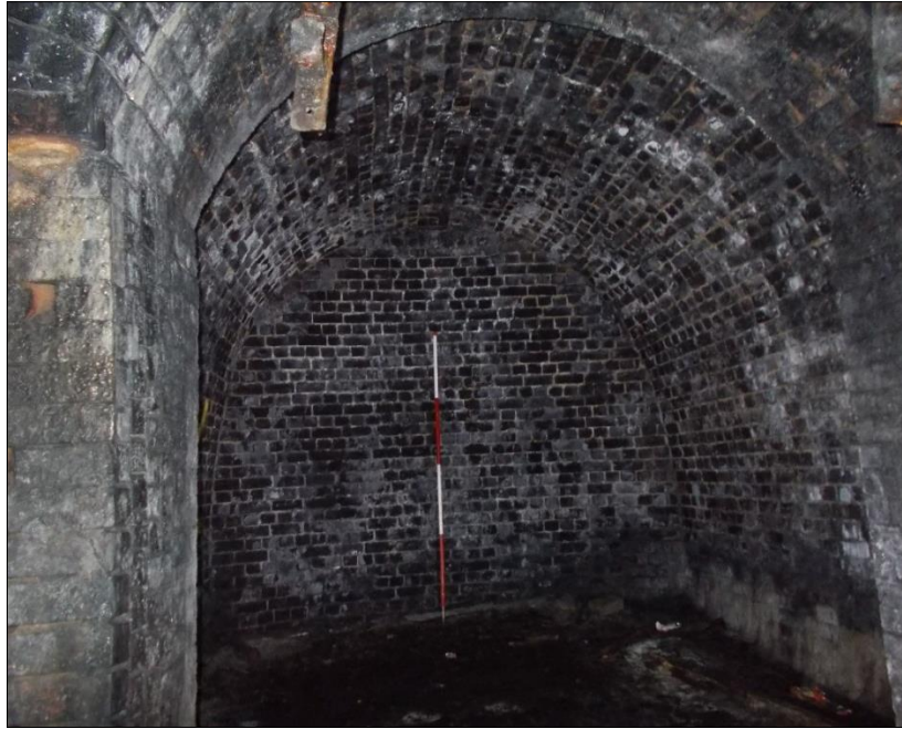
Fig 9: One of the three rest cabins on the east (Up) side of the tunnel, looking east. Here the thickness of the tunnel brickwork can be gauged. 2m scale.
