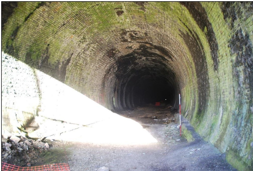
Fig 7: View along the tunnel from the southern, Charwelton end; 2m scale. A miniscule pinprick of light marks the opposite end, 3000 yards away.
