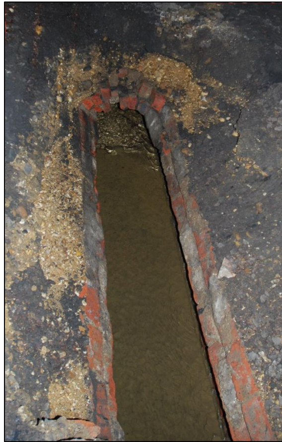
Fig 5: a short section of the tubular brick drainage culvert exposed, its vault opened for inspection
