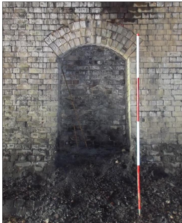
Fig 8: One of the arched refuge niches on the west side of the tunnel. Hard-packed gravel is 'splashed' over its base. 2m scale.
