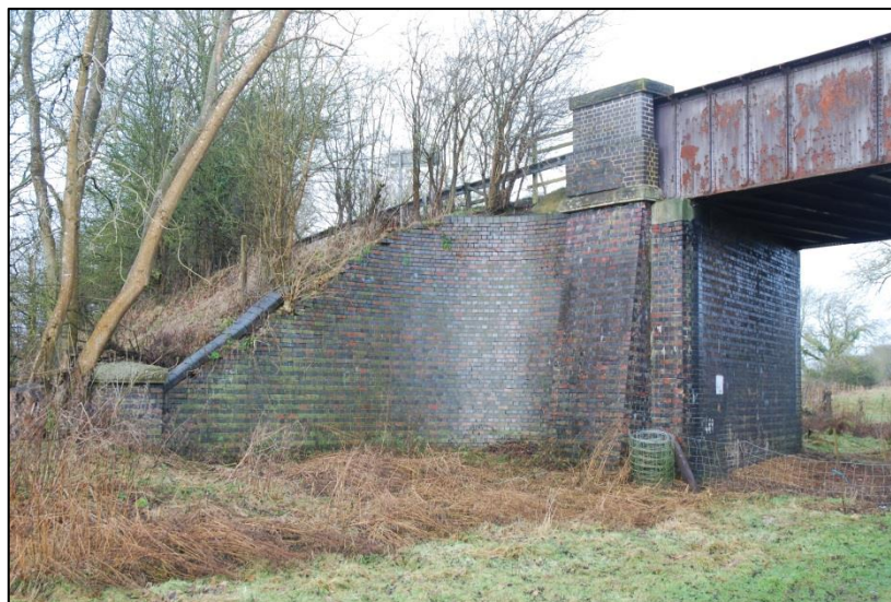
Fig 16: Staffordshire blue engineering brick bridge abutment, looking north-west. Note the principal girder-bearer in stone, matched by the finishing details.
