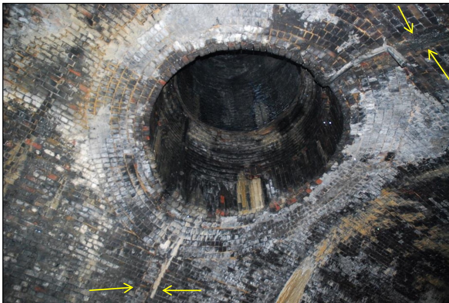
Fig 10: One of the ten-foot wide ventilation shafts; note the elaborate tumbling-in of brickwork to marry up the two different-sized brick cylinders involved. Built-in drainpipes run off each side (arrowed)
