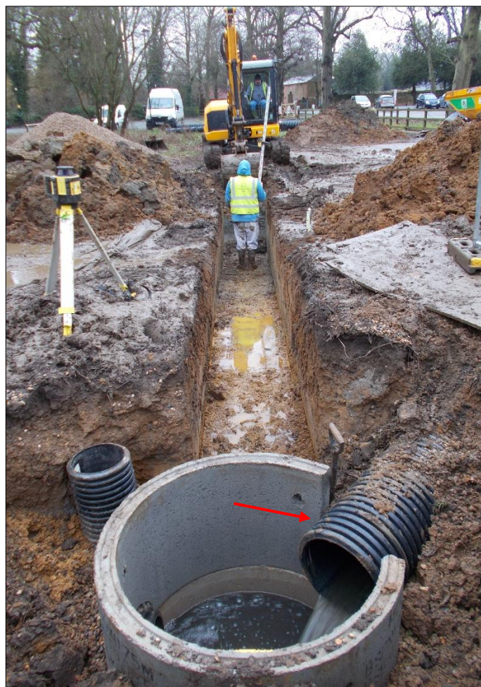
Fig 6: The inspection pit at the south end of the primary north-south new water pipe run, looking east. The short south-east section (arrowed) has been fitted which connects with an existing stone culvert manhole. Looking east.
