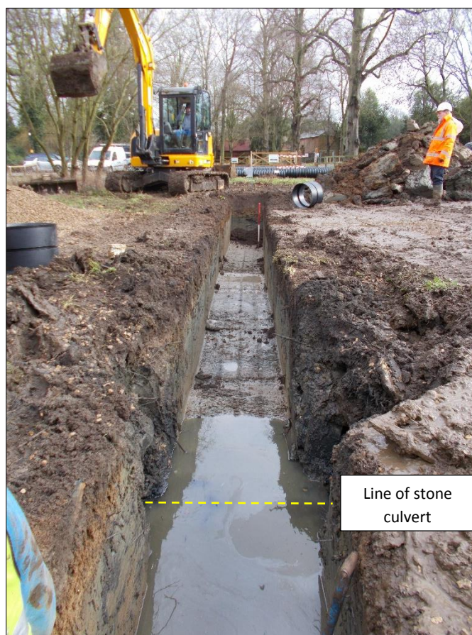
Fig 8: The eastern end of the east-west section of new pipe trench, looking east. 1m scale bar.
