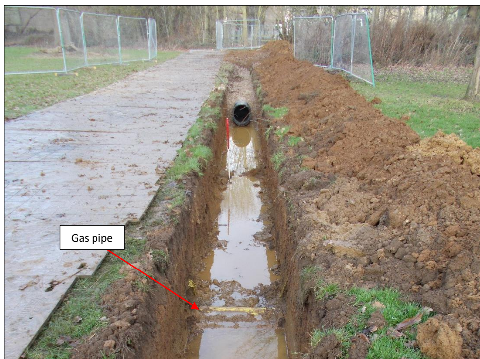
Fig 5: The new trench with installed new water pipe and backfilled section, looking north. 1m scale bar.
