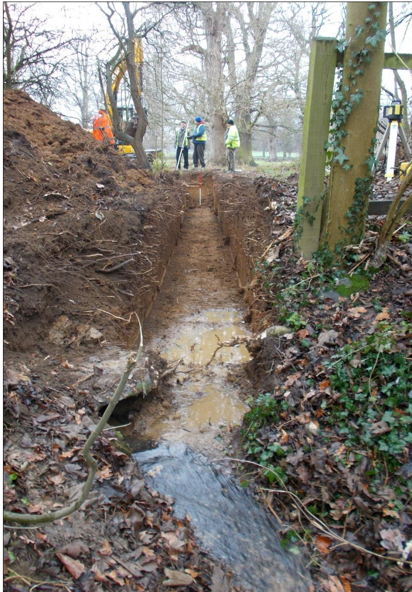
Fig 4: The north end of the new drain run trench (right) and the old stone culvert outlet (left), looking south-west. 1m scale bar.
