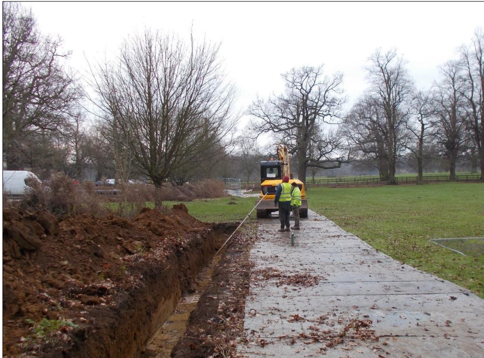
Fig 3: The trenching underway showing the temporary trackway laid to prevent rutting, looking south.
