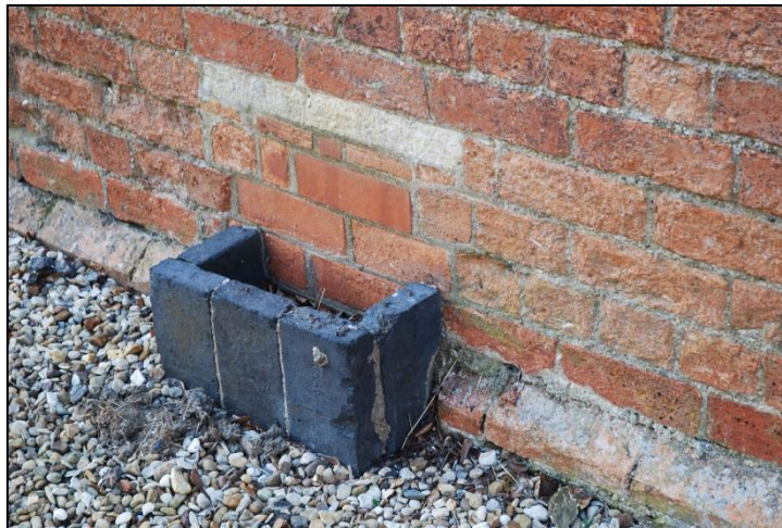
Fig 7: Bricked-up ventilator at ground level (three to each long side), probably reduced in size and efficiency in 1925; Note chamfered brick plinth integral to the chapel
