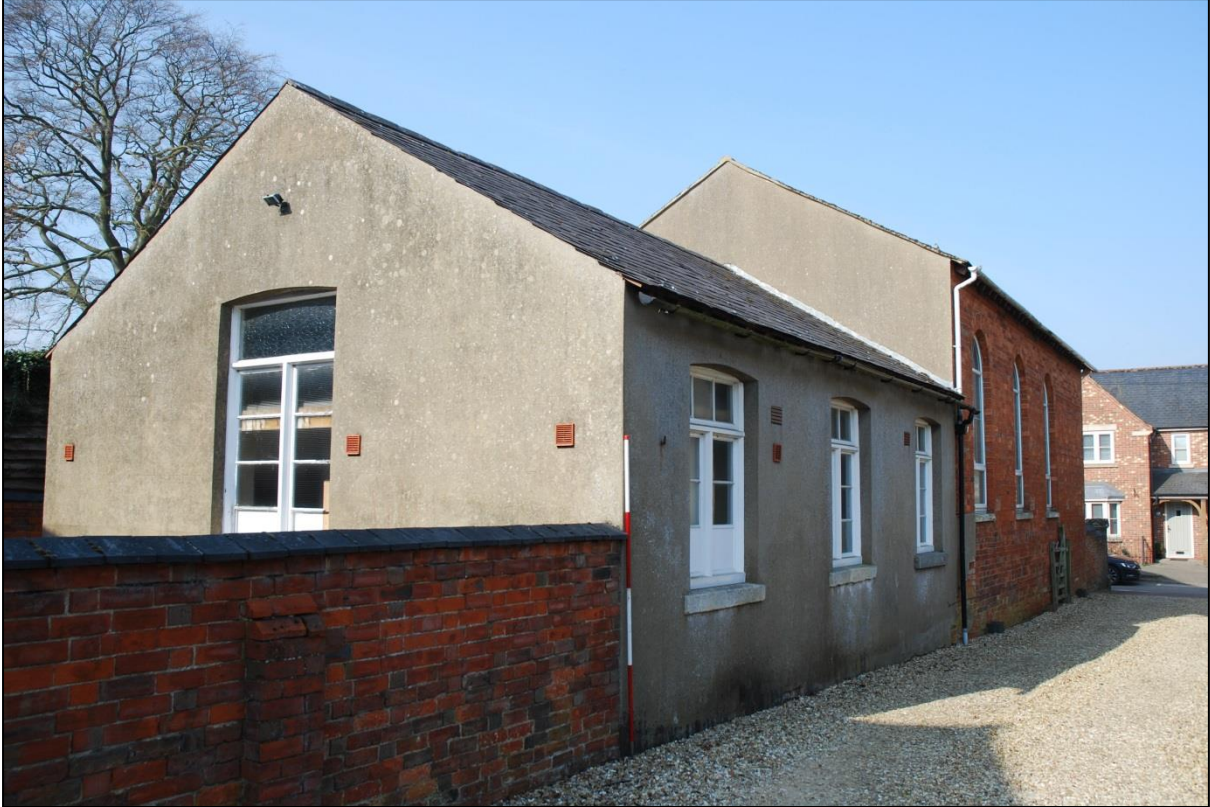
Fig 5: The fully-cement-rendered schoolrooms (foreground) added to the east gable of the chapel; scale 2m
