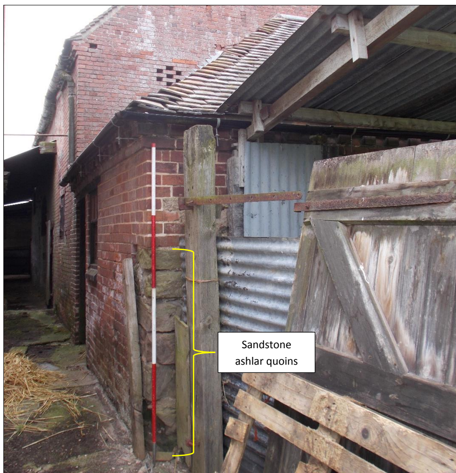
Fig 84: The north end of the cattle stall range, looking south-east. 2m scale rod.
