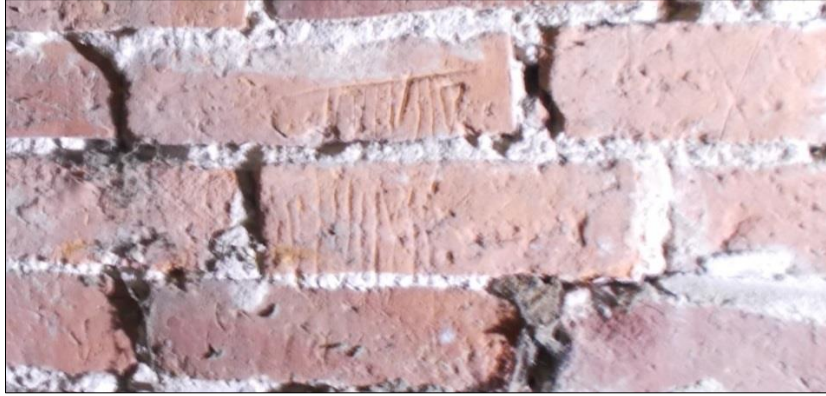
Fig 69: An example of the numerous tally marks inscribed on the brickwork surrounding the central doorway of the store barn.
