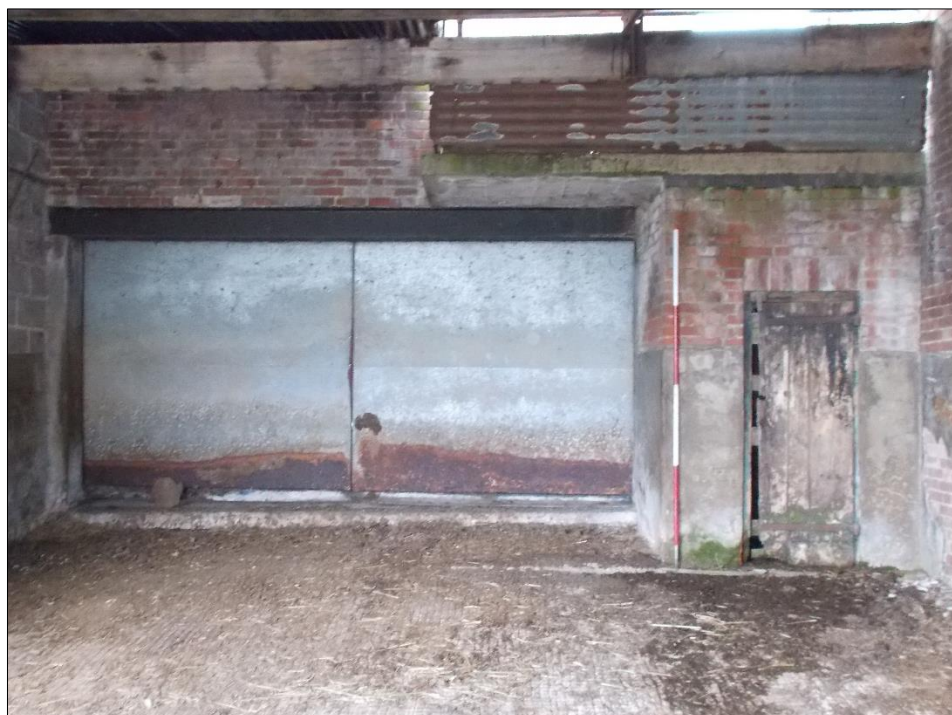
Fig 94: The ground-floor north gable wall of the two-storey dairy showing the inserted double-doors, looking south-west. 2m scale rod.
