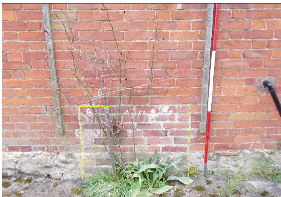
Fig 12: Infilled cellar window in north-west gable wall. Outline indicated in yellow dashes. 2m scale rod.
