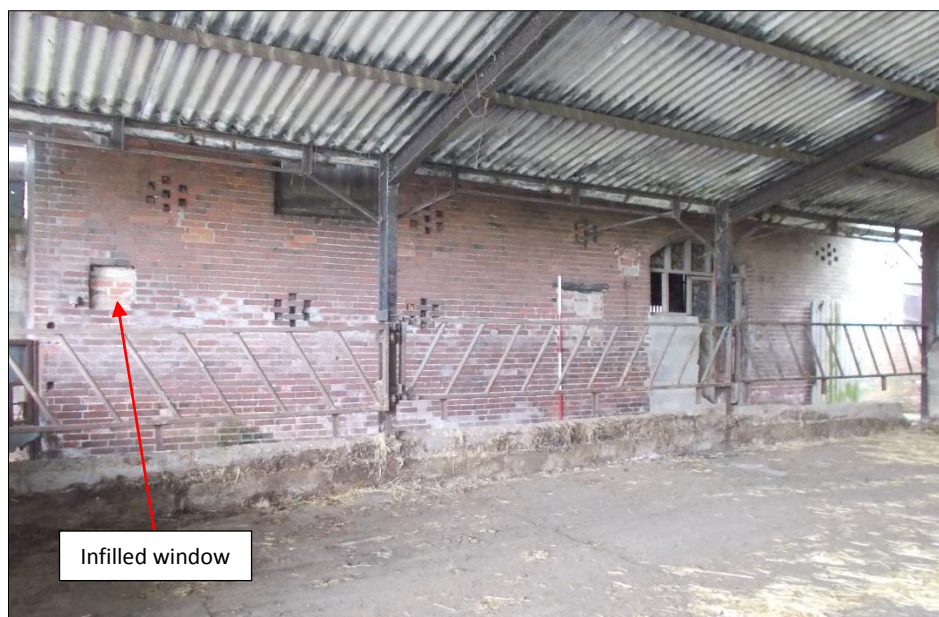
Fig 66: The north-east elevation of the store or threshing barn, looking south-west. 2m scale rod.
