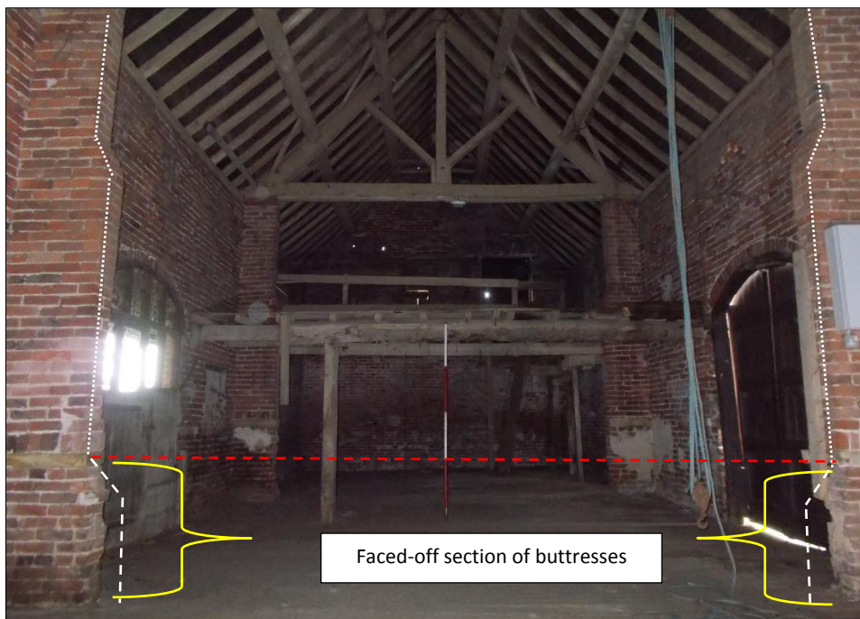
Fig 70: The internal buttresses showing the faced-off lower portions, looking south-east. The white dotted lines show the current raking profiles of the upper sections, the white dashed lines the possible lower profile. The red dashed line shows the possible location of a low (?) dividing wall. 2m scale rod.
