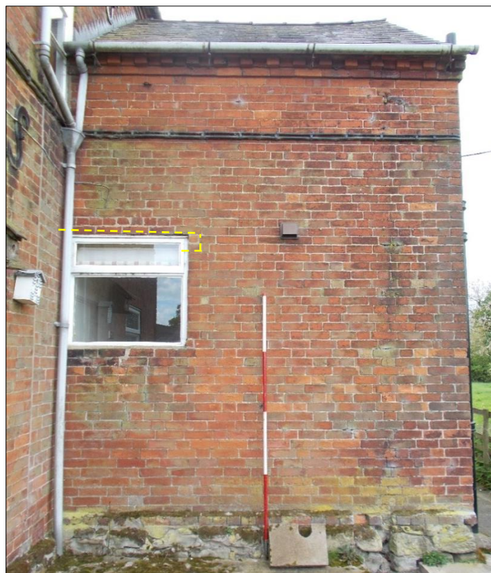
Fig 10: The north-east facing elevation of the rear wing, looking south-west. Probable outline of former timber lintel shown with yellow dashed lines. 2m scale rod
