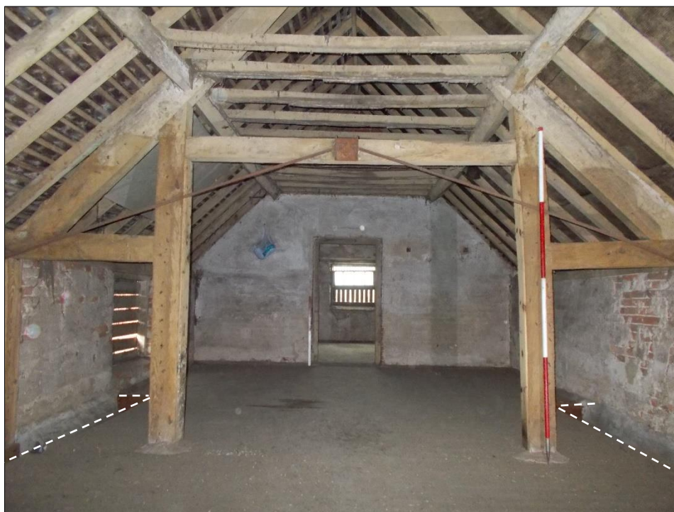
Fig 98: The two-storey dairy range, first-floor room showing the roof truss, looking north-east. White dashed lines show fodder slots. 2m scale rod.
