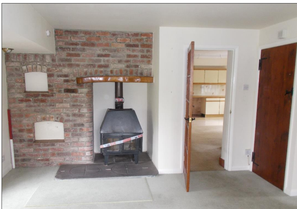
Fig 40: Room G11 looking north-east (room G6 through open door). 1m scale rod.
