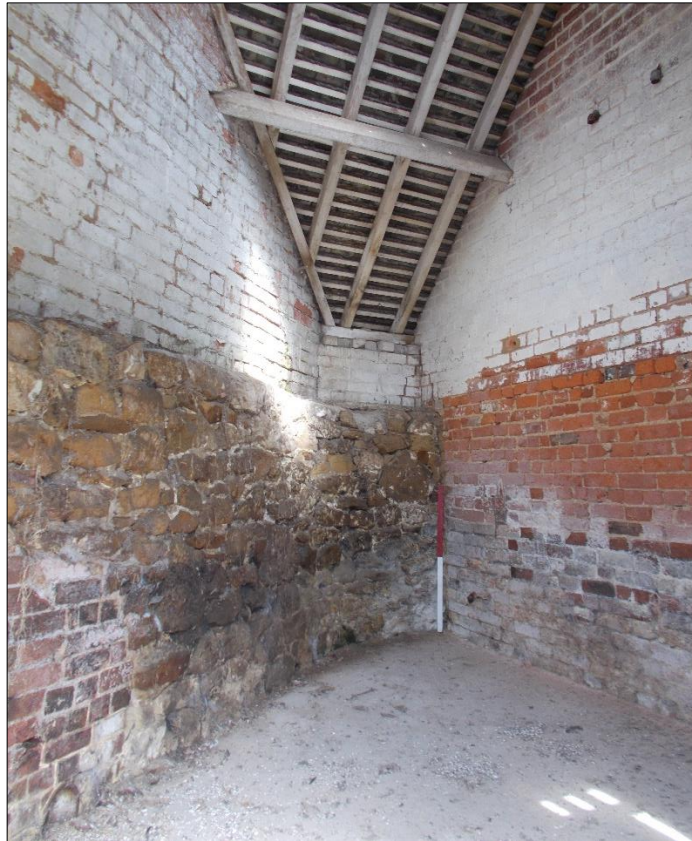
Fig 85: The odd-shaped room at the southern end of the cattle stall range, looking north. 2m scale rod.
