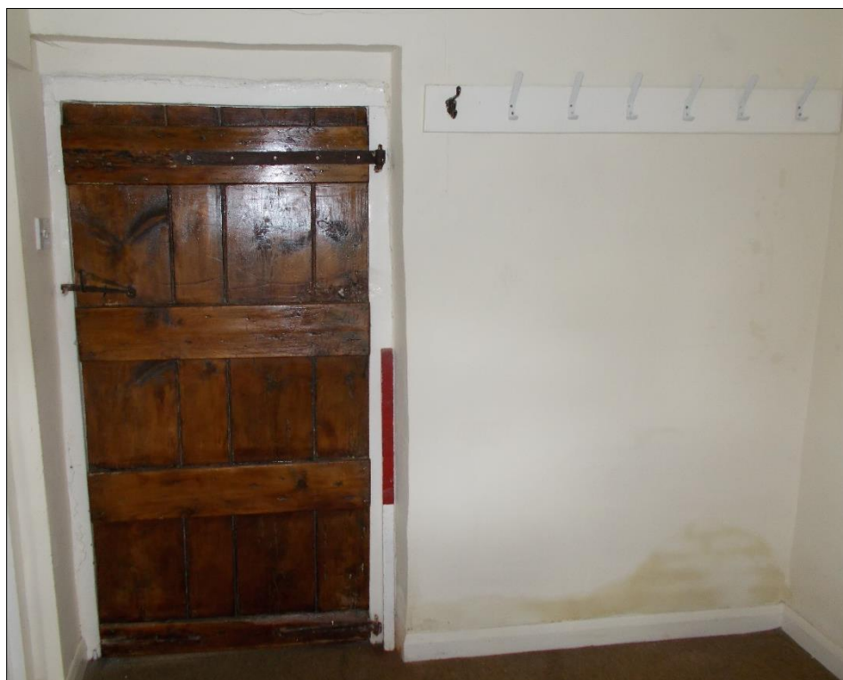
Fig 37: Room G10, looking south-east to door into room G6. 1m scale rod.
