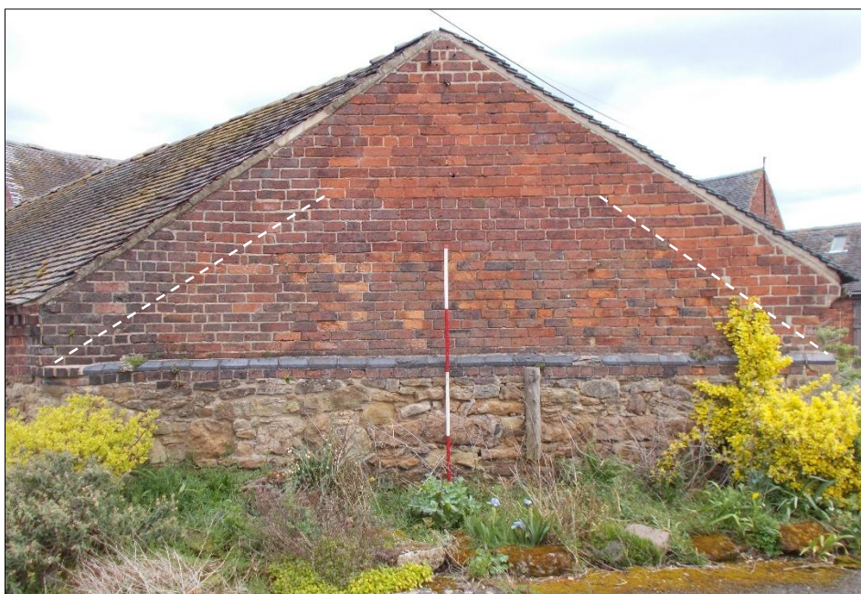
Fig 82: The south gable of the cattle stall range, looking north-east. The white dashed lines indicate the earlier roof profile. 2m scale rod.
