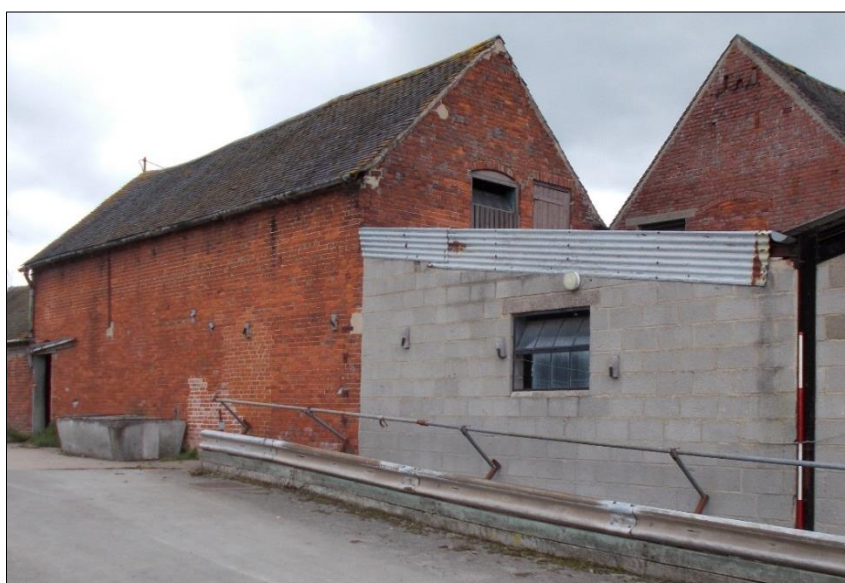
Fig 93: The north gable wall of the two-storey dairy range, looking south-west. 2m scale rod.
