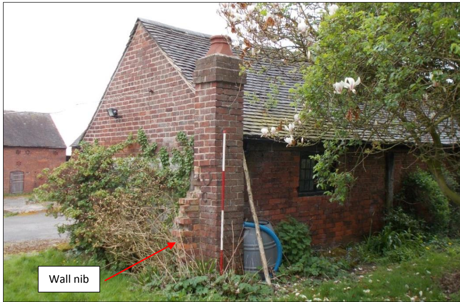
Fig 58: The chimney stack and wall-nib of the lost structure located at the north-west end of the loose box and cart shed range, looking east. 2m scale rod.
