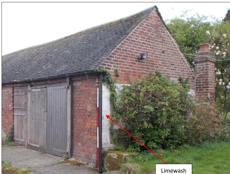
Fig 59: The north-west elevation of the former interior face of the lost structure, looking south. 2m scale rod.
