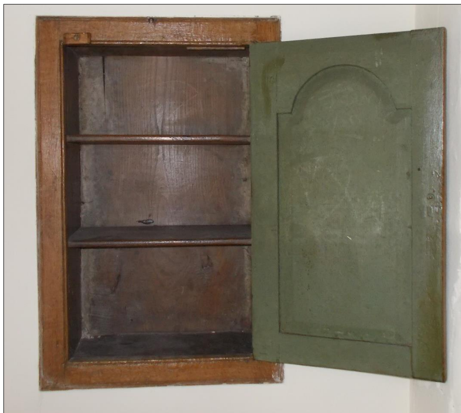
Fig 18: The spice cupboard set with the back wall of the inglenook in G4.
