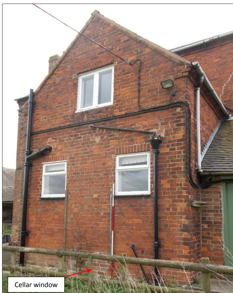
Fig 11: The north-west gable of the rear wing, looking south-east. 2m scale rod.
