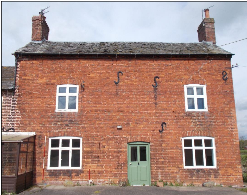
Fig 6: The two and a half storey phase one portion of the main farmhouse, looking north-west. 1m and 2m scale rods. The 1m rod rests in a 300mm-deep French drain cut through the surrounding concrete apron.
