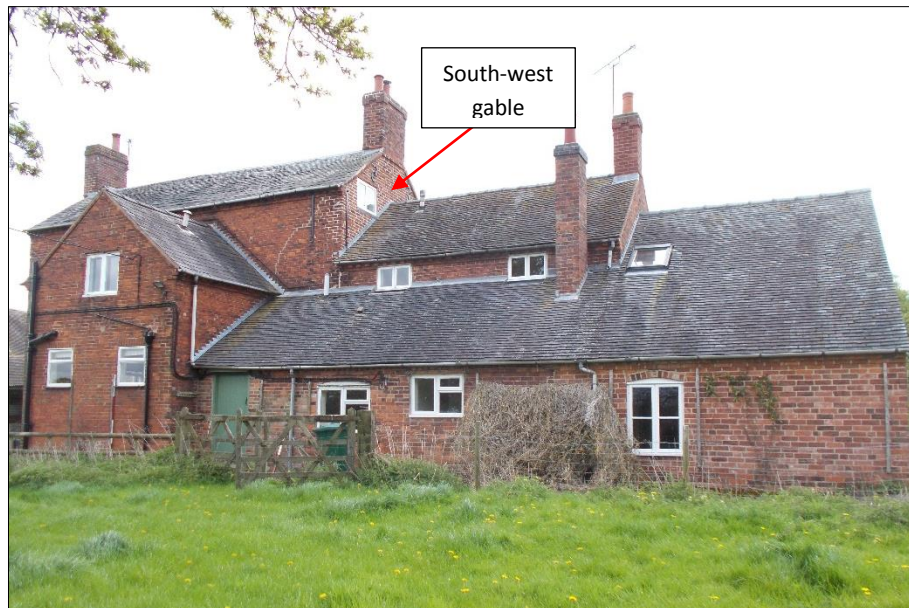
Fig 13: The farmhouse, looking south-east showing early south-west gable above later work. 2m scale rod.
