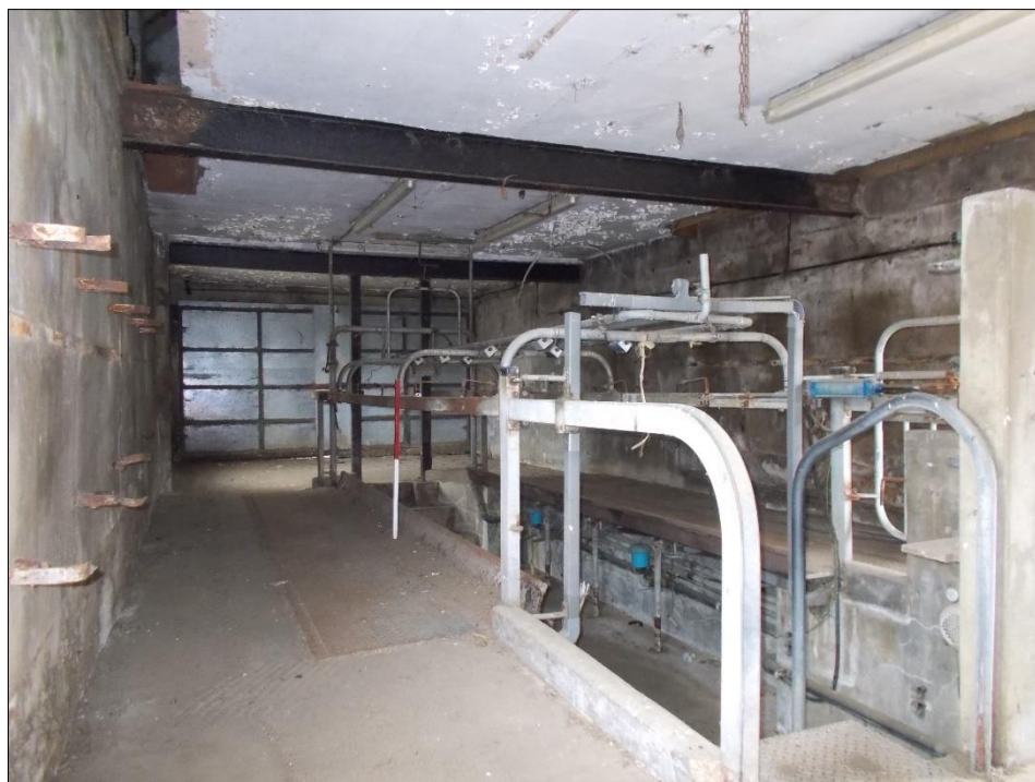
Fig 95: The ground-floor of the two-storey dairy range showing the milking parlour, looking north-east. 1m scale rod.
