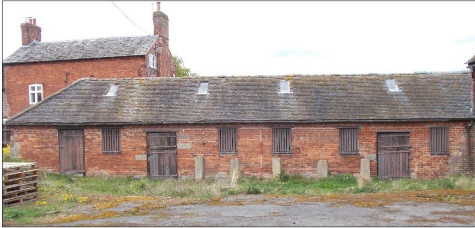
Fig 80: The cattle stall range, the stockyard elevation, looking north-west. 2m scale rod.
