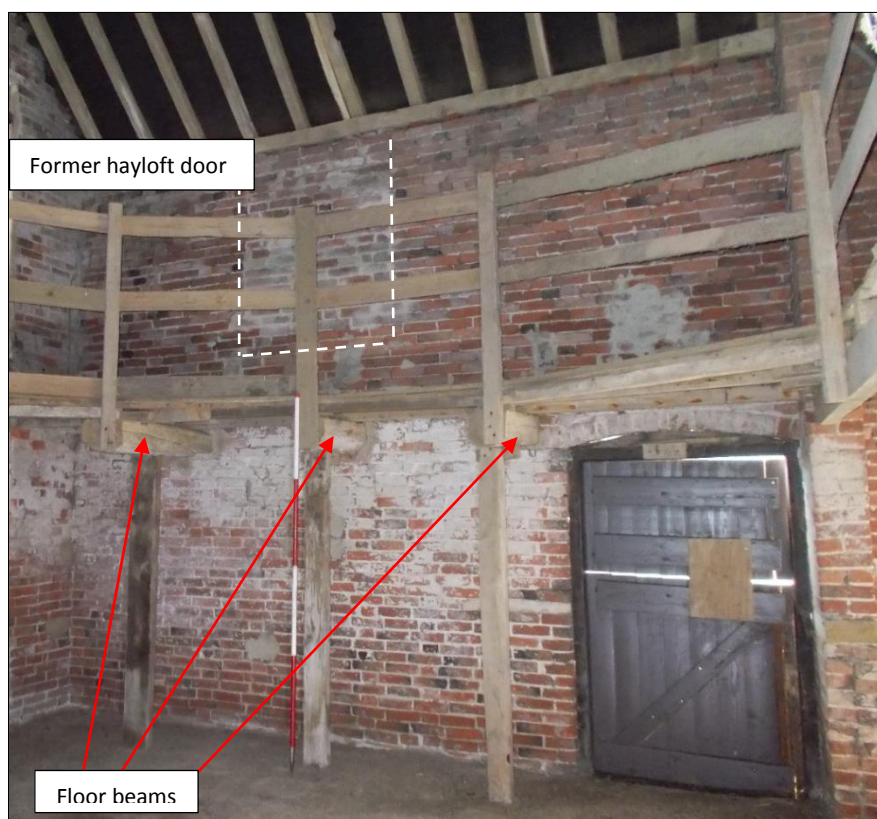
Fig 67: The southernmost bay of the south-west elevation, looking south. 2m scale rod.
