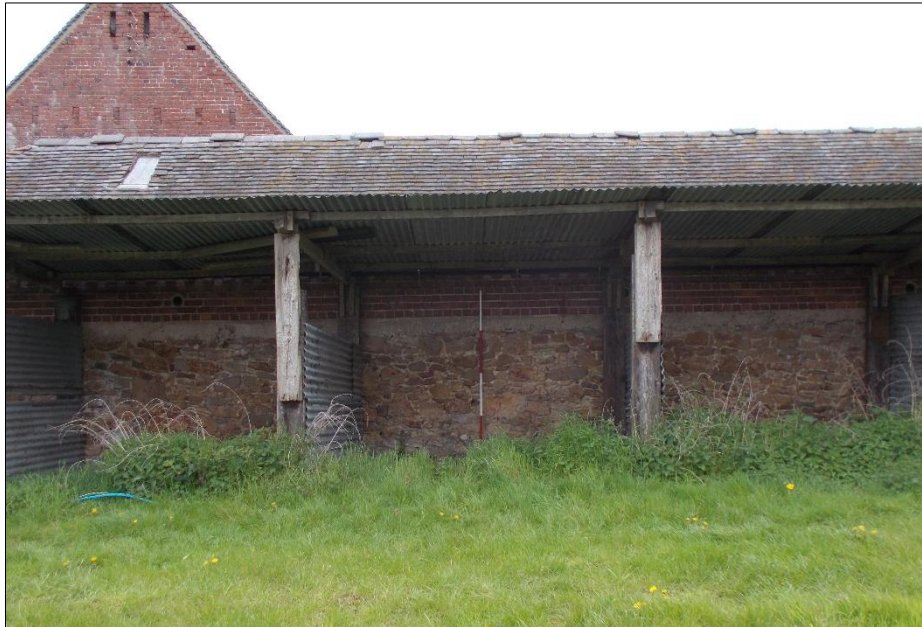
Fig 83: The north-west elevation showing the stone and brick construction. 2m scale rod.
