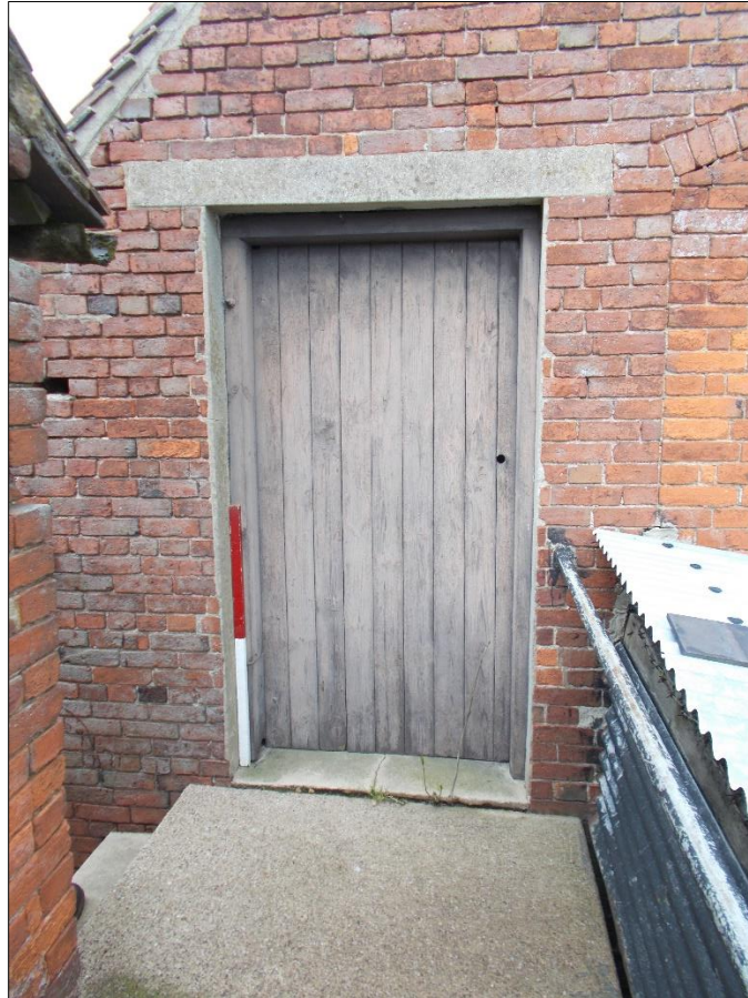
Fig 77: The external stairs and landing affording access to the first-floors of the store barn and the dairy barn ranges, looking north-west. 1m scale rod.
