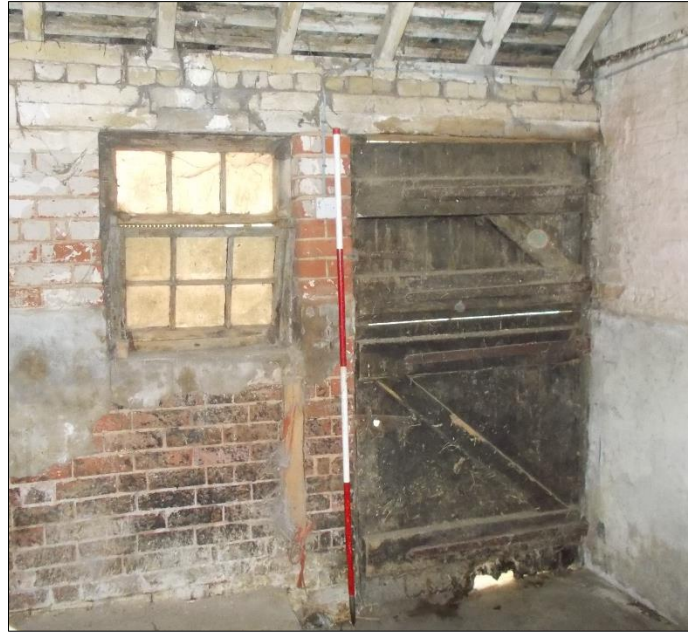
Fig 87: The north wall of the cattle stall range, looking north-east. 2m scale rod.
