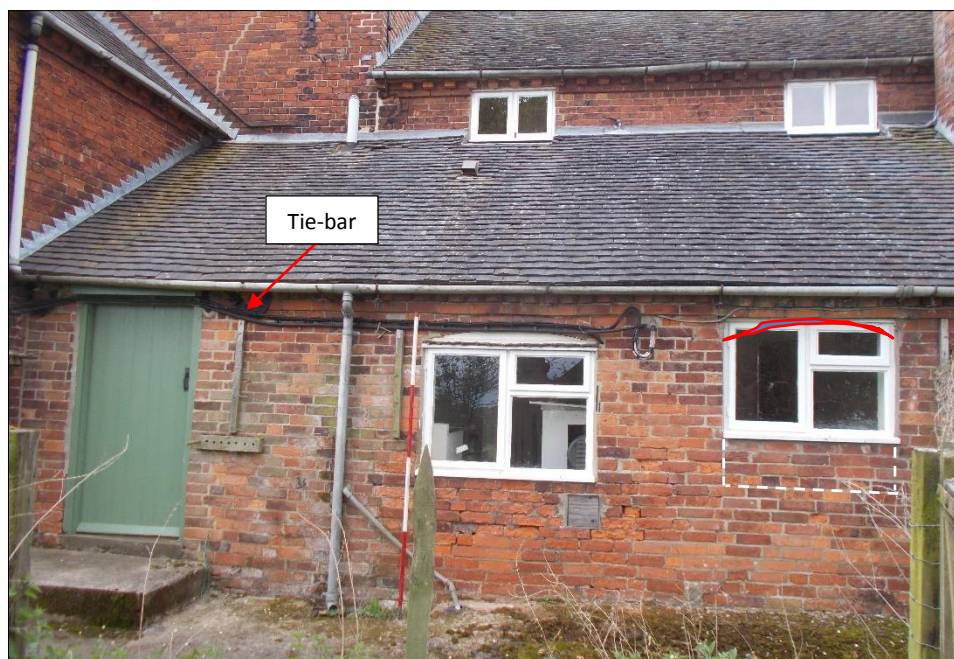
Fig 35: The phase three lean-to extension, looking east. The white dashed lines show reduced window to the right, red line former segmental arch above same opening. 2m scale rod.
