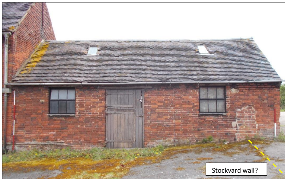
Fig 99: The southwest elevation of the single-storey dairy range, looking east. 1m and 2m scale rods.
