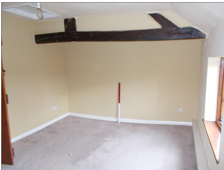
Fig 33: Room F6, looking north-east showing lower part of roof truss. 1m scale rod.
