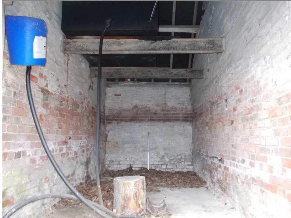
Fig 50: Room G14, looking south-west showing oil tank on RSJ's. 1m scale rod.
