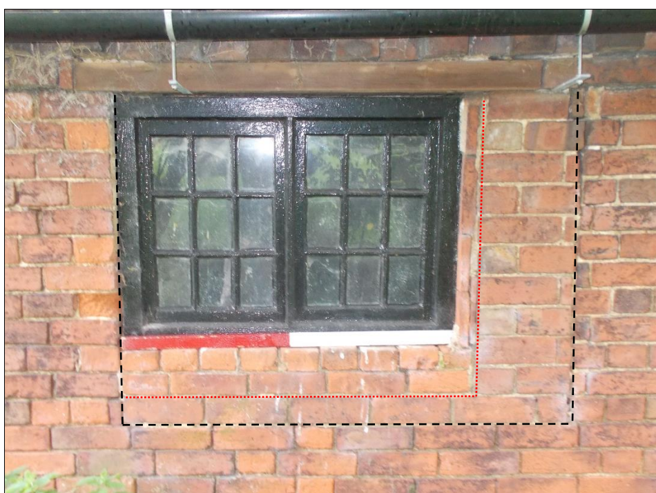
Fig 45: Room G12, the re-set window showing two previous settings; the first outlined in black dashed lines, the second in red dotted lines. Looking north-east. 1m scale rod.
