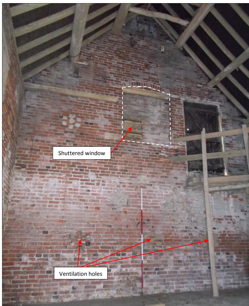
Fig 76: The south-east gable wall, interior elevation, looking south-east. Former hayloft door outlined with white dashed lines. 2m scale rod.
