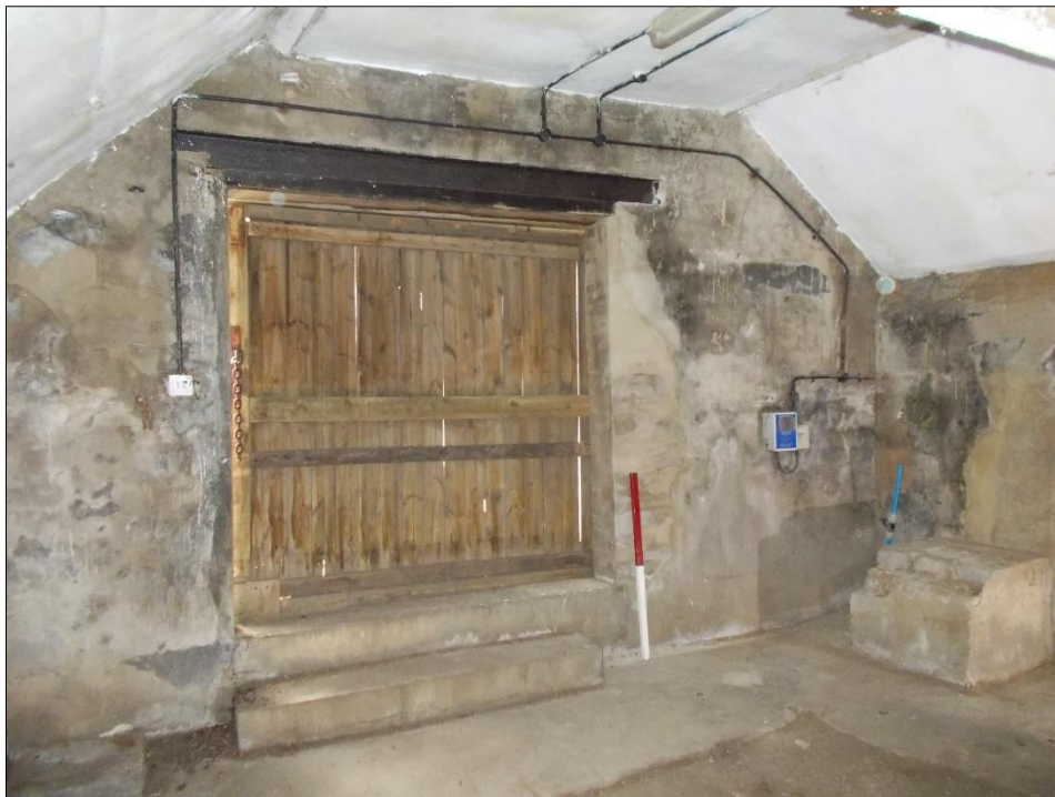
Fig 102: The south gable wall with sliding door, of the single-storey dairy range, looking west. 1m scale rod.
