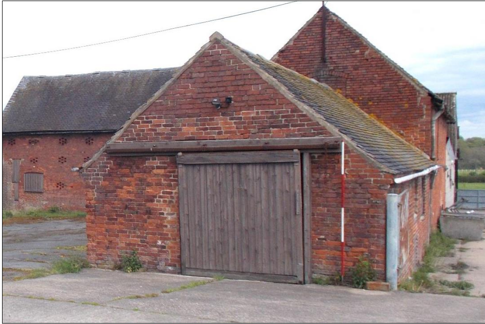
Fig 100: The south gable wall of the single-storey dairy range, looking north. 2m scale rod.
