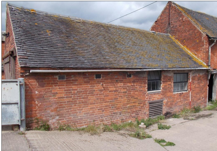
Fig 101: The south-east elevation of the single-storey dairy range, looking north. 2m scale rod.
