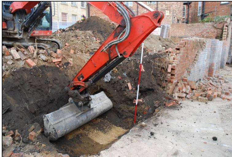
Fig 3: A machined test pit failed to expose natural ironstone geology even 300mm below the Vulcan Works (adjacent Block A, bay 9) concrete floor, c2.5m below the modern (Angel Street) ground surface; scale 2m
