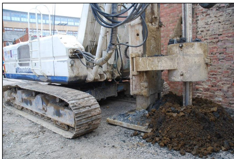
Fig 7: CFA piling in progress in angle between retained portion of Weights and Measures building and Vulcan Works inter-war shed 1. View looking south-east.
