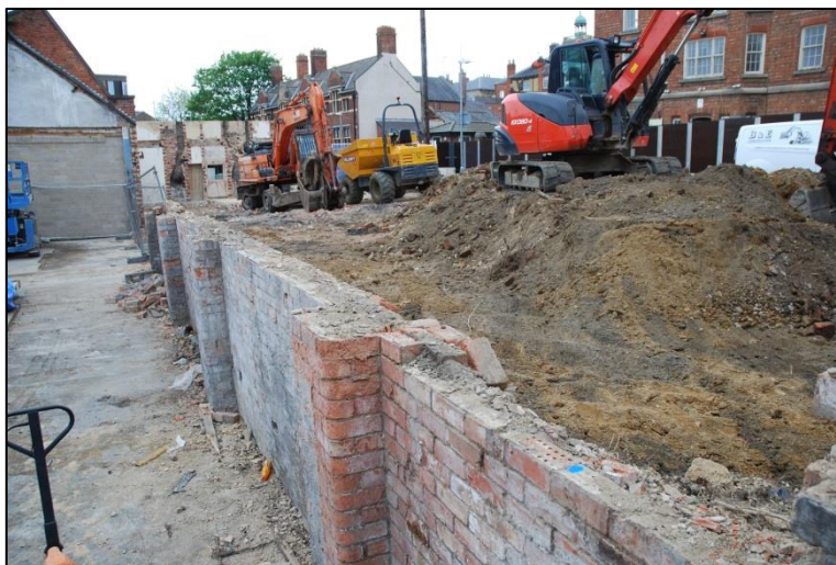
Fig 2: Reducing the modern (Angel Street) level; at left the Vulcan Works floor level (Block A, bays 5-11). View looking west from Block A, bay 5.
