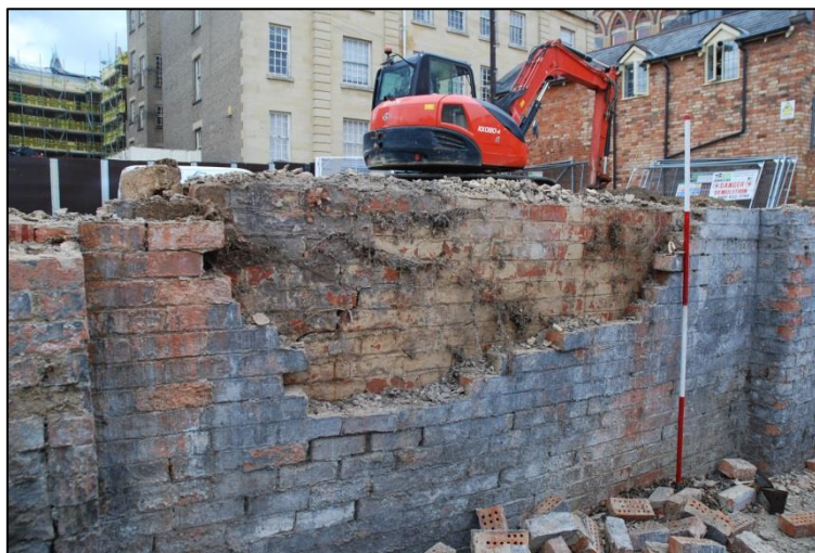
Fig 4: The 4 ½ inch-thin Vulcan works (Block A, bay 9) north wall-skin, built up against the outer face of earlier foundry boundary retaining wall, still with its pale lime-wash. View looking north; scale 2m
