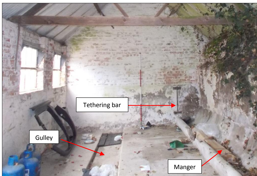
Fig 18: The interior of the central room in the west range, looking west. 2m scale rod.
