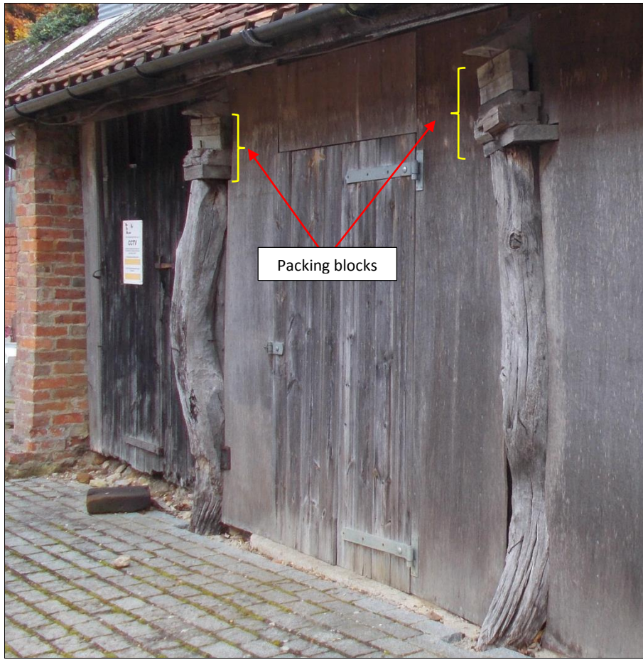
Fig 7: The re-set oak posts with timber packing to support the roof trusses.
