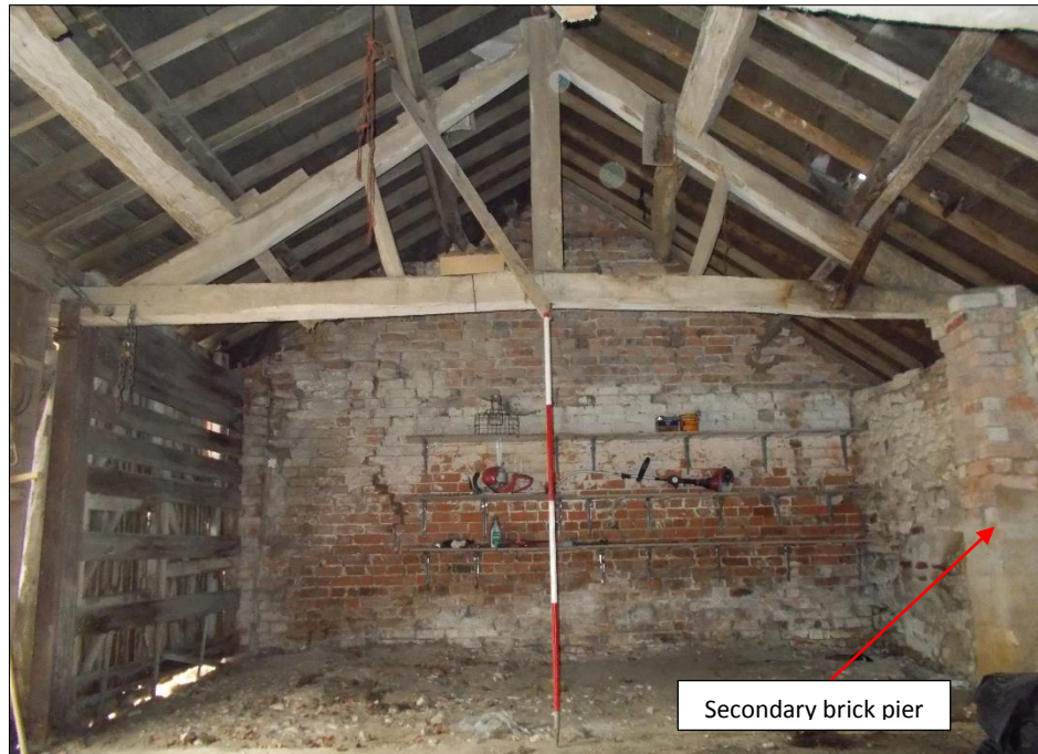
Fig 6: The east range three-bay hovel with western roof truss, looking west. 2m scale rod.
