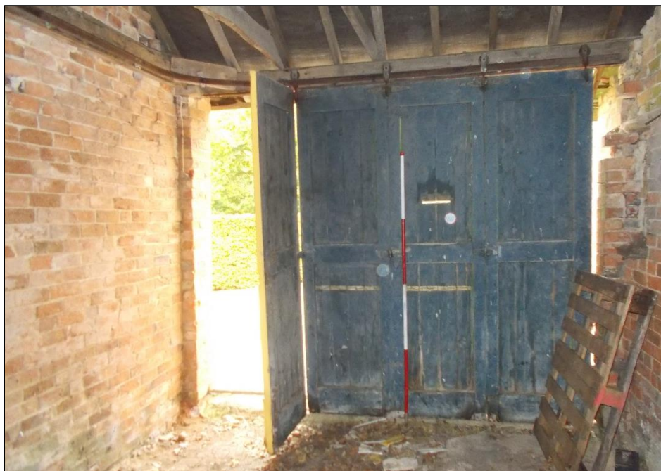
Fig 11: The eastern room of the east range, showing the inner face of the sliding door and hanging rail. 2m scale rod.
