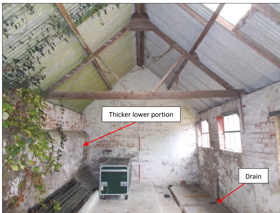
Fig 14: The interior of the central section of the east range, looking east. 2m scale rod.
