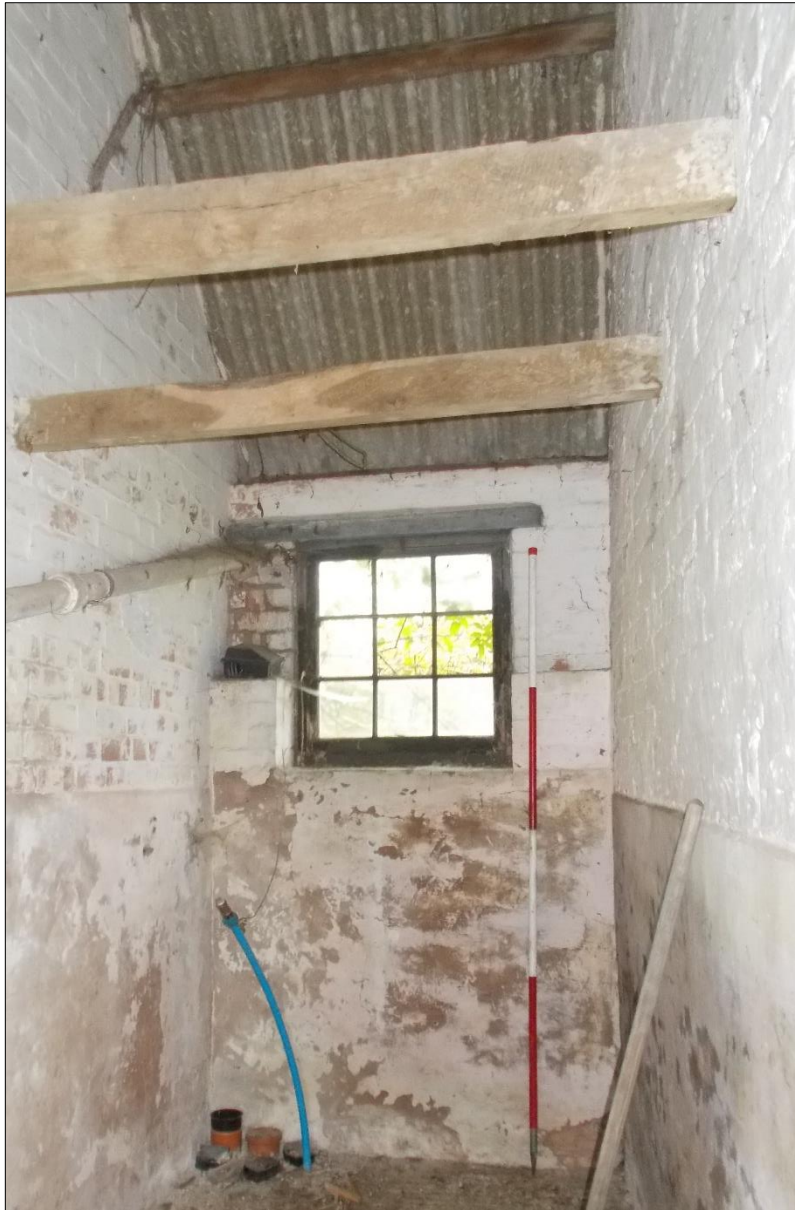
Fig 19: The eastern room of the west range, looking north. 2m scale rod.
