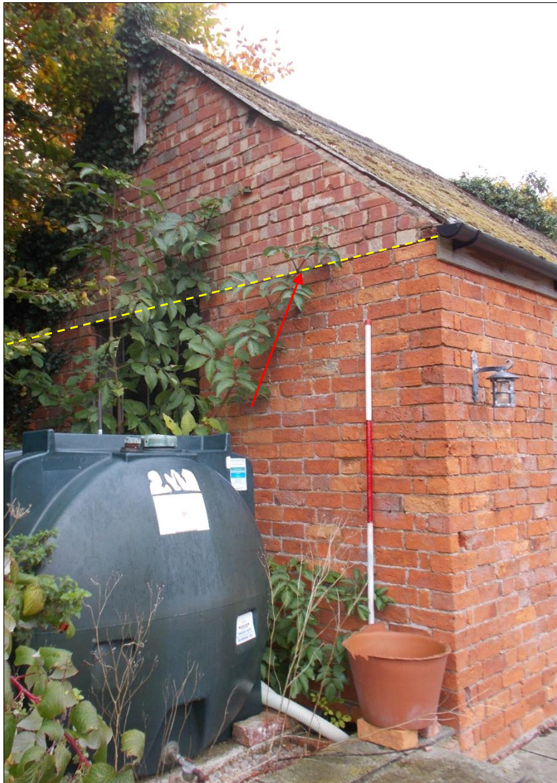
Fig 13: The west gable showing the upper re-built section (above yellow dashed line). 2m scale rod.
